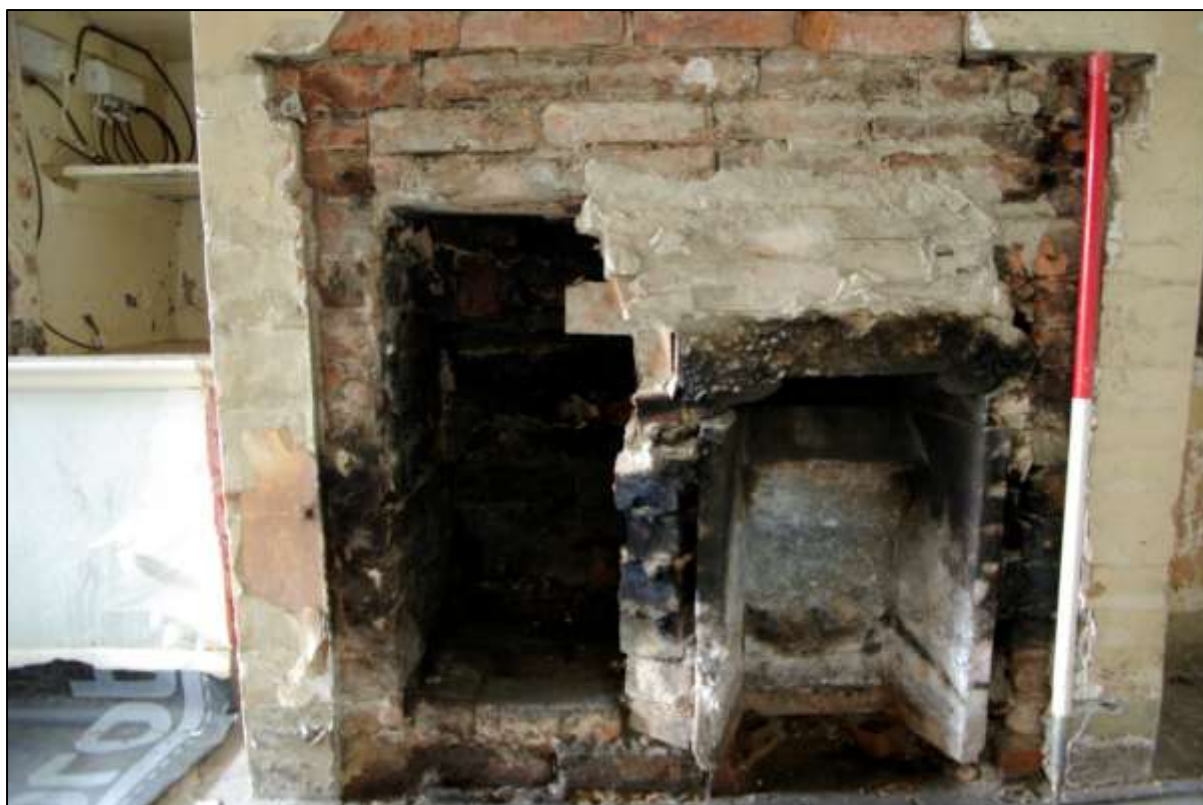
Figure 51. Outline of earlier fireplace and partially blocked opening showing position of earlier range stove, with modern fire-bricks to right hand side.
