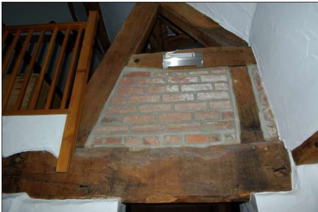
Figure 48. Interrupted tie-beam supported by short post, which is tenoned into the transverse axial floor beam. Looking south.
