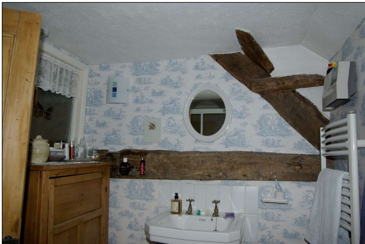
Figure 42. Principal rafter roof truss in gable end wall of modern bathroom, looking west.
