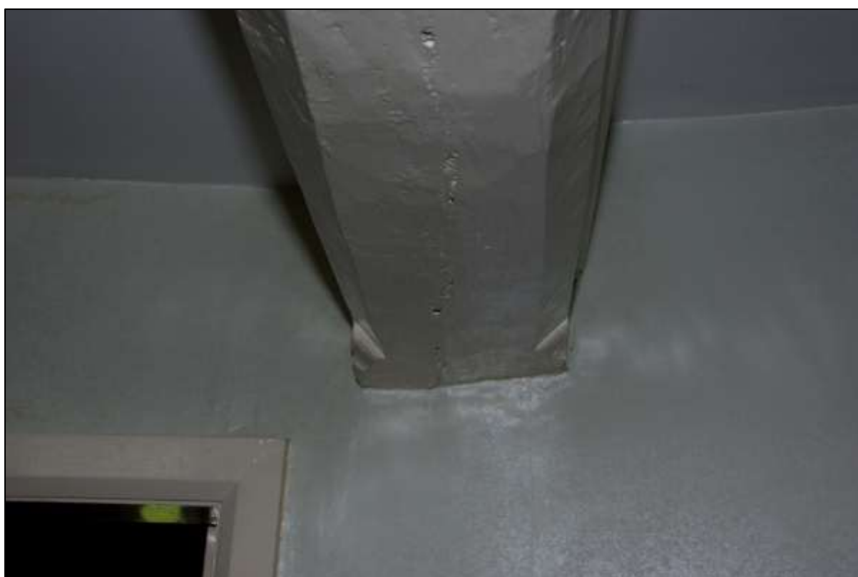
Figure 35. Chamfered axial beam over former living kitchen, with scroll stops. Looking north.
