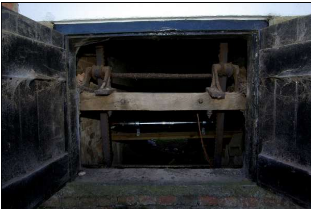
Figure 30. Sluice-gate mechanism in wheel-house. Looking east.
