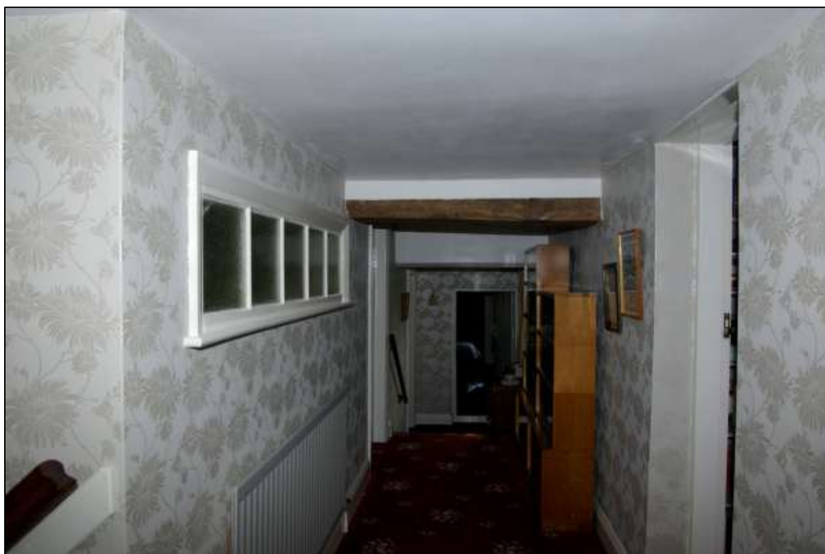
Figure 37. First floor landing, 1930s stud partition wall to left hand side, looking south.
