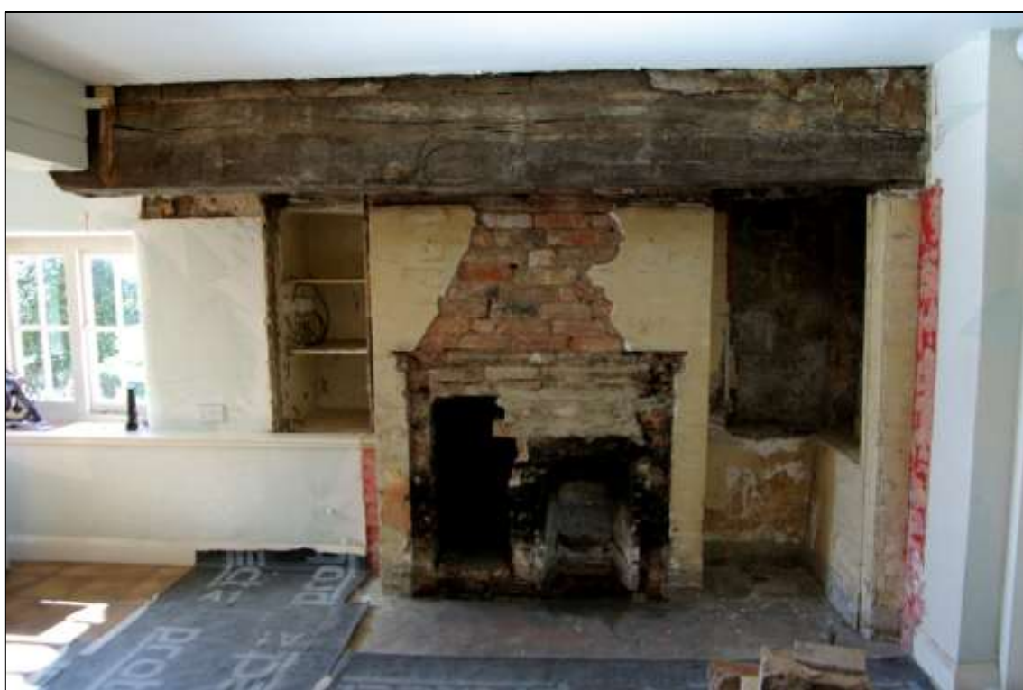
Figure 50. Timber bresummer and 19th-century brick stack exposed following removal of modern brickwork
