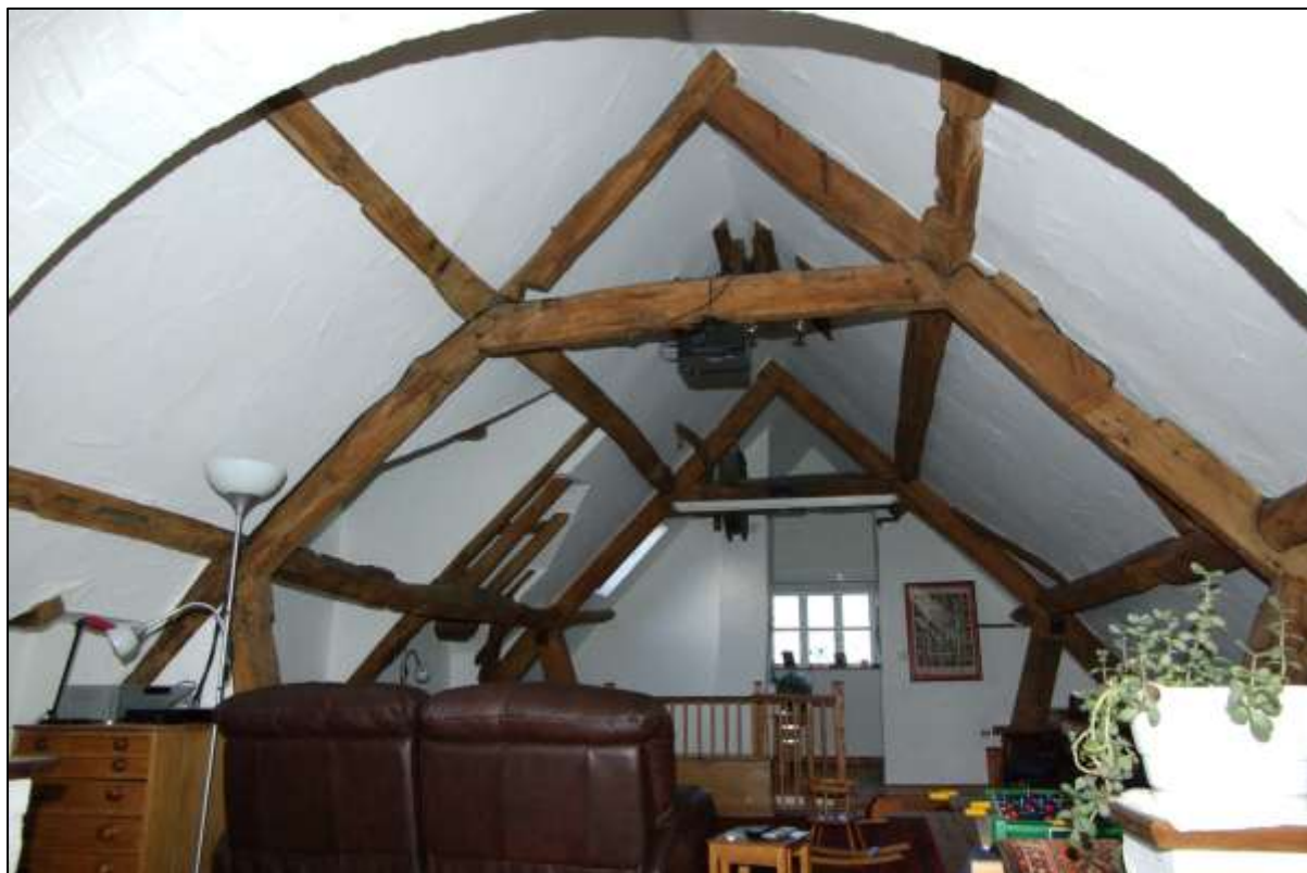
Figure 44. Principal-rafter room trusses at second floor level, with interrupted tie-beam. Looking north.
