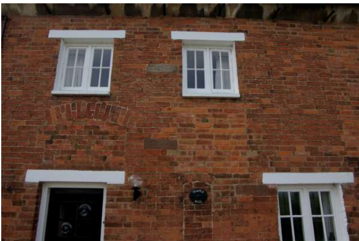
Figure 22. Front elevation with blocked doorway opening at first floor level, looking west.
