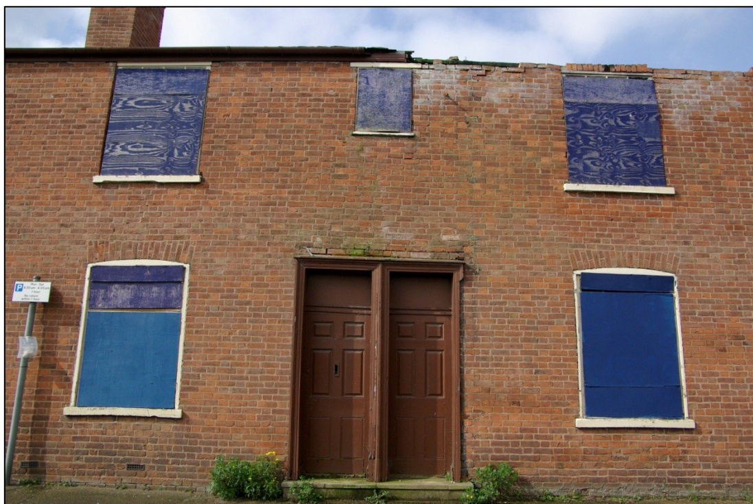
Figure 29. Bath Lane cottages, pair of moulded timber doorcases, with boarded fanlights and panelled doors. Looking west.
