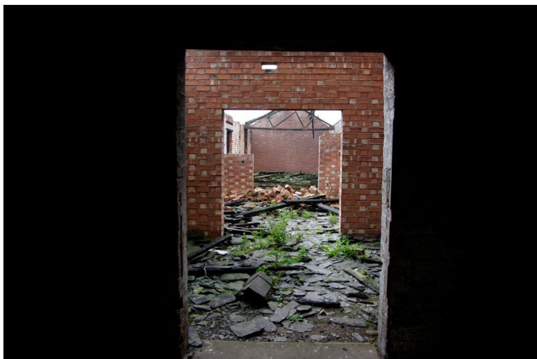
Figure 40. Bath Lane cottages, first floor, seen from Bath Lane Mill interior. Looking south.
