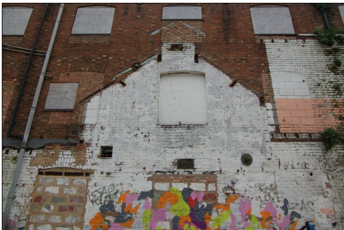
Figure 34. Detail of above, with blocked window openings and scars of removed structures. Looking east.
