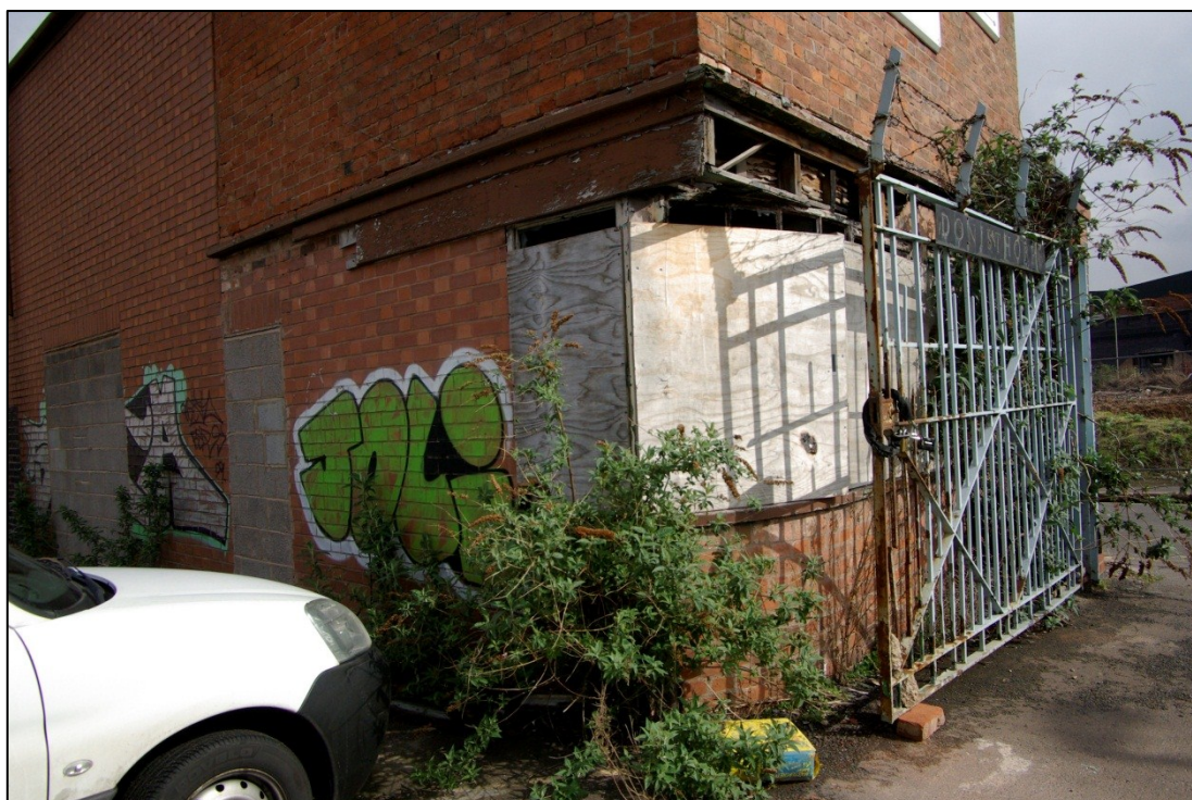
Figure 28. Bath Lane Cottages, timber windows and fascia boards to former offices, looking east.
