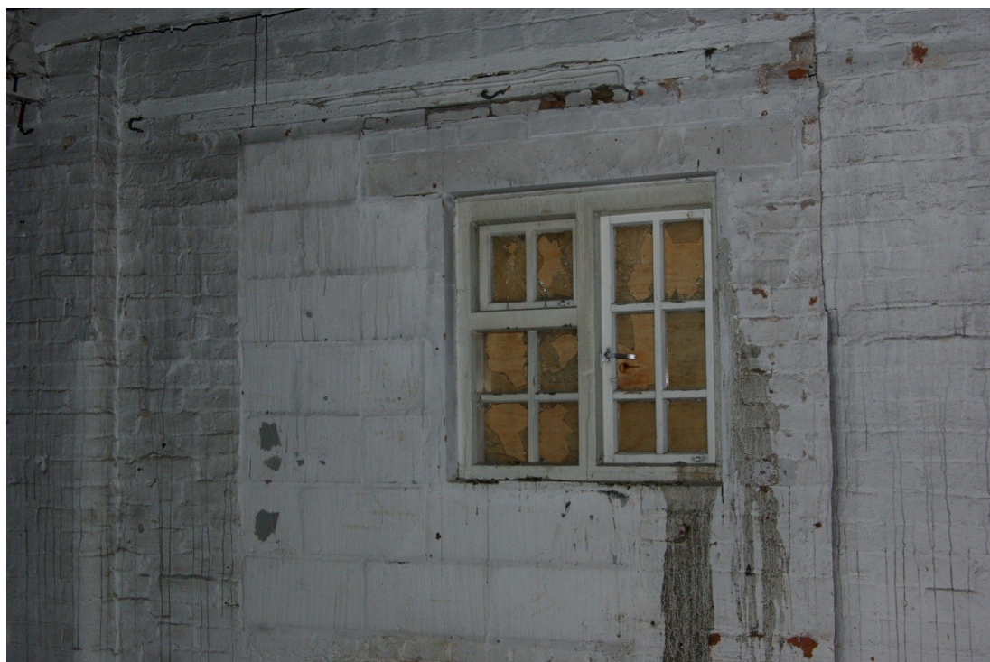
Figure 39. Bath Lane Mill, first floor. Small timber multi-paned window frame inserted within larger, blocked original window opening. Looking west.
