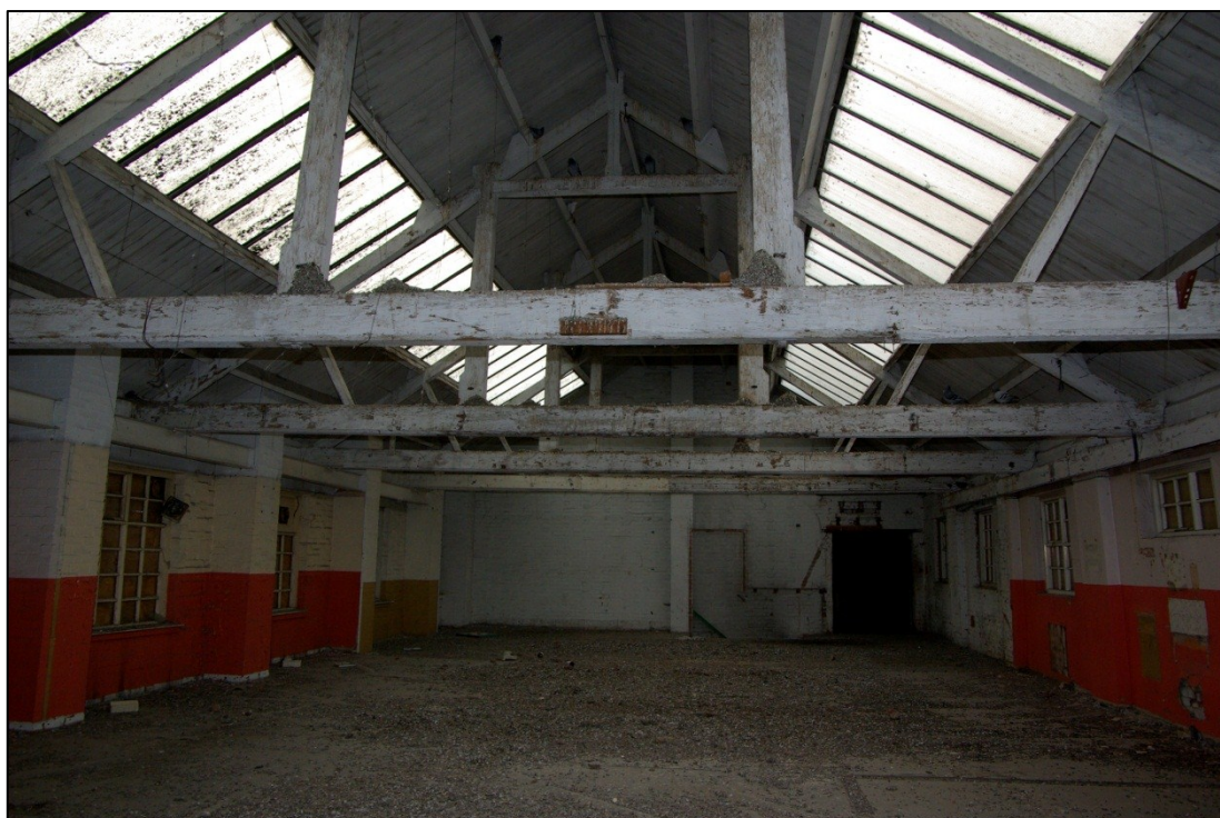
Figure 41. Bath Lane Mill, second floor. Timber queen-strut roof trusses, with upper king-posts supported by a strainer beam. Looking south.
