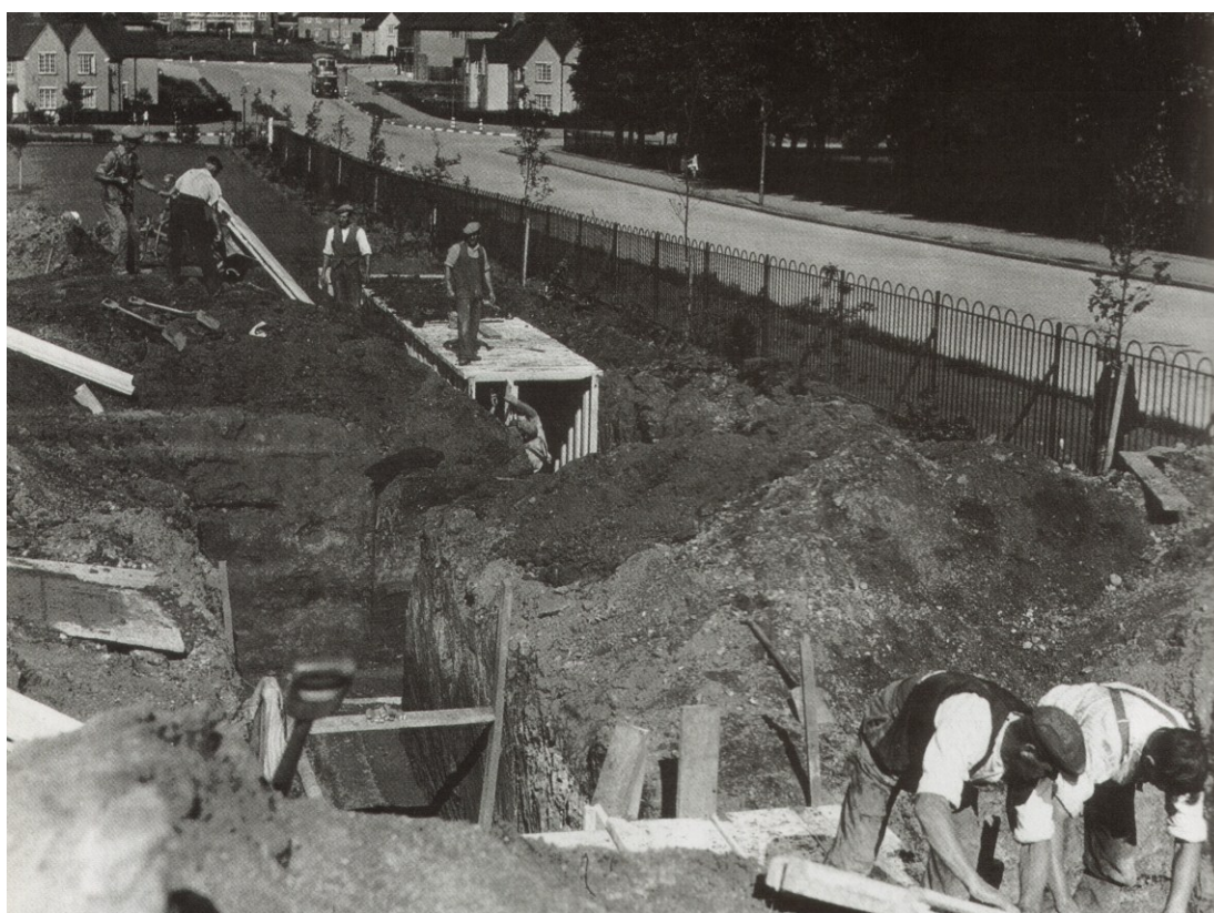
Figure 24 Construction of an air-raid shelter Fullhurst Community College (formerly Newarke Girls School) (Record office for Leicestershire, Leicester and Rutland)
