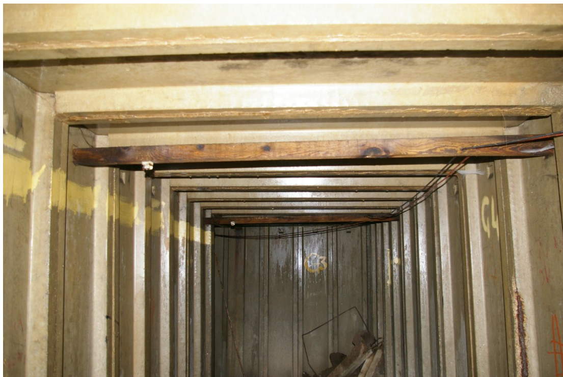
Figure 22 Lighting system in-situ, Tunnel G Looking north east. Note wooden cross members held in pre-cast slots
