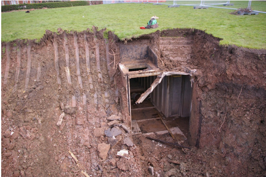
Figure 14 Roof structure and vent Note original turf line running across the section at ceiling height
