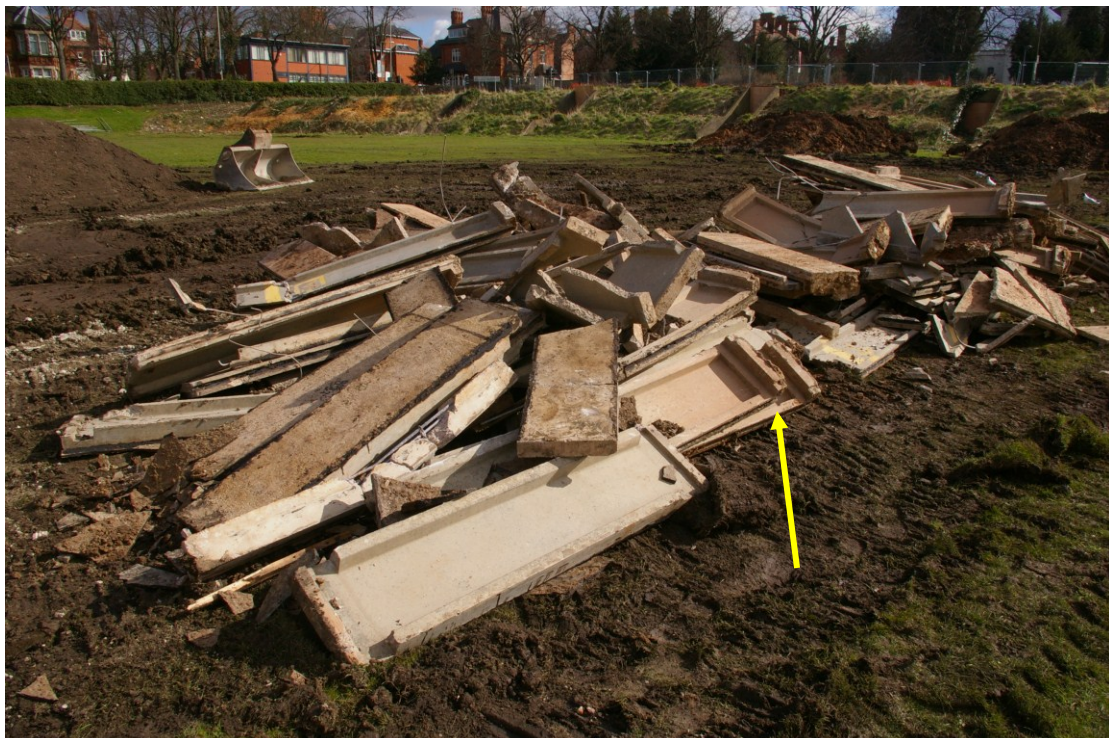
Figure 15 Removed roof and wall panels Roof panel in foreground. Arrow the shows foot of a wall panel
