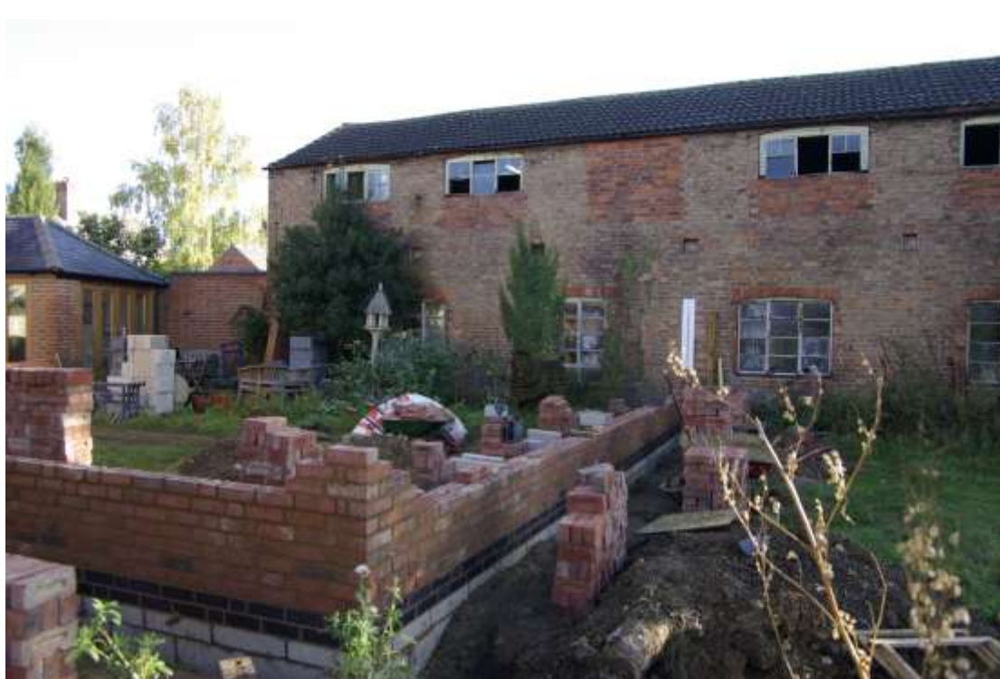
Figure 16 Northern end of Building 2 belonging to 22 High Street Photo taken in October 2013 during construction of new boundary wall
