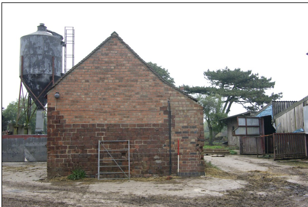
Figure 16. South-west facing gable end, with lower courses of 'jumb' bricks and early 20th century rebuild above and extension to the western side.
