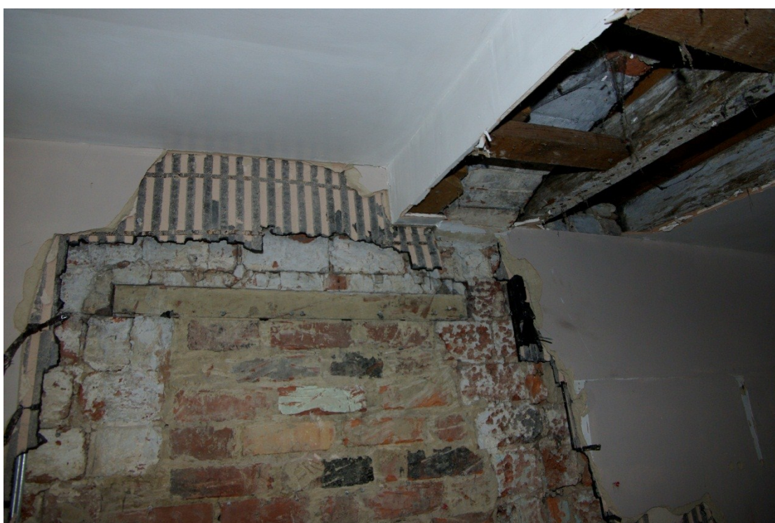
Figure 40. Blocked doorway with timber lintel and brick relieving arch over, looking south-west.
