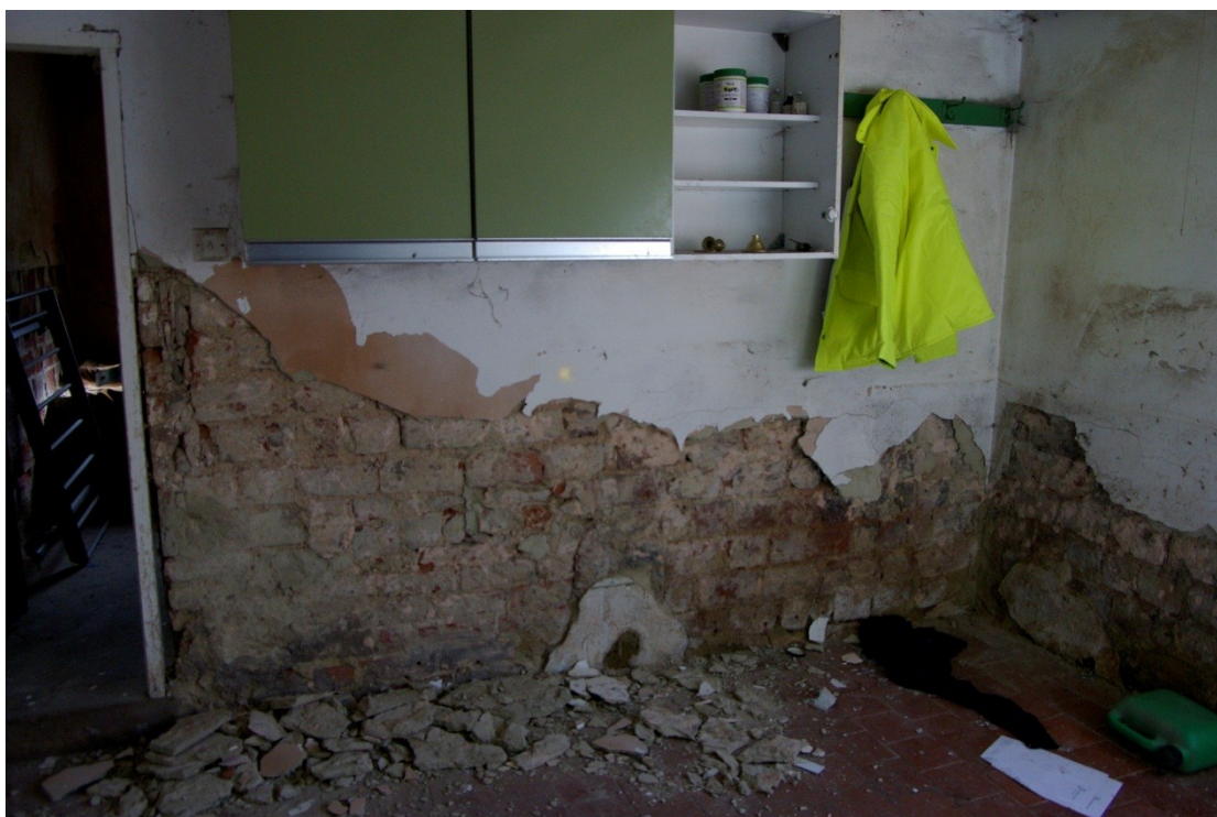
Figure 42. Jumb bricks to internal and external wall of utility room/possible former dairy. Looking south.
