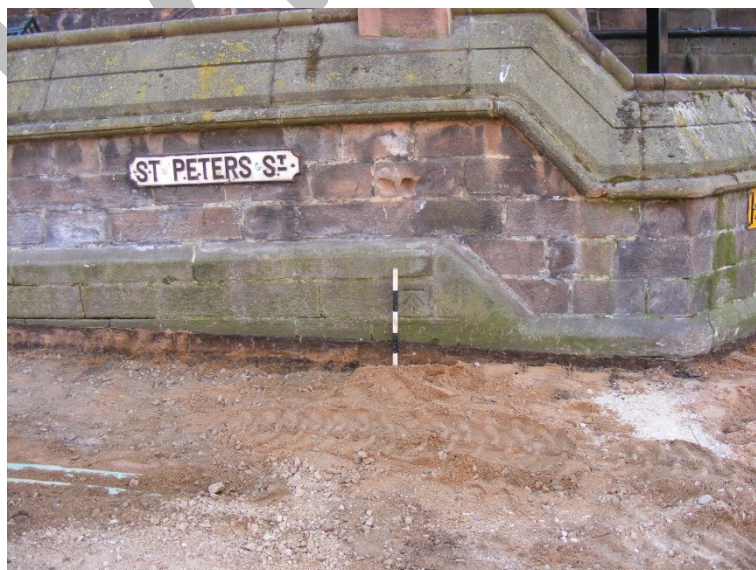
Figure 5: Bench-mark on the east end of the church, showing relation to formation level
