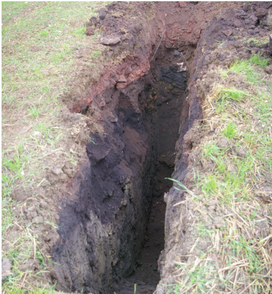
Plate 8: Geo-technical pit excavated in northern part of field, showing deep quarry backfill, looking west
