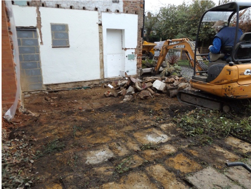
Figure 4. Machine removing overburden to a depth of c. 0.4 m revealing made ground to the south of the existing building.
