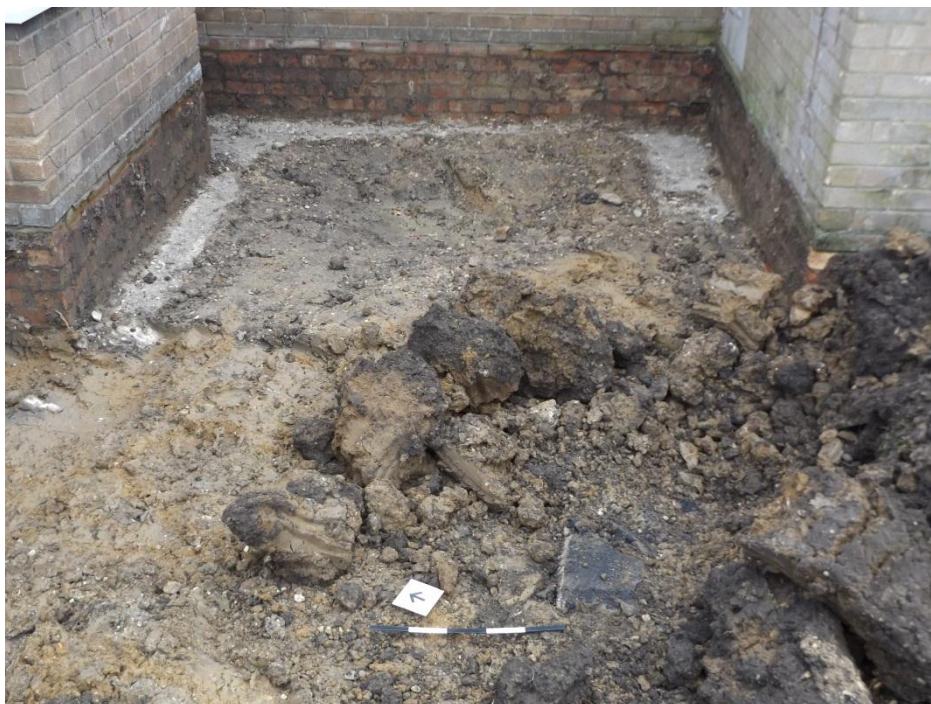
Figure 6. Soakaway pipe cover (black asphalt slab in foreground) and made ground in natural substratum within extension footprint.
