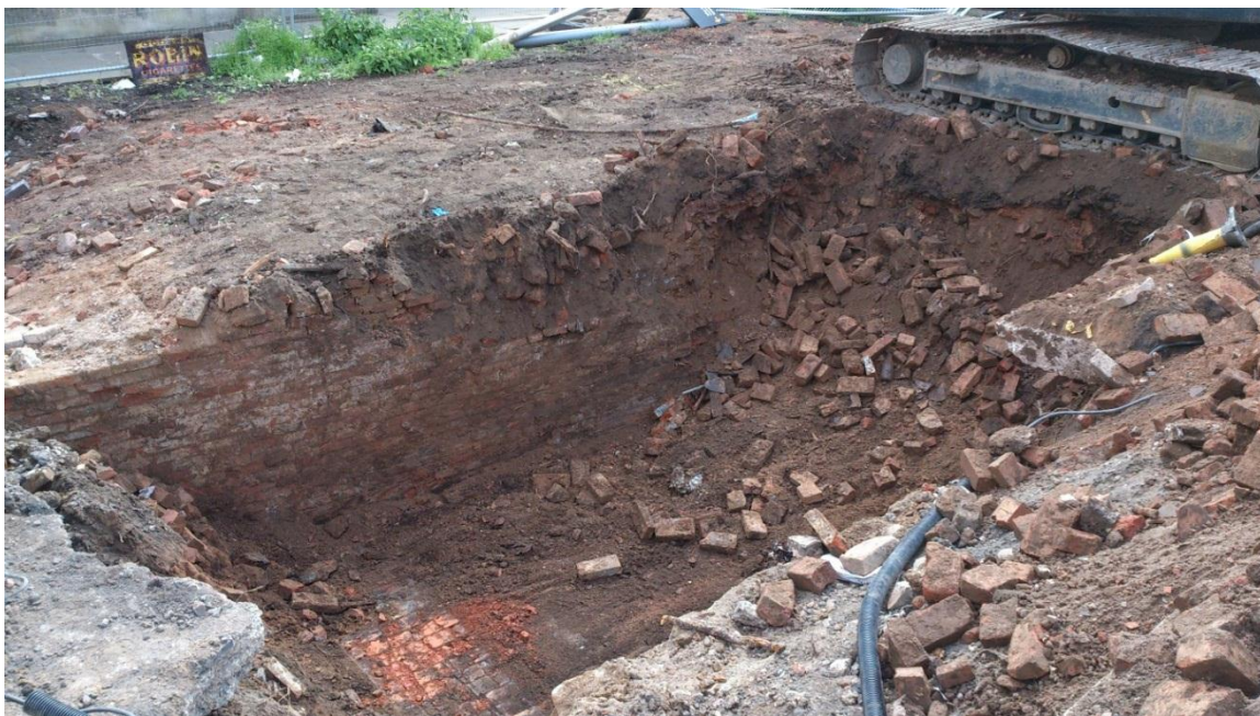
Figure 37 Tree-pit TP19 during excavation. Cellar wall at south, and cellar floor being exposed. Looking south-west.
