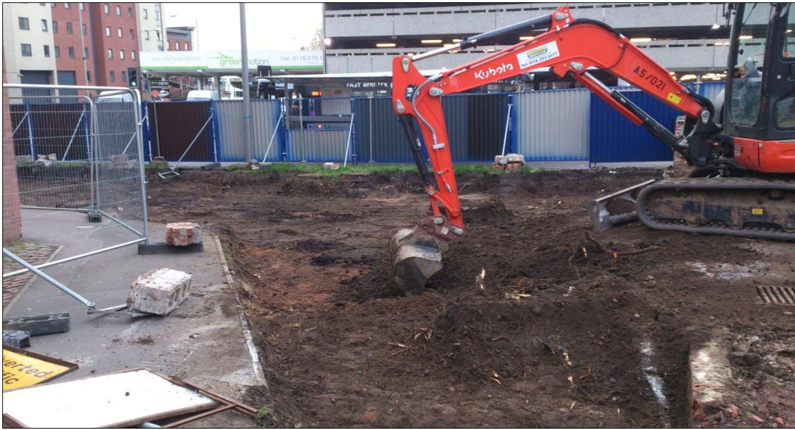
Figure 8 Reduced level works, in the area west of Carey's Close, looking west.
