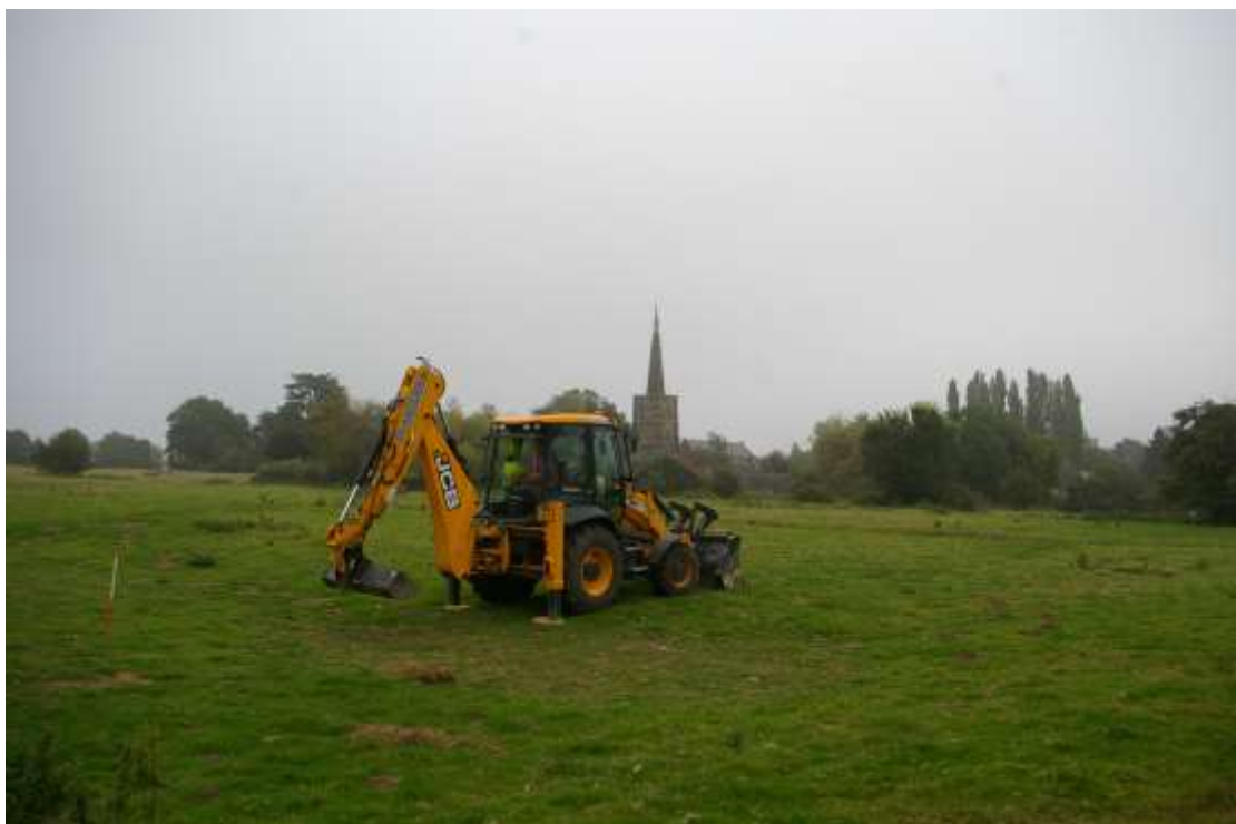
Figure 8 Trench 1 before excavation Trench 1 to be dug between ranging poles. JCB is on top of low earthwork
