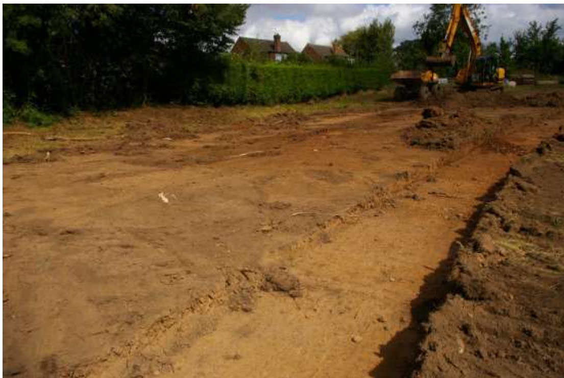
Figure 10 Reducing site down to formation level adjacent to Measham Road Looking north
