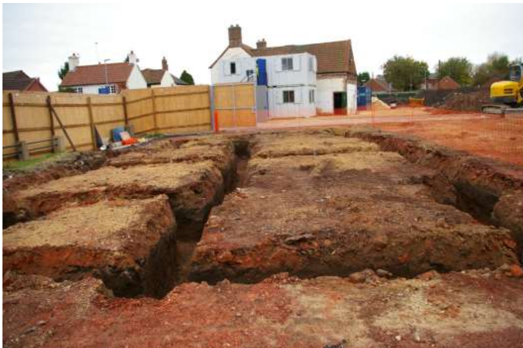
Figure 7: General view of foundation trenches looking south towards the pub and showing make-up layers.
