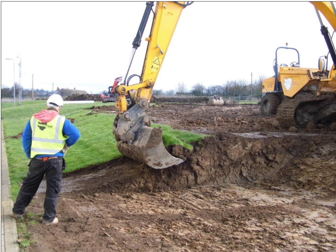
Figure 4: Machine removing turf/topsoil to reveal made ground immediately south-west of existing buildings (Phase 1).
