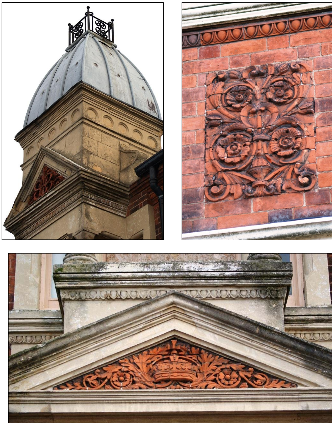
Fig. 26. Detailing on west facing elevation, west range. Top left, the tower, looking north east; top right, an example of the terracotta relief looking south east; bottom, the lower pediment crown design, looking east.
