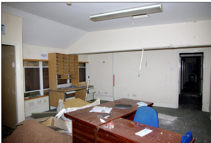
Figure 34. Office space in the low extension, looking north east, with 1m scale
