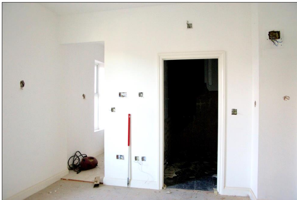
Figure 23. A modernised first floor bedroom with ensuite, looking southeast with 1m scale
