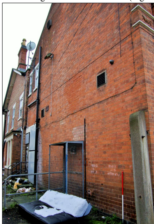
Figure 28. North facing elevation of west range looking south east with 1m scale.
