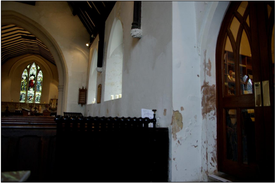
Figure 22. South wall of nave, with area of damage caused by damp. Looking south-east.
