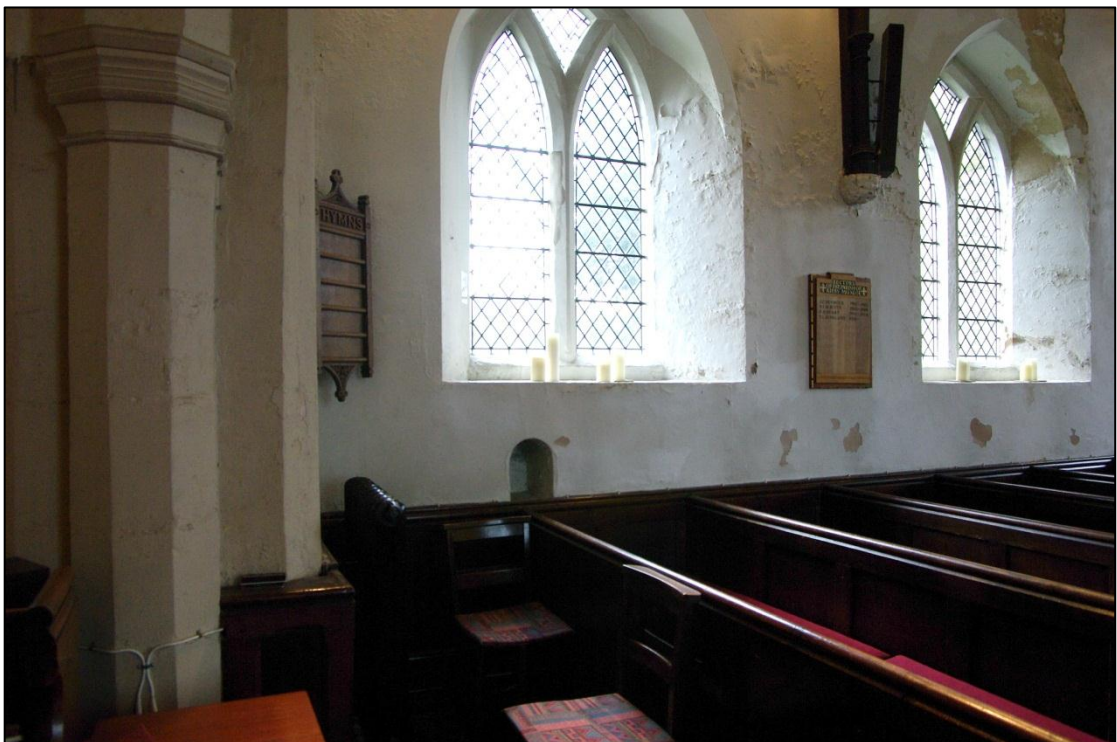
Figure 23. South wall of nave and piscina, showing further signs of damage to plaster. Looking south
