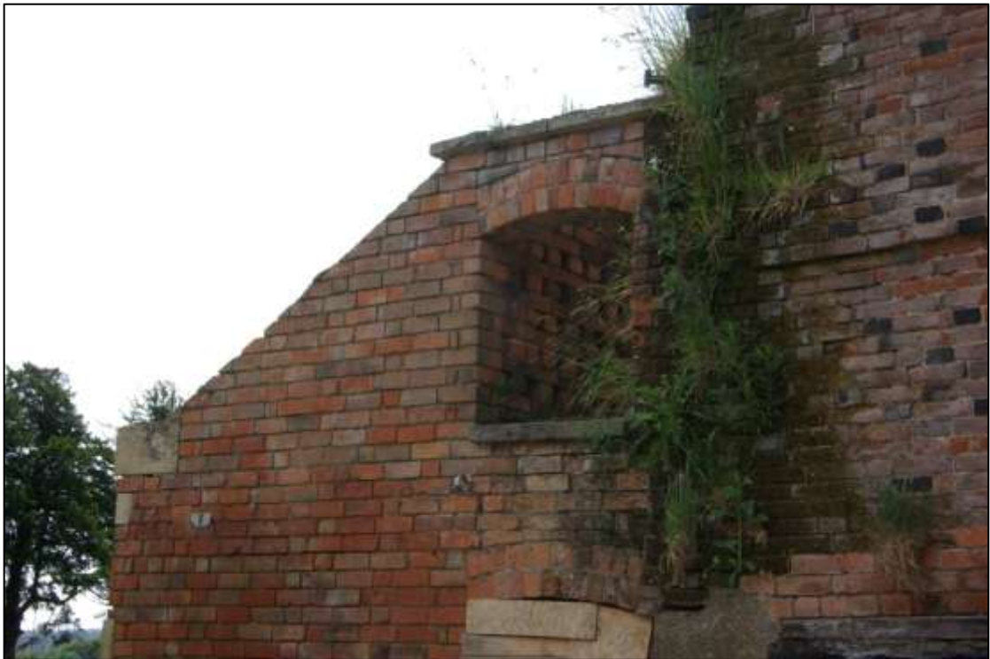
Figure 18. Pigeon holes into nesting boxes, formerly located within roof space. Looking south.
