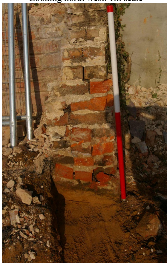
Figure 26 Section across north wall Base of metal fencing is resting on the internal ground floor level. Looking west. 1m scale
