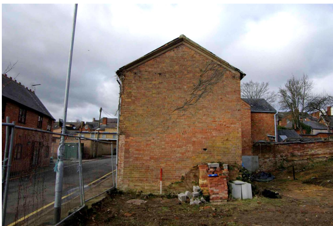
Figure 11 East facing elevation Looking west. 1m scale. Note wall scar on south corner of the Coach House
