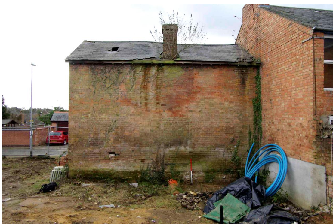
Figure 13 North-facing elevation Looking south. 1m ranging pole is just to right of blocked door
