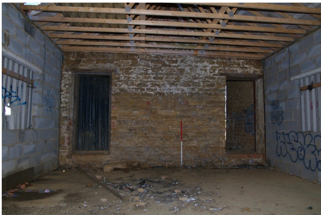
Figure 17 Old Barn, south facing elevation inside modern barn Looking north. 1m scale
