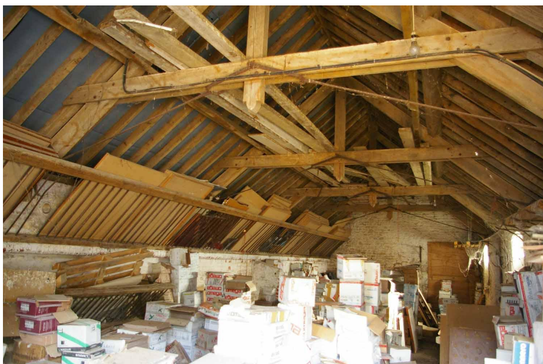
Figure 22 North range, western room (ground floor) Looking east north east. Note trough and stalls on left of picture
