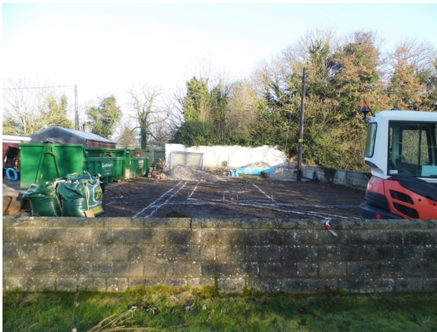
Figure 6: View of site prior to excavations. Former swimming pool in background. Looking north-west
