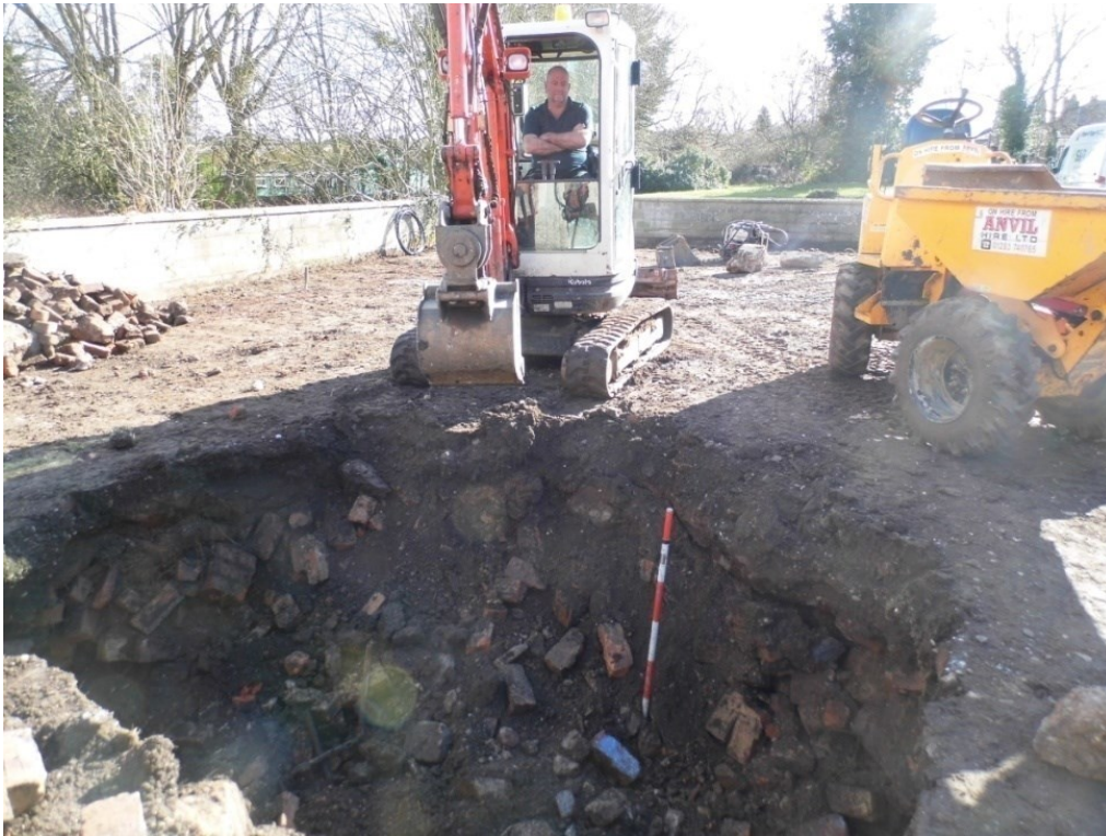
Figure 8: Excavation of water tank showing brick and concrete rubble. 1.10m scale. Looking south.
