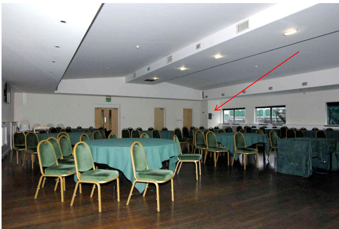
Figure 29 The Tiger Bar Looking north-east. Arrow points to chimney leading up from boiler room
