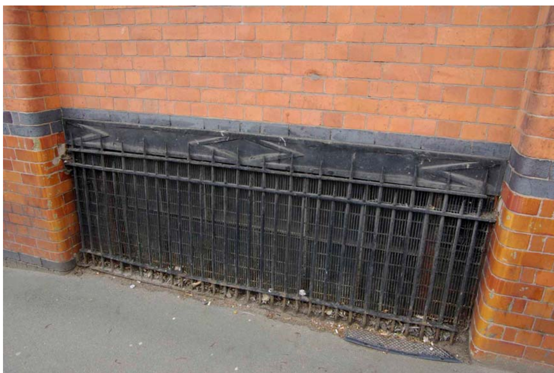
Figure 9 North-east facing elevation basement window detail Note glazed bricks either side of window
