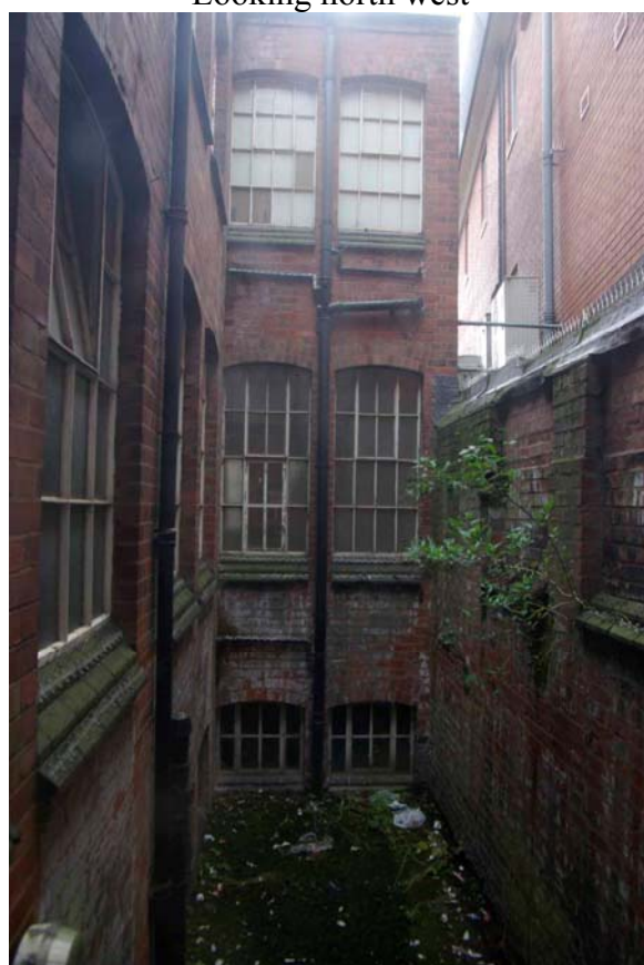
Figure 27 Lightwell/courtyard on west side of building Looking south west towards south range (taken through glass)
