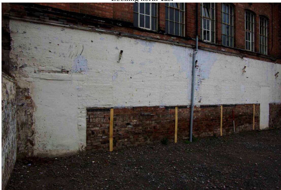
Figure 15 South-west facing elevation basement wall Looking north-east. 1m scale. Note blocked windows
