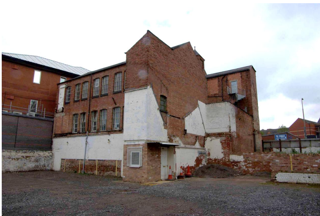
Figure 13 South-west and south-east facing elevations Looking north. Note retaining wall on right of photograph showing difference in ground levels
