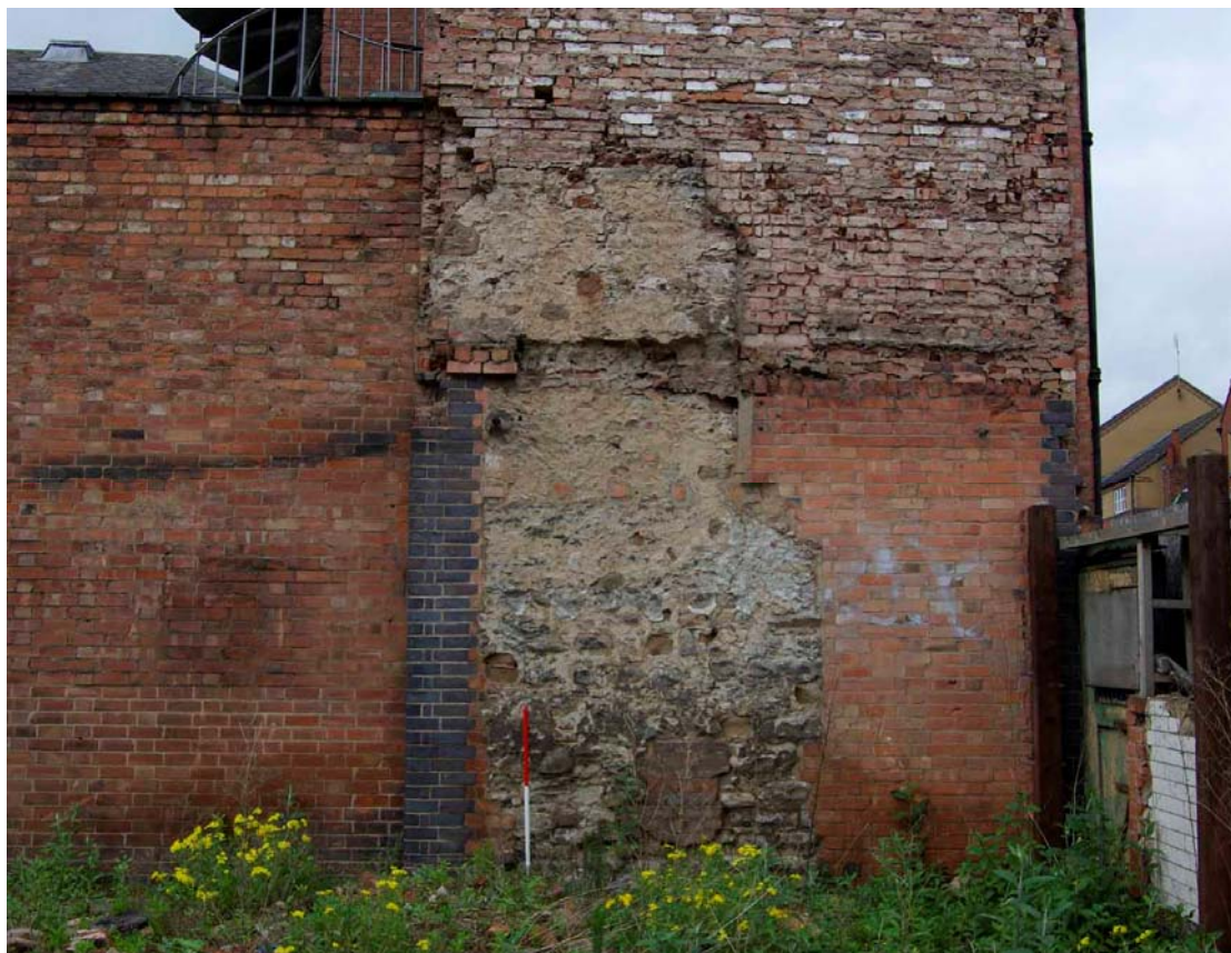
Figure 12 Scar of stone building on south west facing elevation Looking north-east. 1m scale
