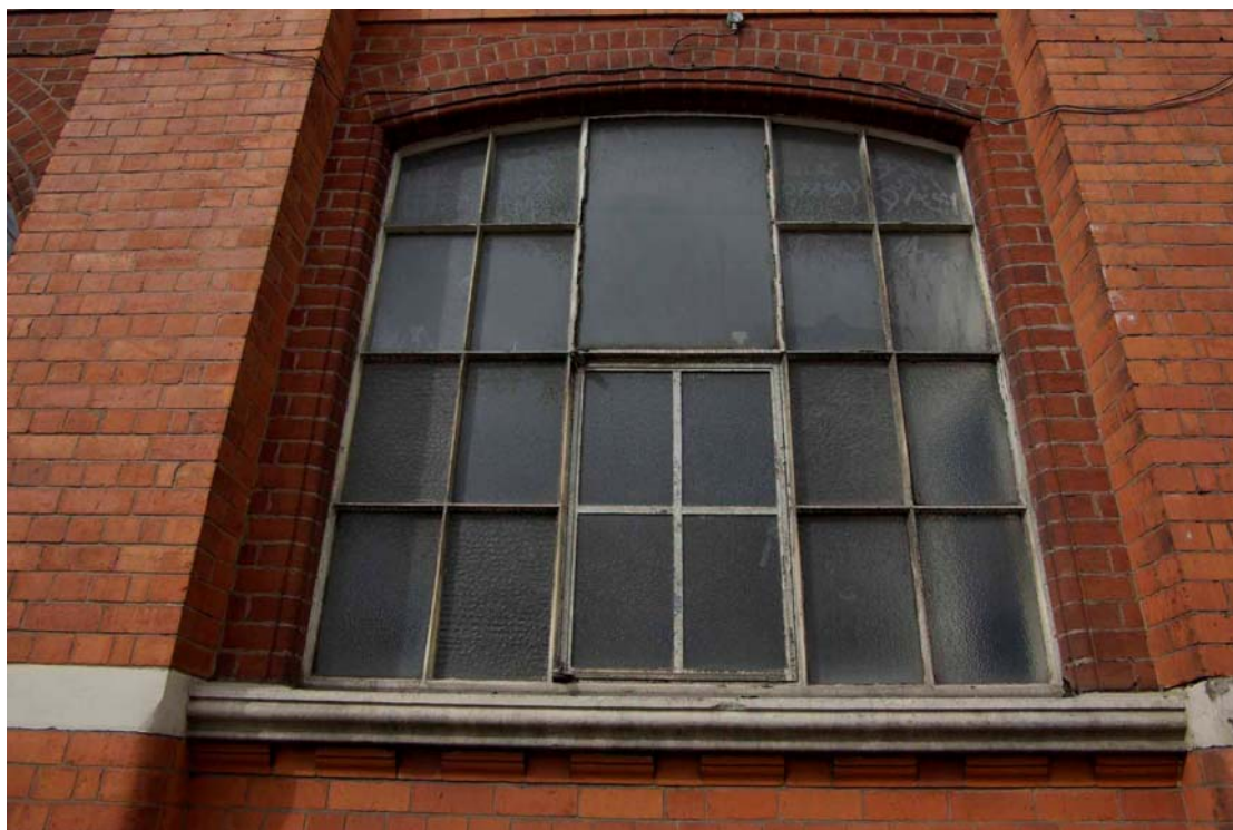
Figure 8 North east facing elevation window detail Note decorative brickwork below stone sill
