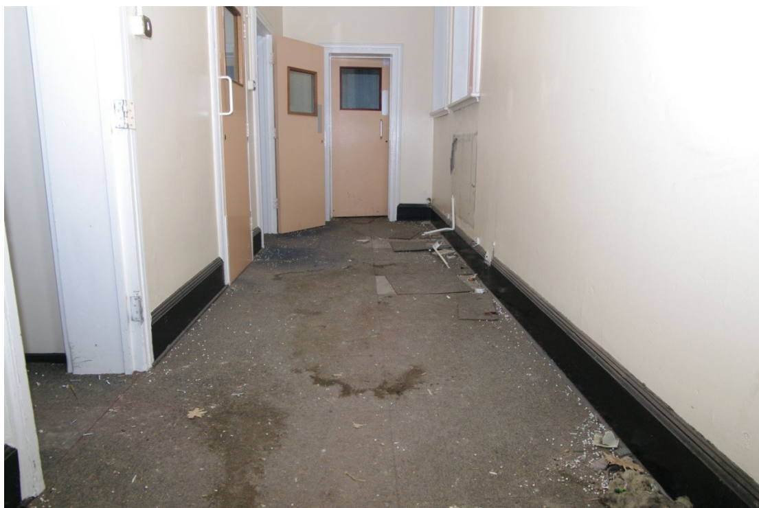
Figure 28 Zone 2 ground floor photo 25 skirting boards
