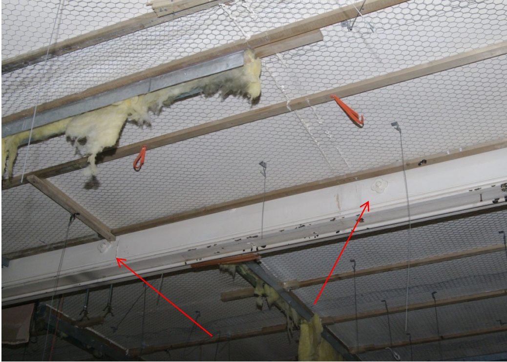
Figure 5 Zone 1 ground floor photo 3 ceiling joists Note decorative bolts (arrowed)
