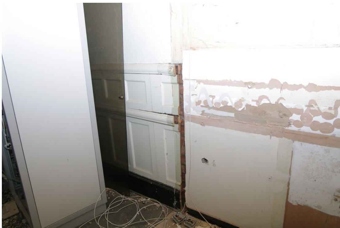
Figure 17 Zone 1 first floor photo 15 truncated panelling
