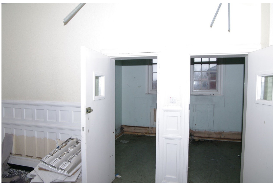
Figure 33 Zone 2 first floor photo 30 day room panelling and probable panelled doors to cells
