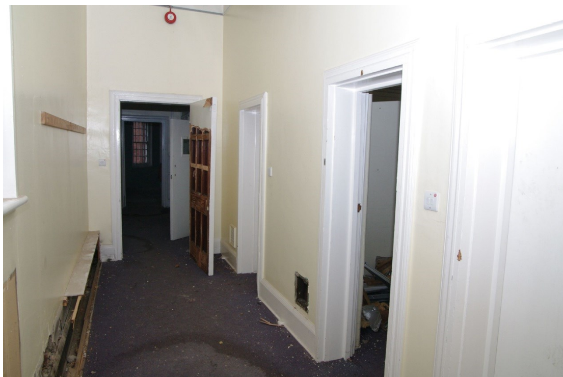
Figure 37 Zone 2 first floor photo 34 cell corridor with panelled doors, surrounds and skirting
