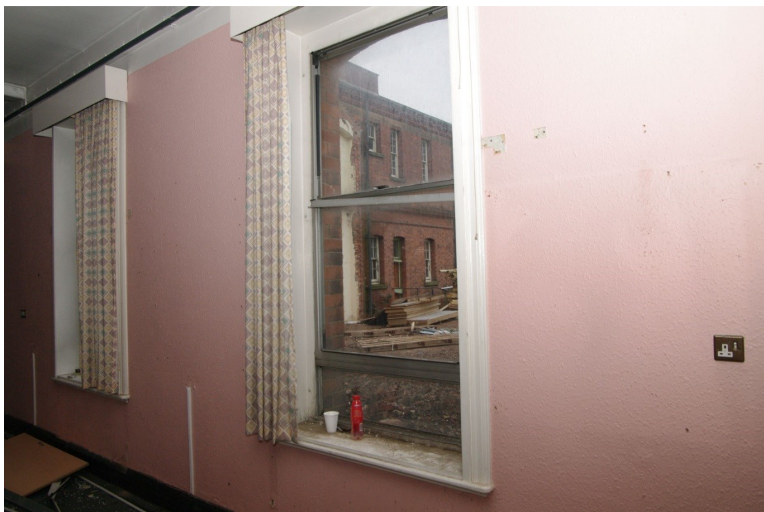
Figure 24 Zone 2 ground floor photo 21 typical window surround
