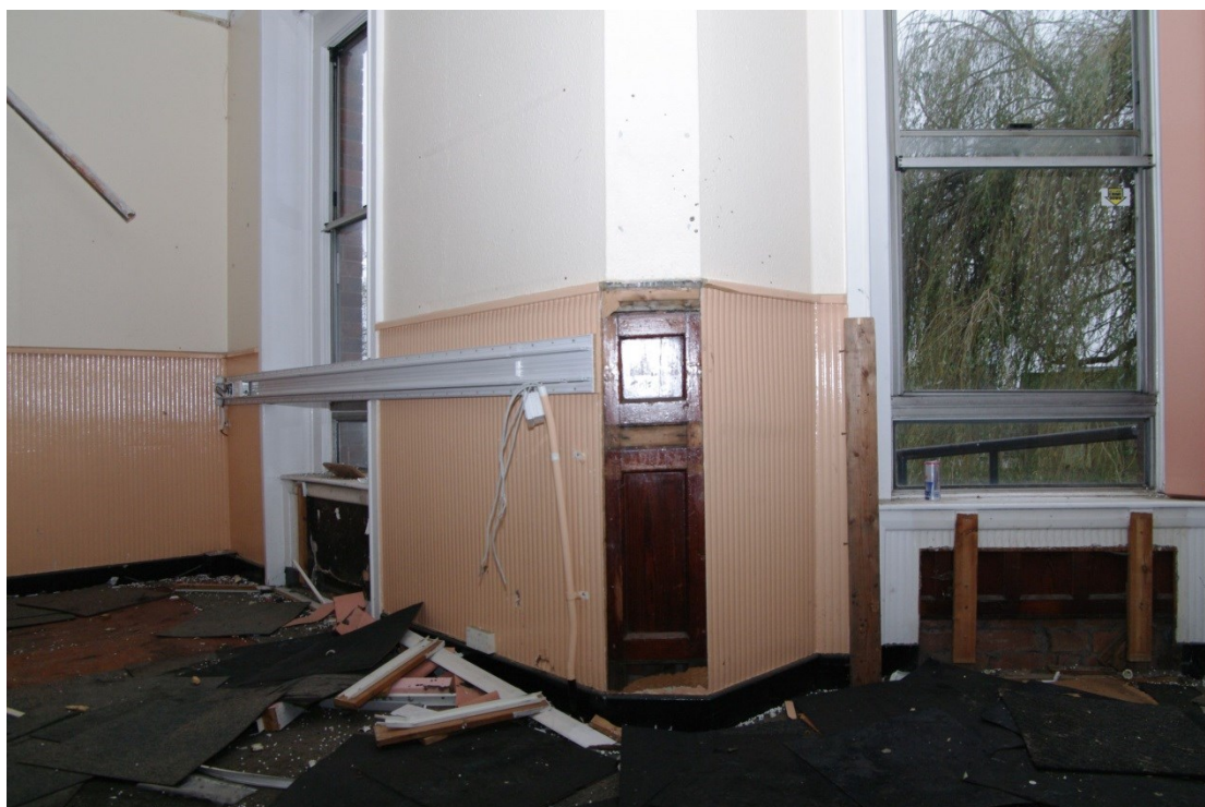
Figure 26 Zone 2 ground floor photo 23 day room panelling behind later sheeting
