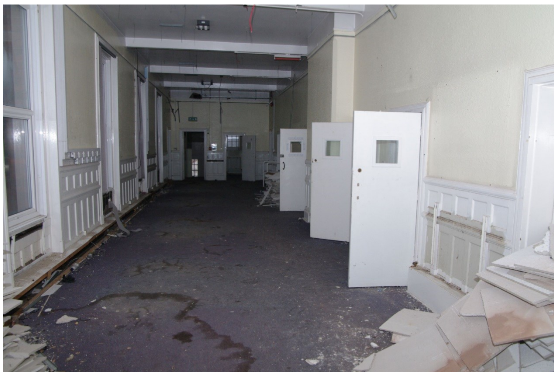
Figure 34 Zone 2 first floor photo 31 corridor attached to day room with panelled cell doors and walls
