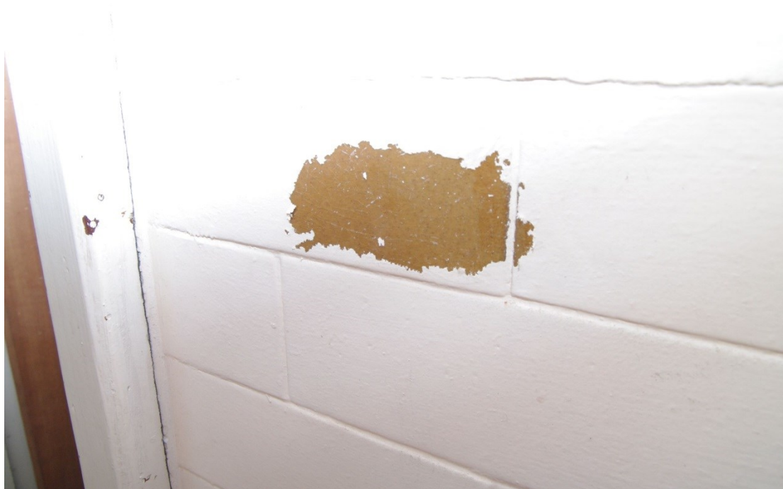
Figure 30 Zone 2 ground floor photo 27 glazed bricks with paint removed
