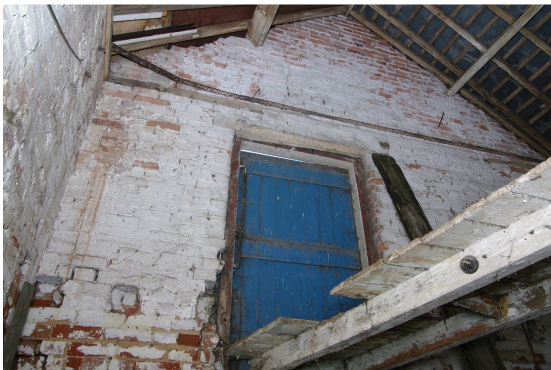
Figure 15 Barn, north room hayloft door Looking north-east. The timber walkway from the hayloft door leads to the first floor of the south room
