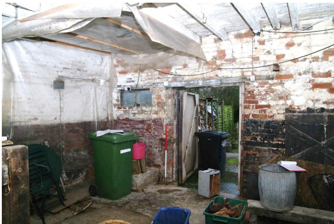
Figure 17 Barn, south room Looking south-west. 1m scale. Note plinth for milling machine beneath pink bucket. Blocked doorway into farmhouse behind green bin and plastic sheeting
