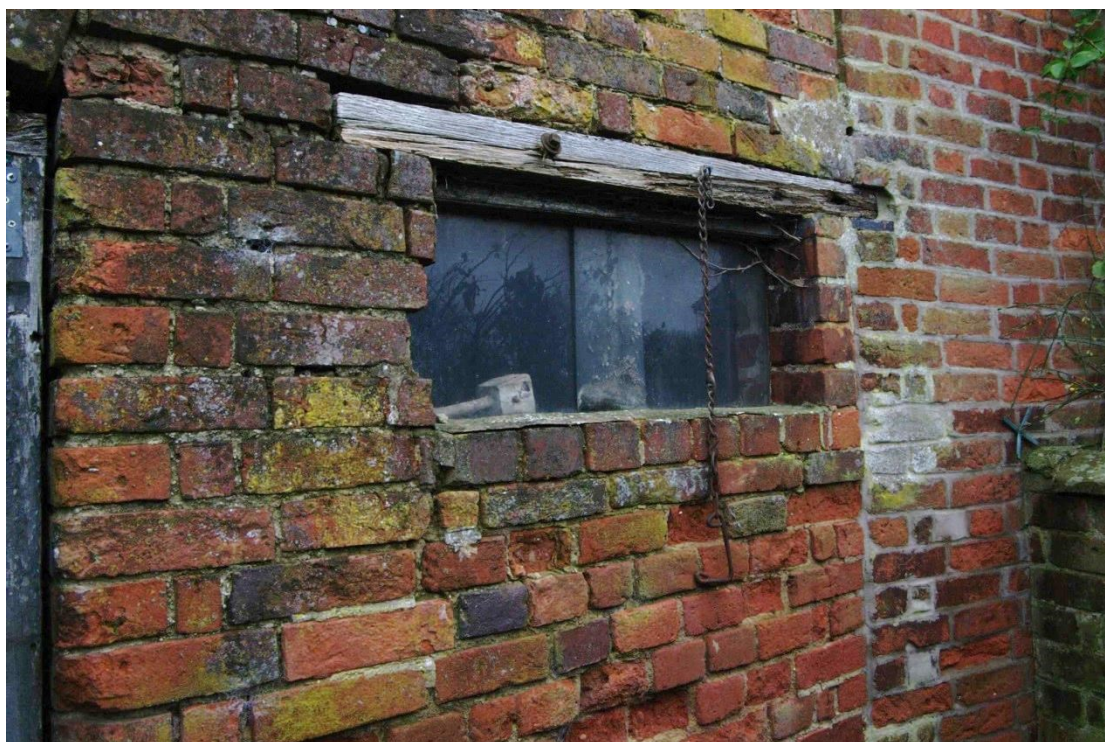
Figure 13 Barn, east facing elevation ground floor window Looking south-east. Note joint with farmhouse to right of window
