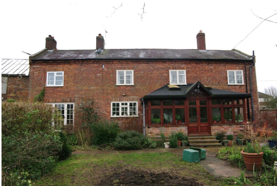
Figure 22 Farmhouse, west facing elevation Looking east. Barn on left of picture. Bay proposed for demolition on right
