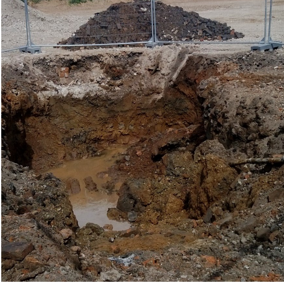
Figure 6 Trench excavated to remove contaminated land in Area 1 viewed from the west
