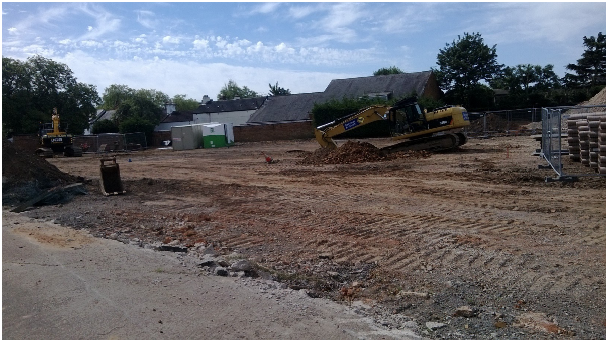
Figure 5 View from north-east of area during groundworks for access road and removal of contaminated land.
