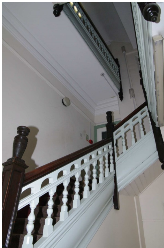
Figure 38 G3 stairs and landing up to first and second floors Looking east
