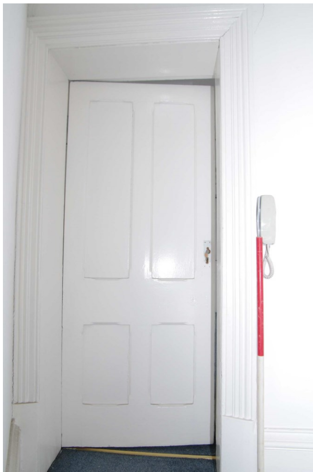
Figure 52 F2 Looking east. 1m scale. Doorway to corridor on left, door to F3 in centre. Note kink in north-east wall
