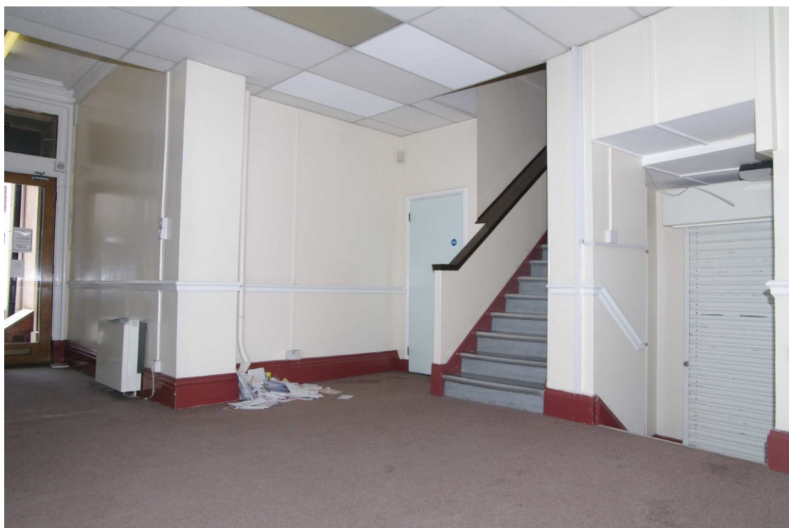
Figure 34 Ground floor G2 Looking west. Entrance G1 on left, stairs to first floor of 54 and 56 centre right, steps down to stairs to rear extension on right
