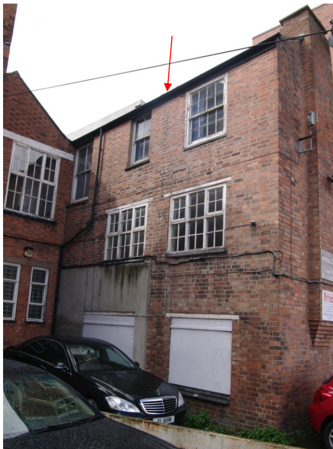
Figure 21 South-east facing elevation of extension to rear of Number 56 Looking west. Arrow indicates joint of two phases
