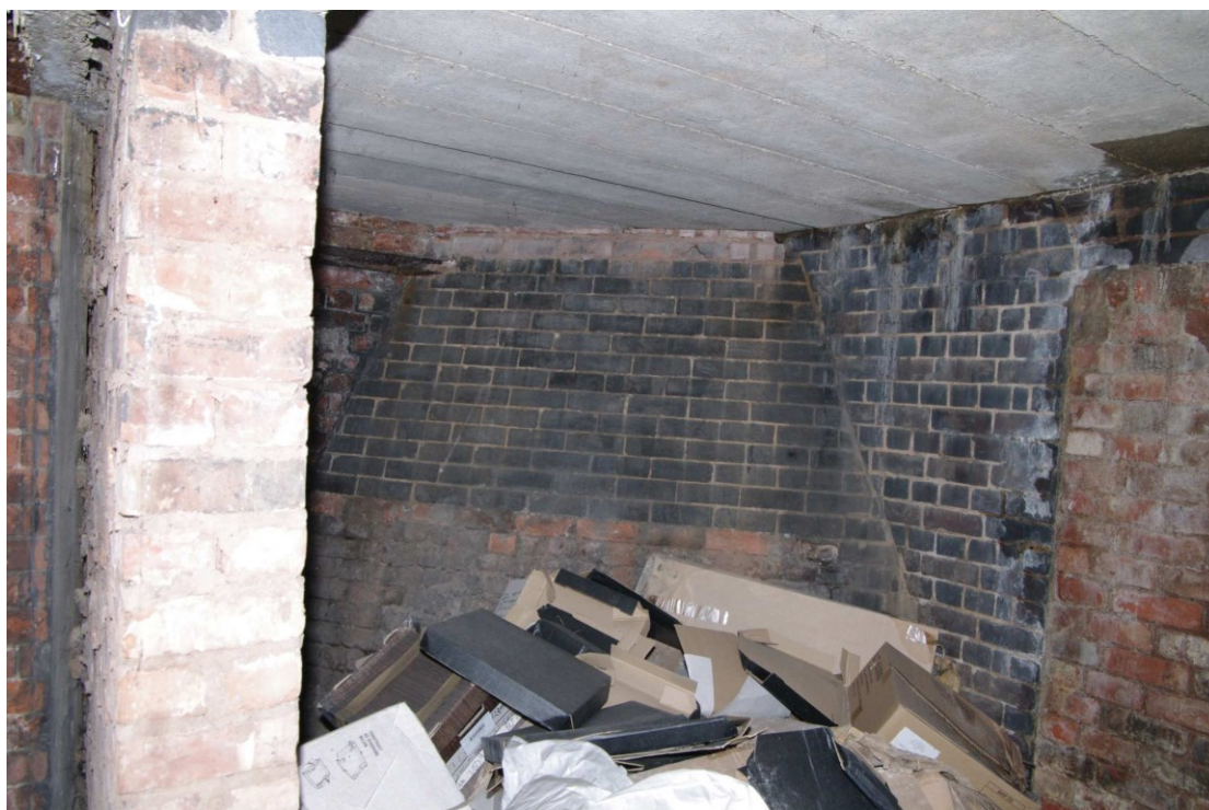
Figure 30 Cellar C3 Looking south. Note sloping wall and double skin of south-east wall on left of picture
