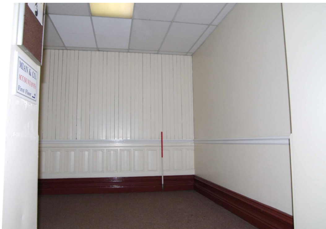
Figure 36 Room G3 Looking south-east. 1m scale. Note inserted wall on right of picture
