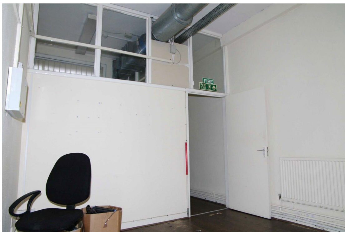
Figure 47 G17 Looking north-east. 1m scale. Note window lights into adjacent room G19
