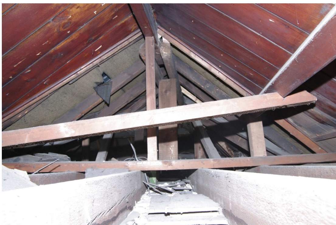
Figure 72 Roof space into Room S1 Looking west through hole in wall of S1
