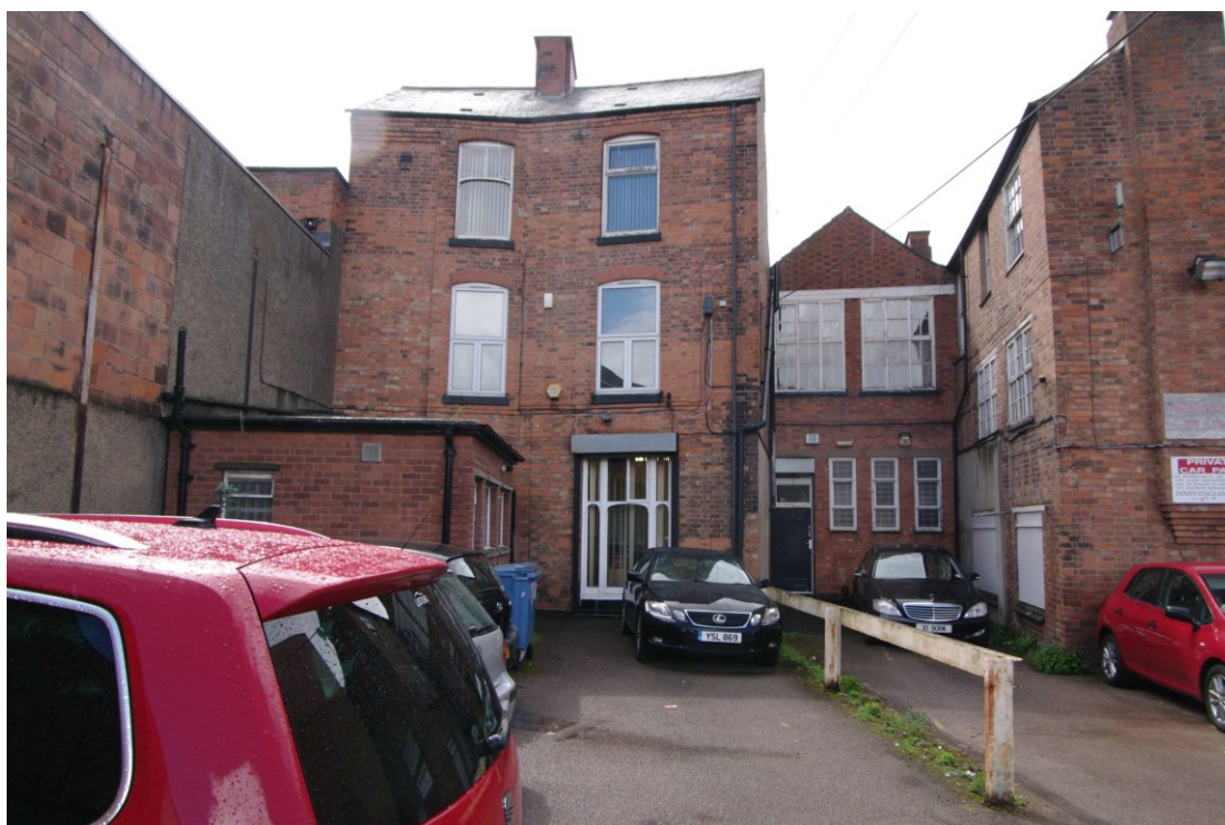
Figure 20 Rear extension of Number 58 Looking south-west. Note kink in building line running down from the chimney stack
