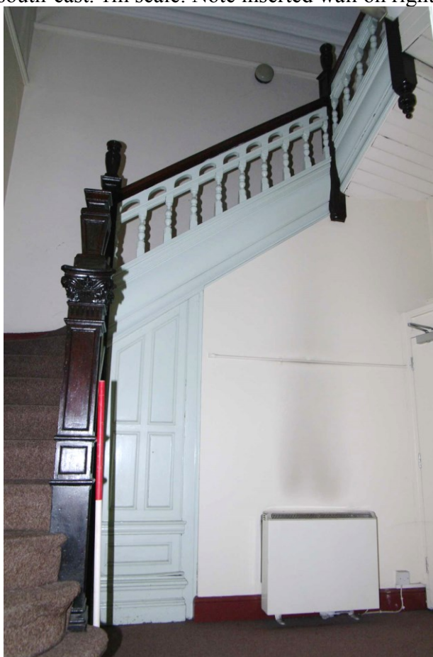
Figure 37 G3 stair case leading up to first floor Looking north-east. 1m scale. Possible blocked entrance to Room G18 behind heater
