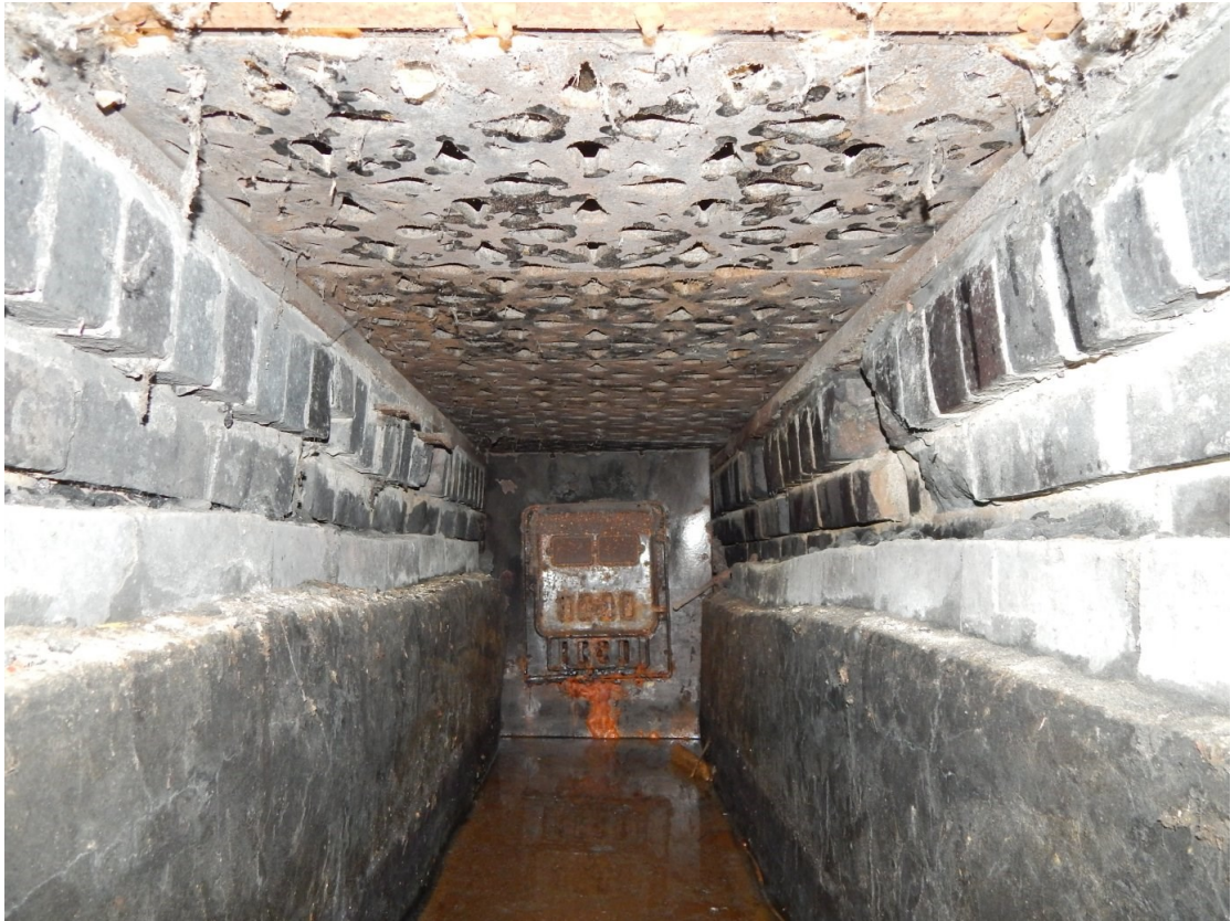
Plate 3: The interior of the heating system at eastern end (T.P 01) looking west
