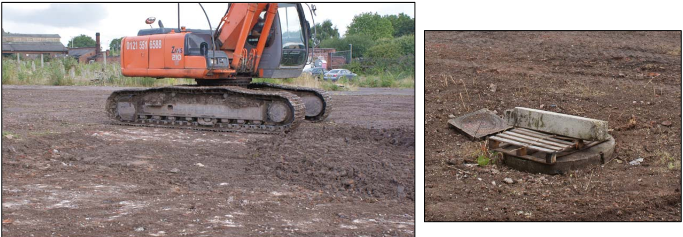
Figure 9: Modern drain running south-east to north-west and lying to the west of the proposed footprint.
