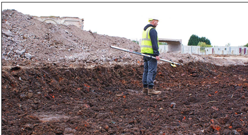
Figure 14: Ground reduction at the northern end of the footprint in the area of the tank.
