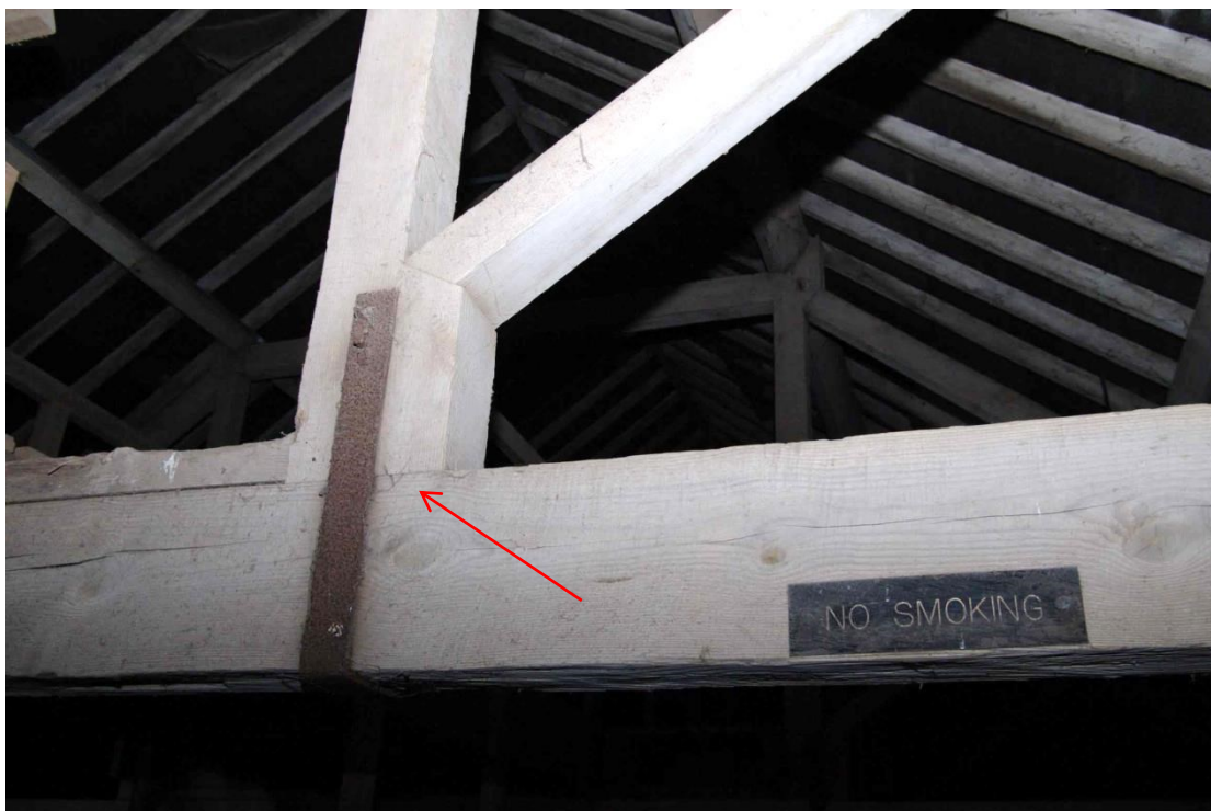
Figure 32: Granary, Room G1 roof detail and carpenter's mark "V" mark indicated by arrow at junction of queen post and truss
