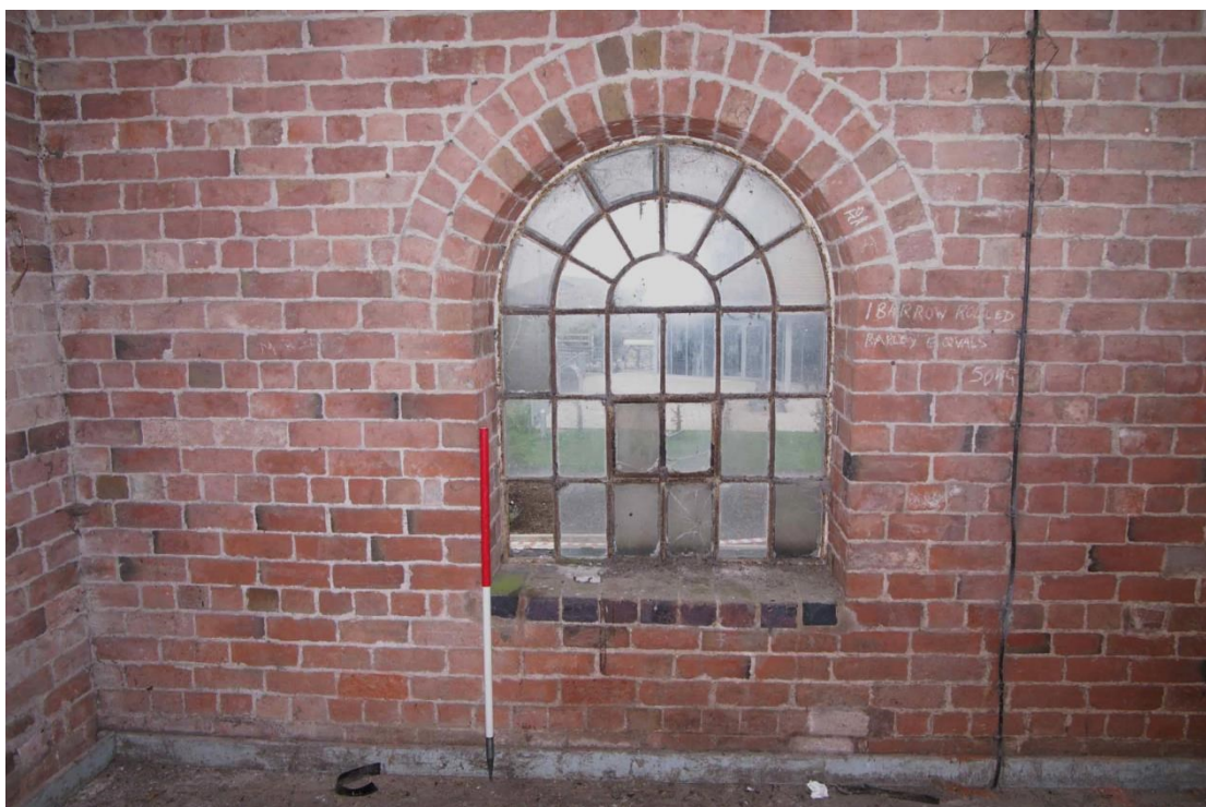
Figure 48: Granary, first floor Room F2. Window detail Looking north. 1m scale. Note chalked graffiti to right of window
