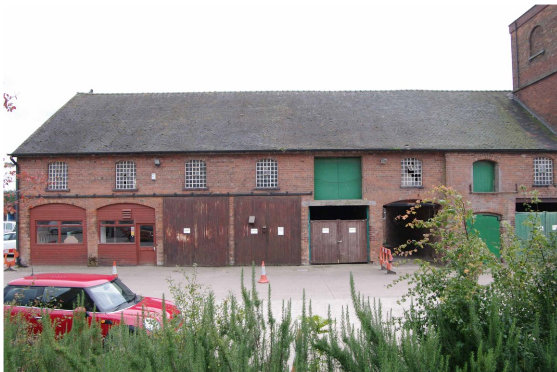
Figure 13: Granary, north facing elevation, eastern end Looking south. Note inserted concrete lintel next to the sliding doors
