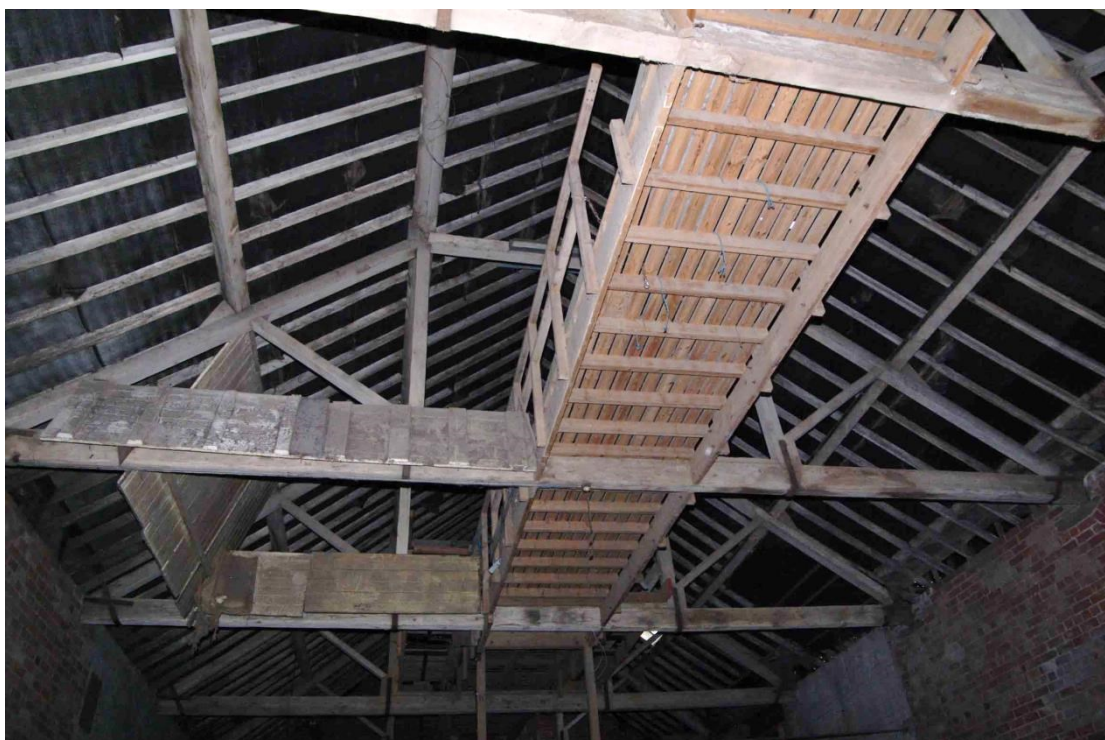
Figure 33: Granary, Room G1 walkway in roof Looking east. Note baffles and other timber structures on left
