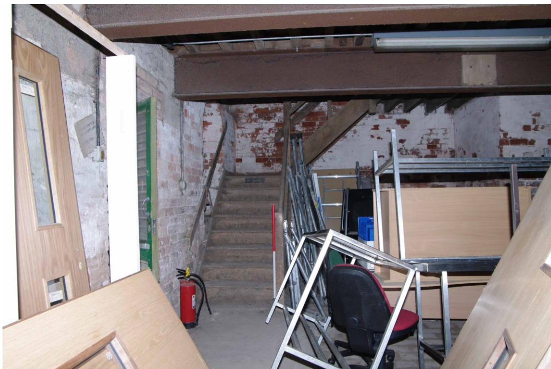
Figure 34: Granary, Room G1 stairs to mezzanine Looking east. 1m scale. Note modern steel beams supporting mezzanine
