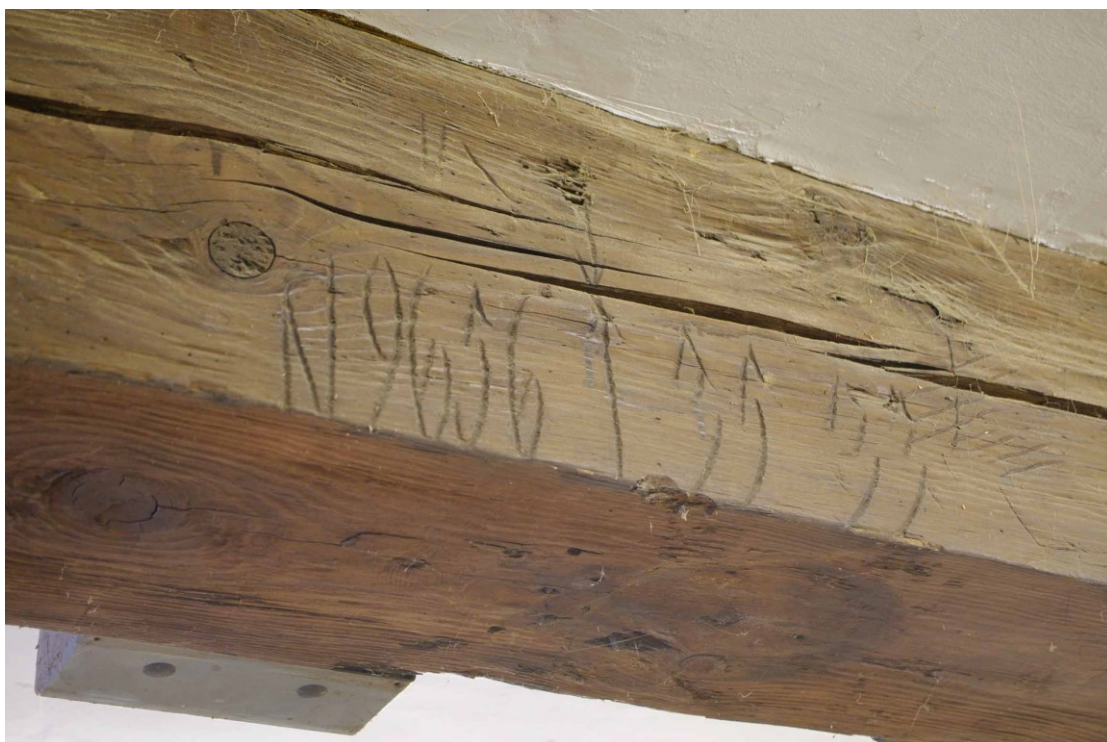
Figure 45: Granary, ground floor Room G7. Raze marks on beam
