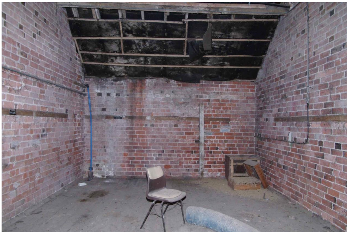
Figure 50: Granary, first floor Room F3 Looking south. Note rail with labels on around room
