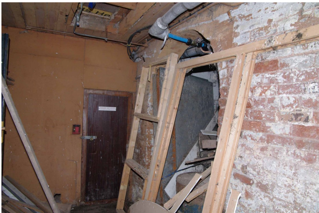
Figure 38: Granary, ground floor. Entrance to Room G3 on right Looking south-west. Photograph taken from Room G4 with modern partition on right
