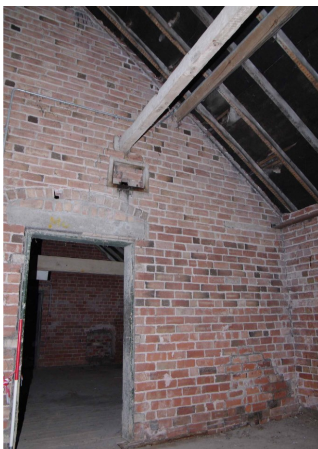
Figure 57: Granary, first floor Room F5 Bearing box on west wall (above door). Looking north-west. 1m scale
