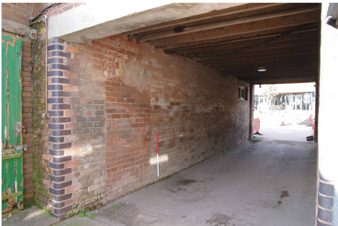
Figure 41: Granary, passageway and outside wall of Room G5 Looking north-west. 1m scale. Blocked doorway to left of scale
