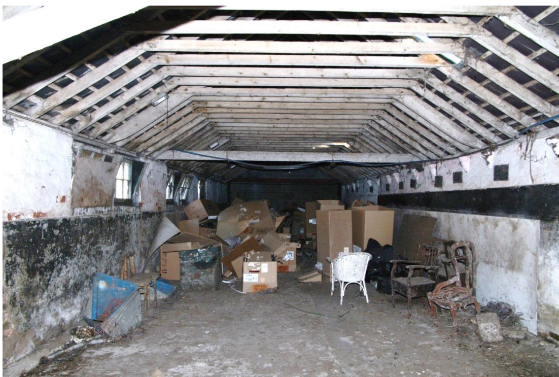
Figure 24 Unit 1, Building 3 Looking north-east. Roller shutter door into Building 2 at far end
