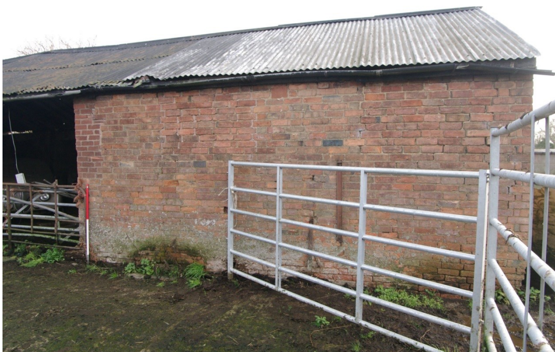
Figure 26 Unit 1, Building 4 north-west facing elevation southern end Looking south-east. 1m scale. Note multiple brick joints
