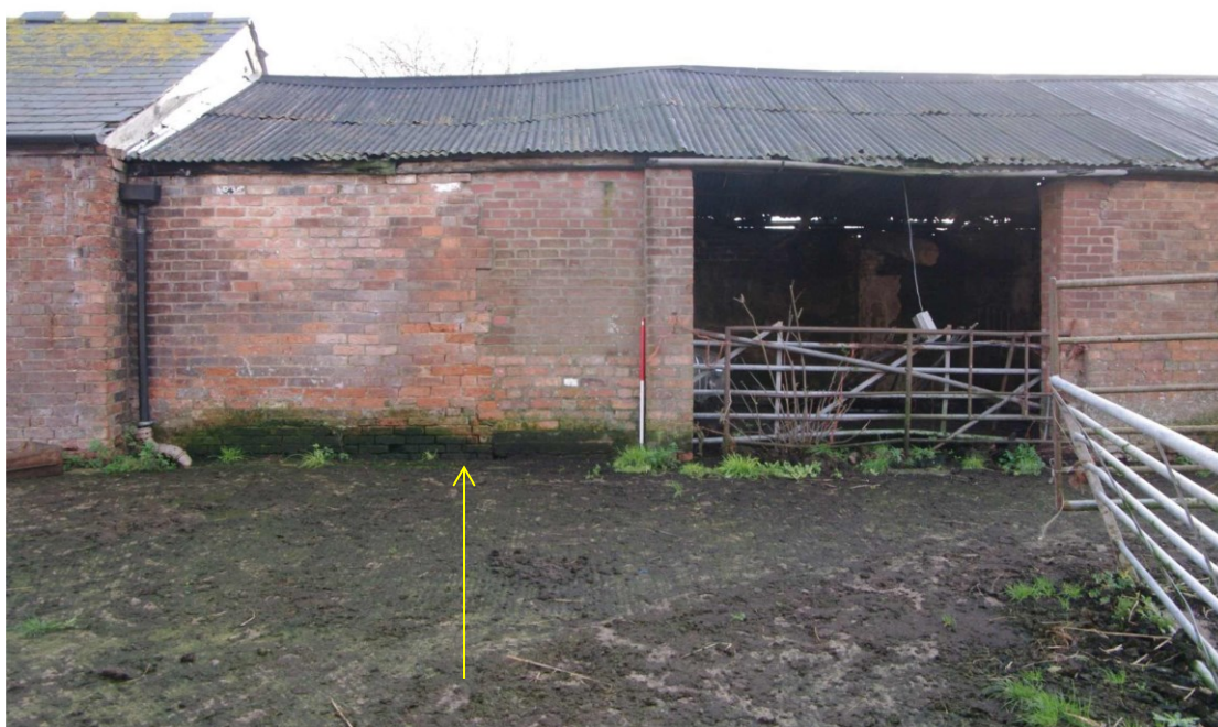
Figure 25 Unit 1, Building 4 north-west facing elevation Looking south-east. 1m scale. Note joint with modern brickwork (on right)
