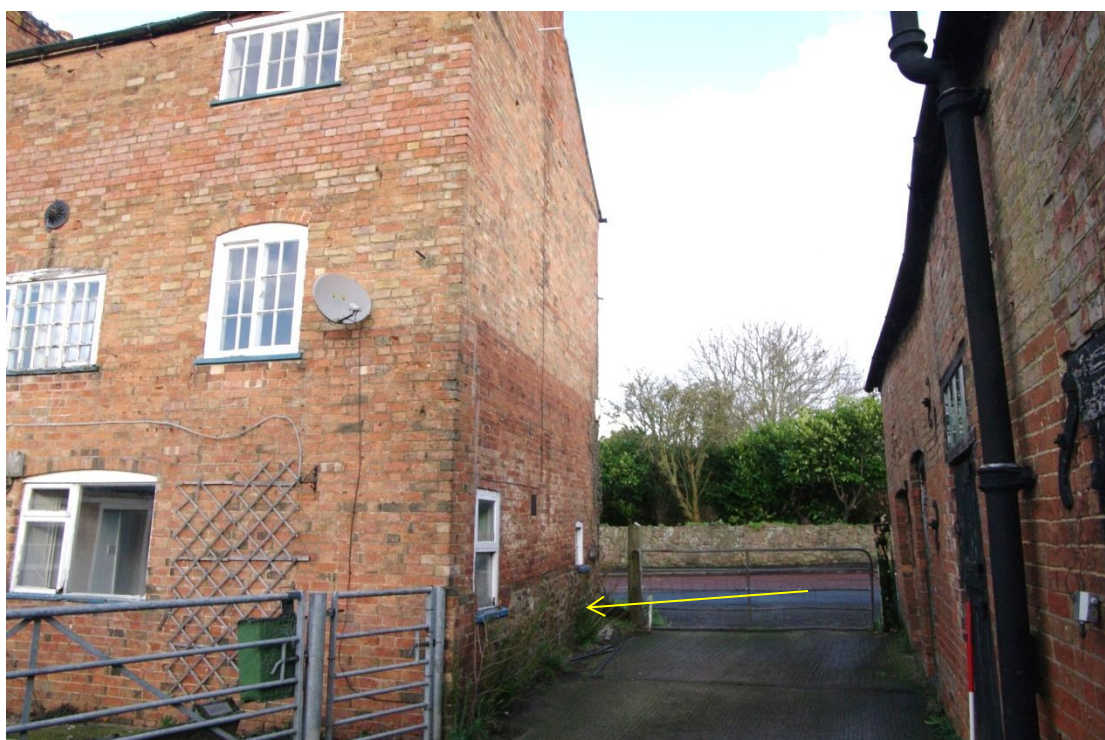
Figure 5 East end of Limes Farmhouse Looking north. Note stone platform (arrowed) and rebuilding line in the brickwork on the gable end. Unit 1 buildings on right of picture
