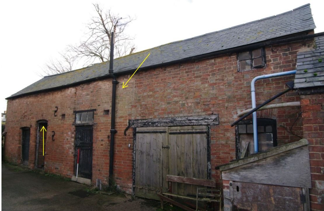
Figure 12 Unit 1, Building 1 north-west facing elevation Looking north-east. 1m scale. Note changes in brickwork (arrowed)
