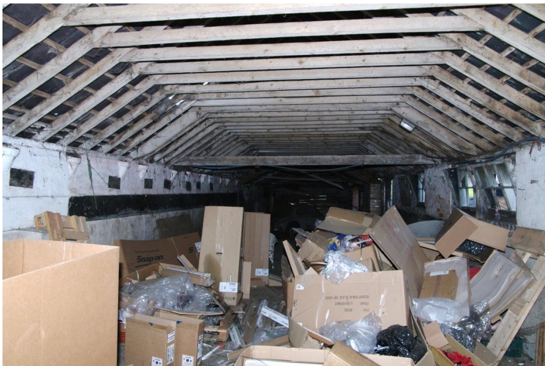
Figure 23 Unit 1, Building 3 inside Looking south-west. Note black plaques to hold the cow's names
