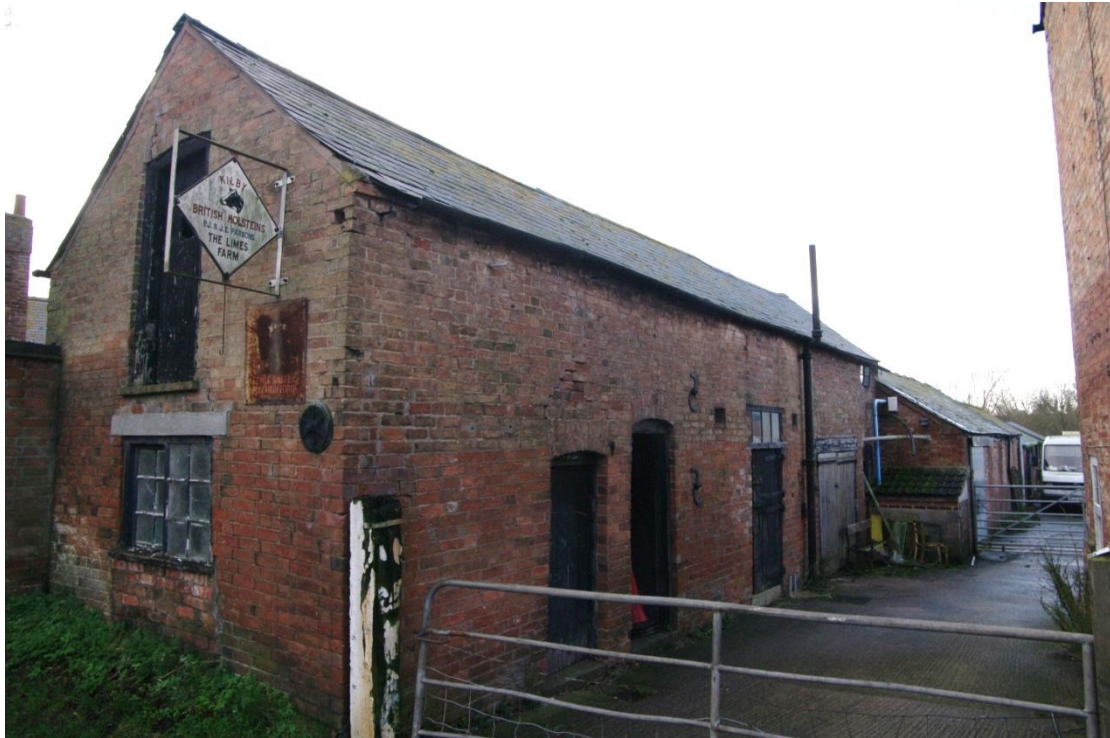
Figure 11 Unit 1, Building 1 north-east and north-west facing elevations Looking south. Note the rest of the Unit 1 buildings continuing down the slope
