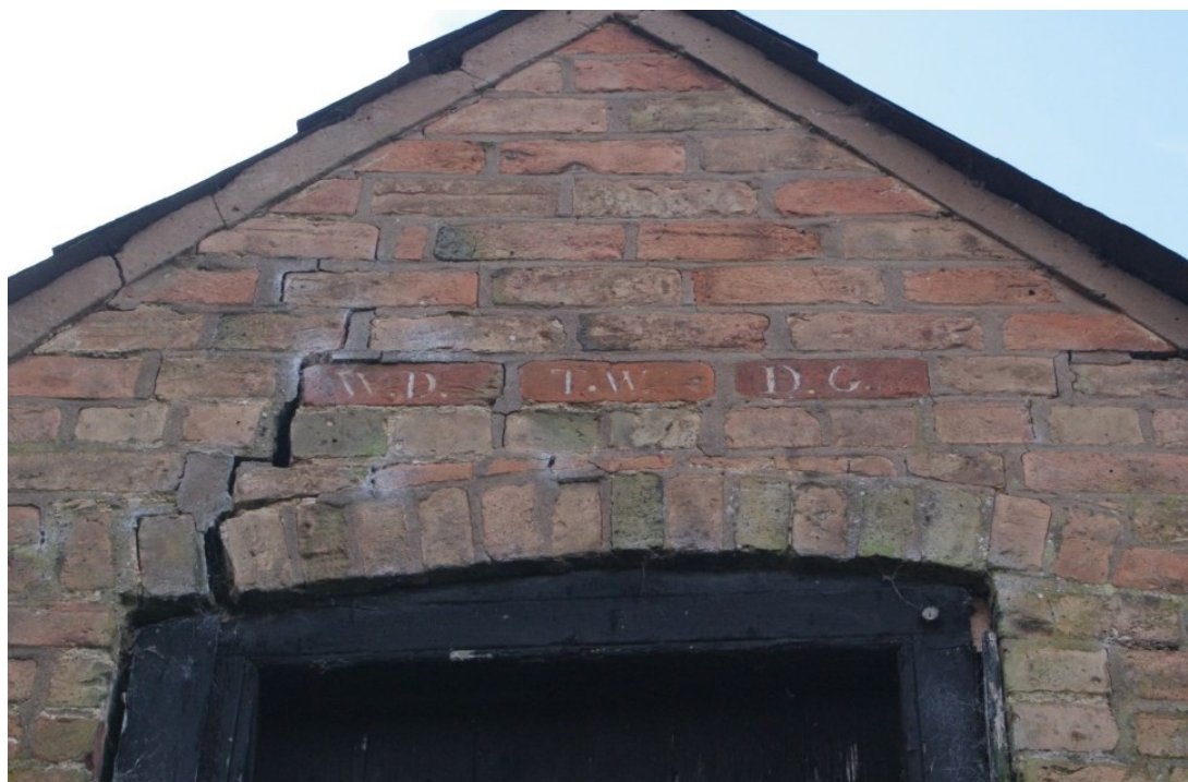
Figure 10 Unit 1, north-east facing elevation gable end bricks above hayloft door Looking south-west
