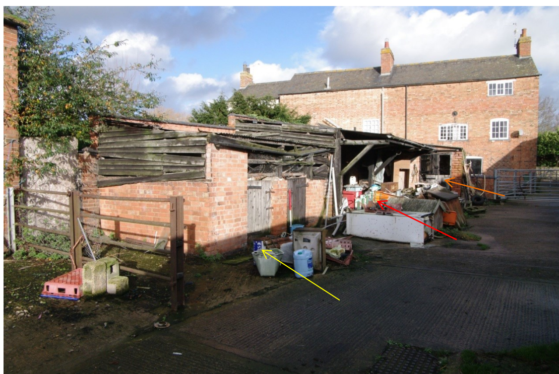
Figure 37 Outbuildings Looking north. 1m scale. Yellow arrow shows the sty, red arrow is the lean-to, orange arrow is the outbuilding
