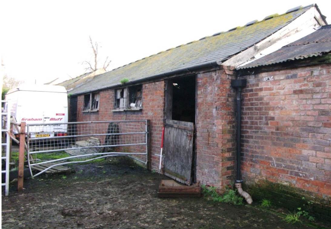
Figure 22 Unit 1, Building 3 north-west facing elevation Looking north-east. 1m scale. Building 3 on right of picture
