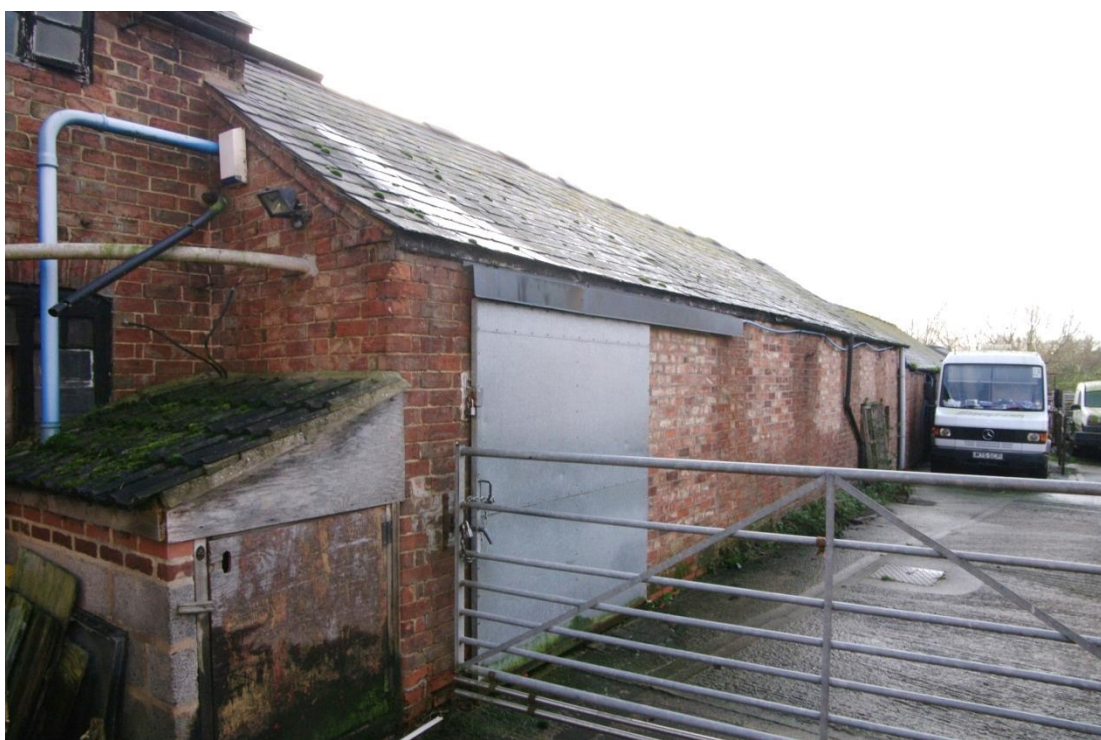
Figure 18 Unit 1, Building 2 north-east and north-west facing elevations Looking south. Note how Building 2 wraps around the corner of Building 1
