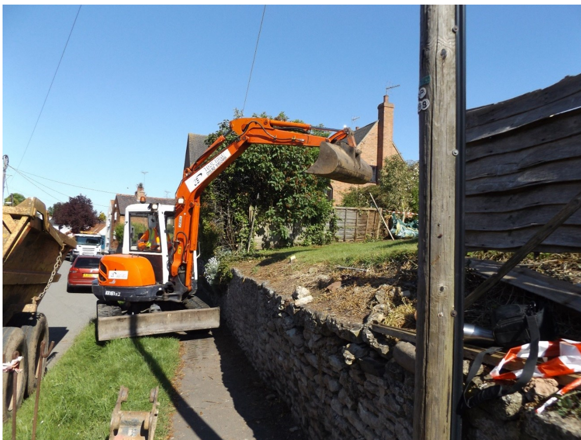
Figure 4: Commencing the removal of the boundary wall and excavation of site access.
