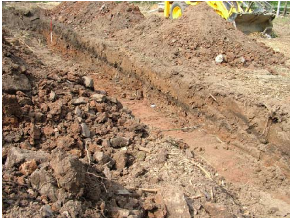
Plate 2: Trench 2, showing topsoil variation in south west facing section. Looking north west
