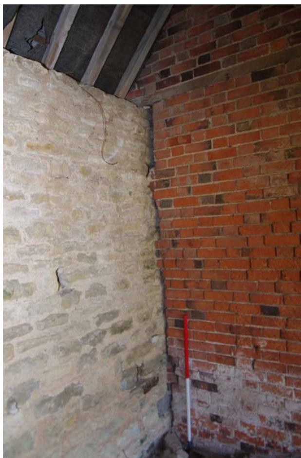
Figure 86: East range, Building D bonding between brick and stone walls Looking south-east, 1m scale
