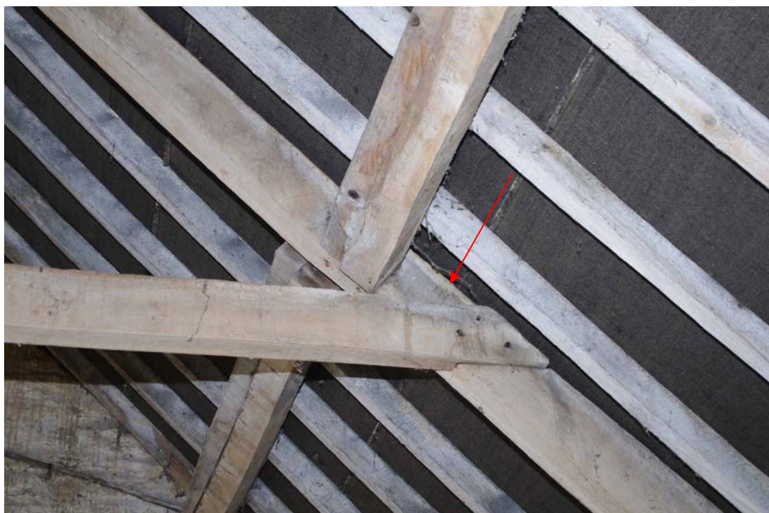
Figure 121: West range, north end of Building G. Roof detail Carpenter's Roman numeral marks arrowed
