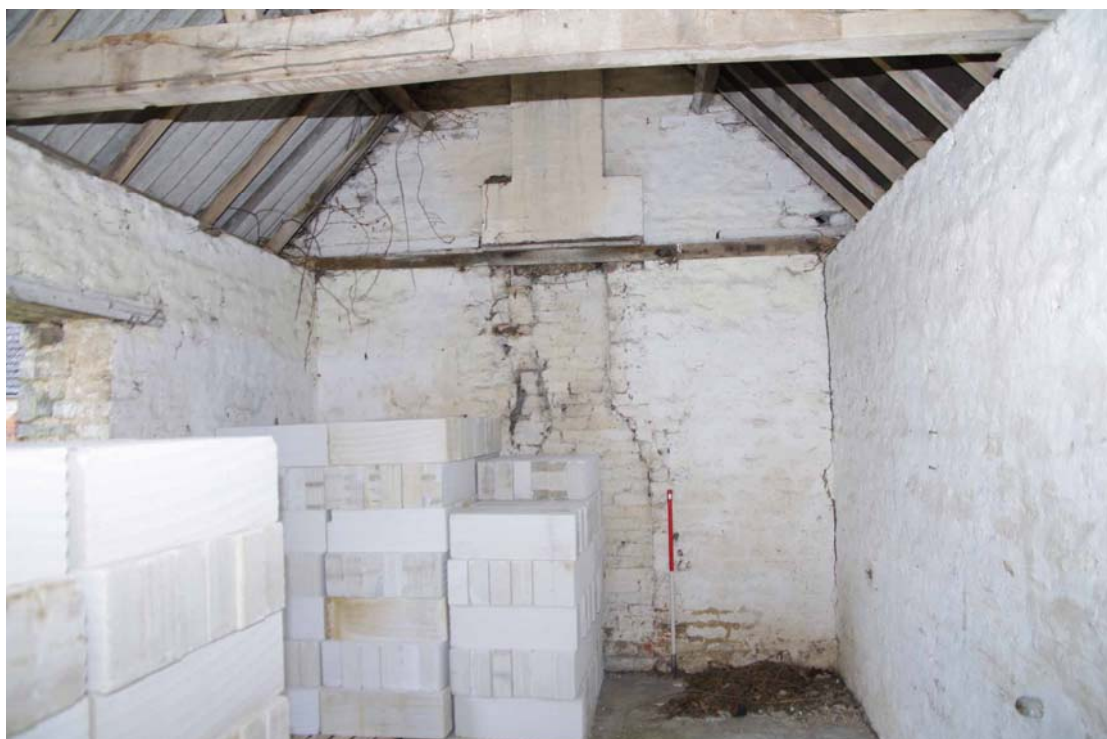
Figure 101: South range, west end room Looking east, 1m scale. Ranging pole is to right of removed fireplace
