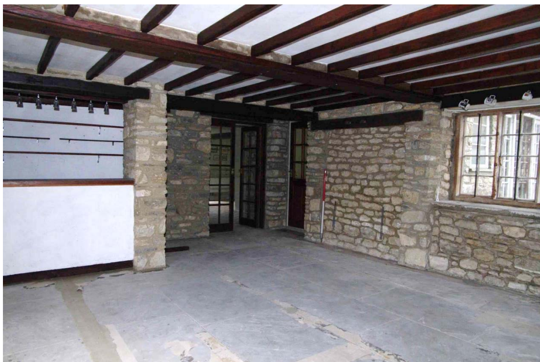
Figure 32: Ground floor, Room G4 Looking north-west, 1m scale. Cellar steps behind bar on left
