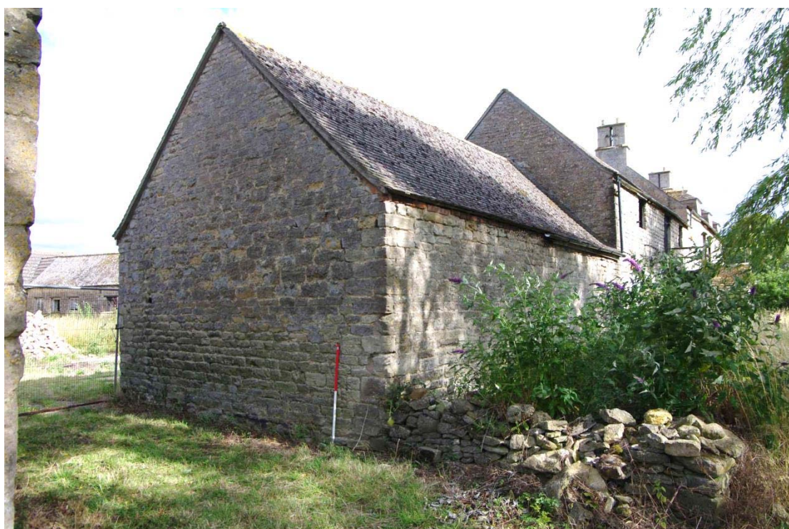
Figure 113: West range, north facing gable end of Building G Looking south-east, 1m scale. Corner of Building A on extreme left
