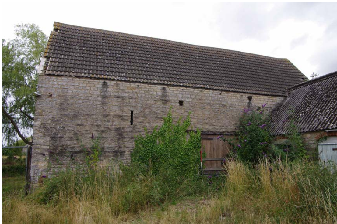
Figure 105: West range, east facing elevation of Building A Looking west, 1m scale
