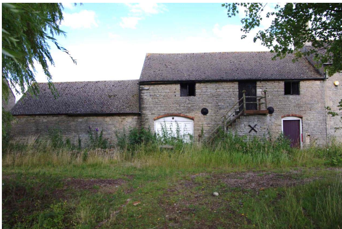
Figure 112: West range, west facing elevation of Building G adjacent to house Looking east, 1m scale
