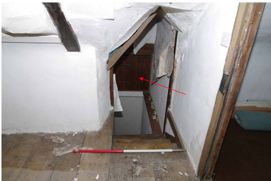
Figure 57: Second floor. Servant's staircase up from F3 into Room S1 Looking east, 1m scale. Note access hatch (arrowed) to roof space of north wing
