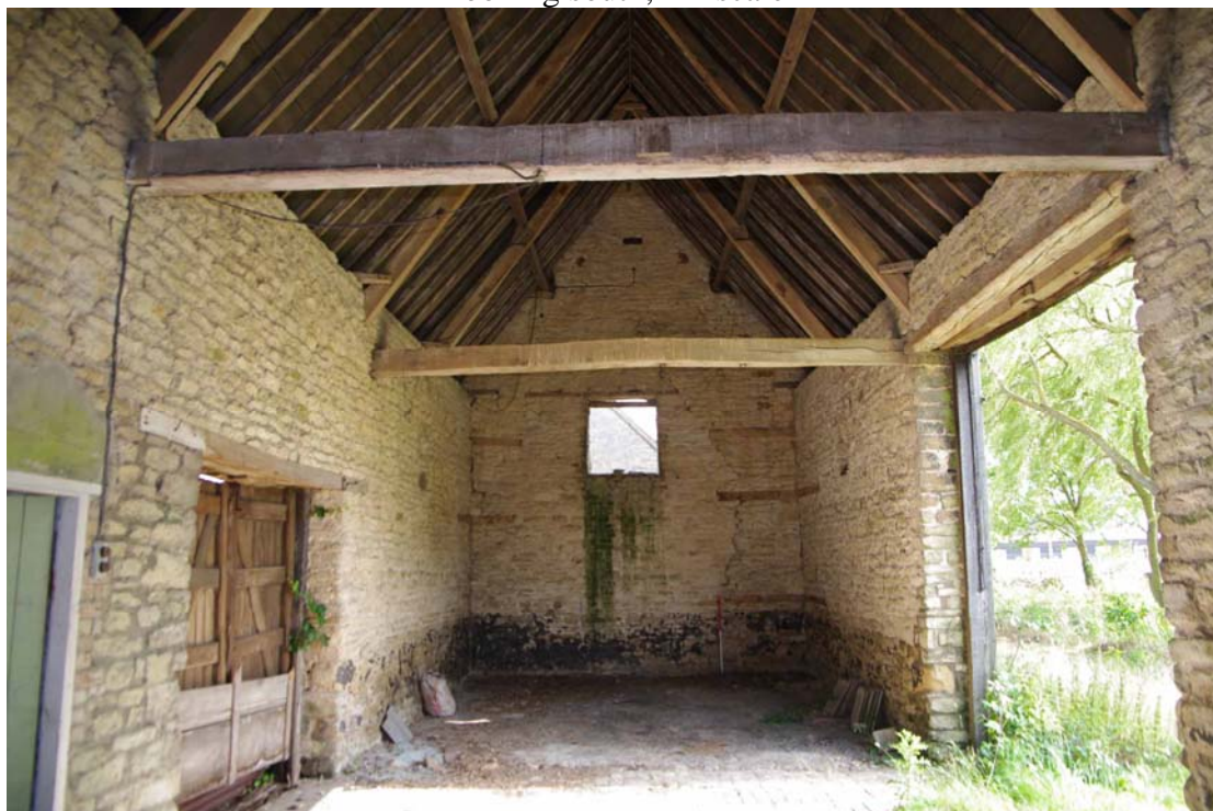
Figure 109: West range, Building A inside Looking south, 1m scale. Note joint of former gable end starting close to scale
