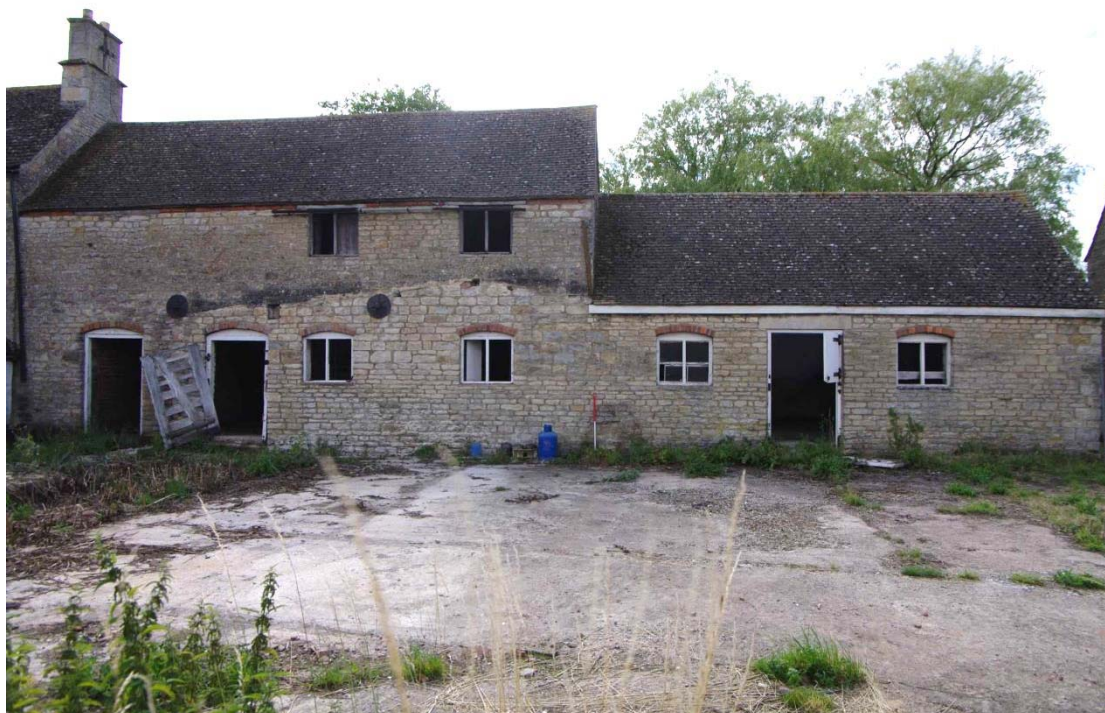
Figure 114: West range, east facing elevation of Building G Looking west, 1m scale. Note scar of recently demolished lean-to
