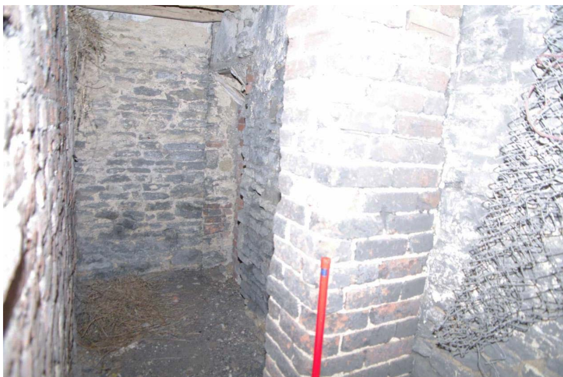
Figure 15: Farm House north facing elevation gable end blocked ground floor doorway. Looking south-east
