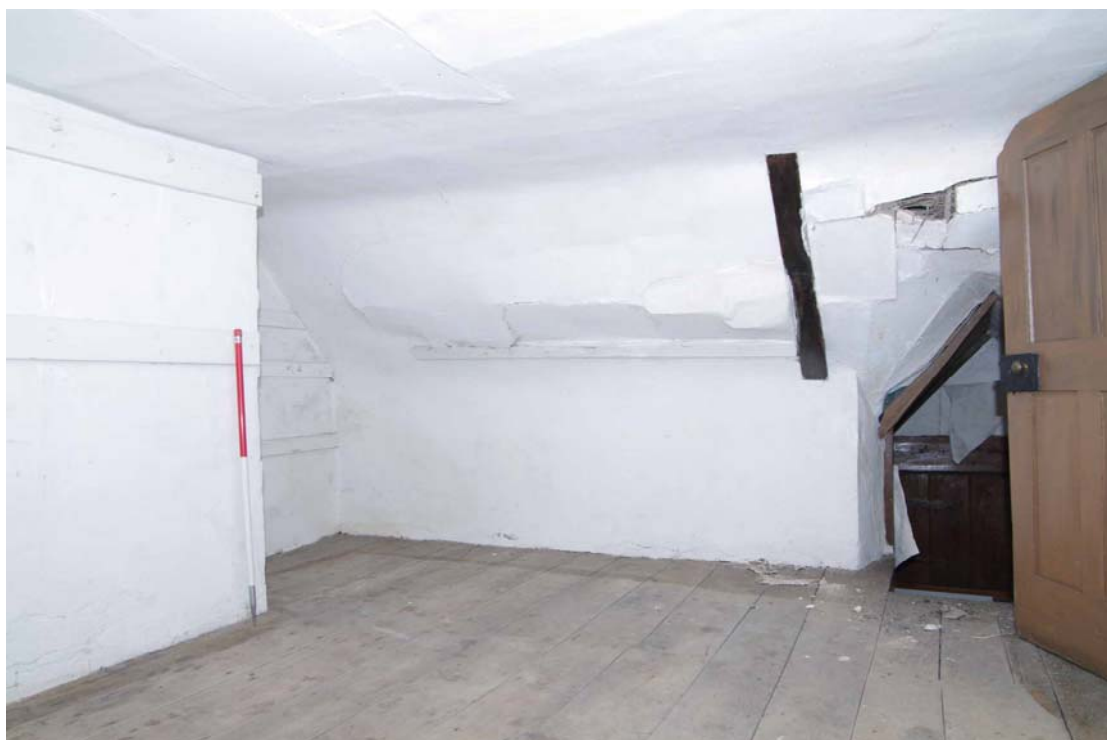
Figure 59: Second floor, Room S1 Looking north-east, 1m scale. Stairs down to F3 to left of door
