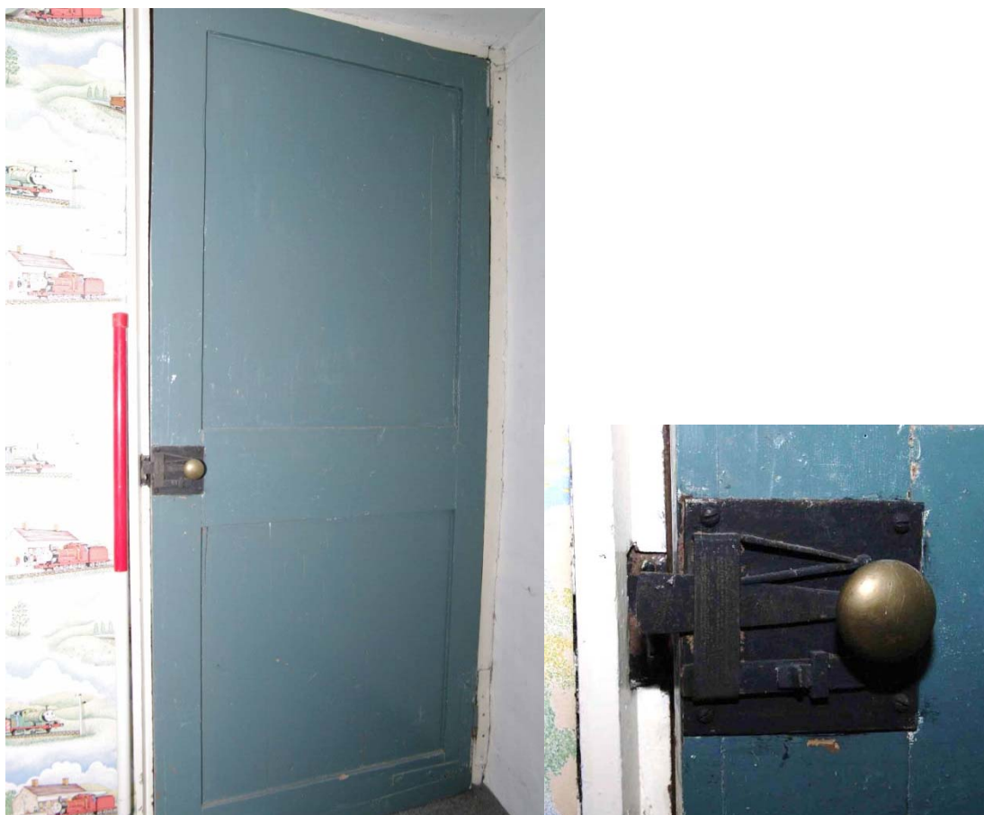
Figure 61: Second floor, Room S2. Door detail Looking east, 1m scale. Latch close-up on right
