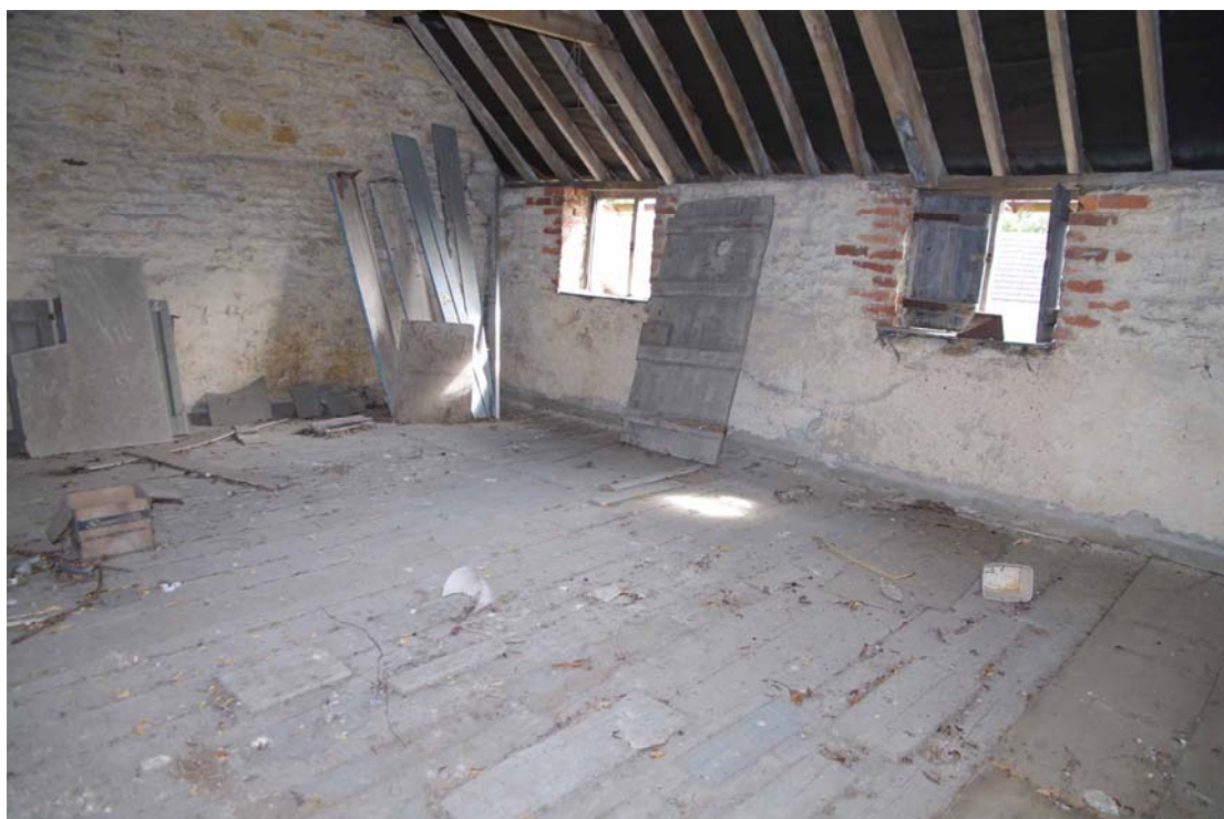
Figure 123: West range, first floor of Building G. North room Looking north-east from entrance doorway
