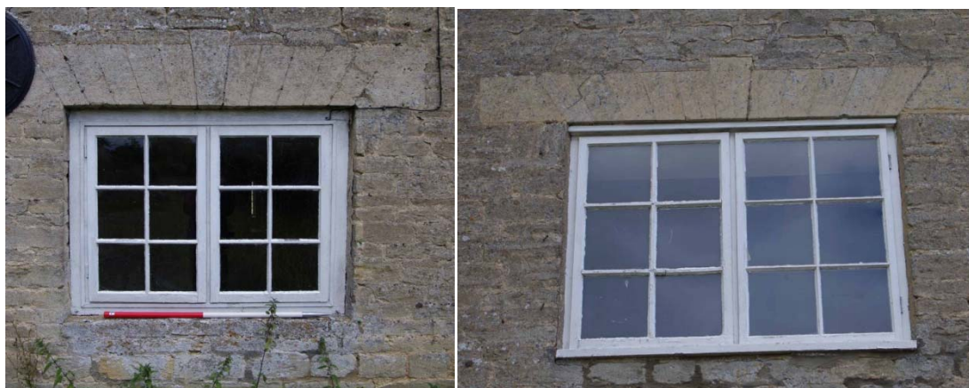
Figure 11 Farm house window details Left: ground floor, right: first floor 1m scale
