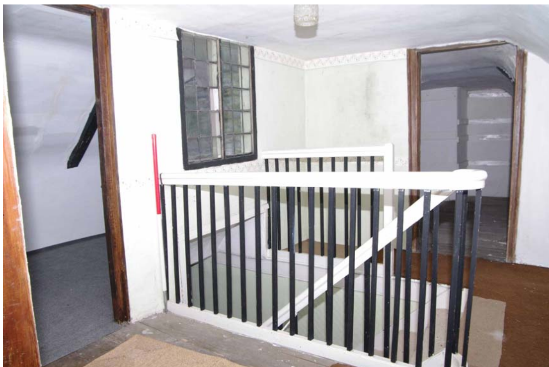
Figure 62: Second floor, outside Room S2 Looking north-west, 1m scale. Door to room S1 on right
