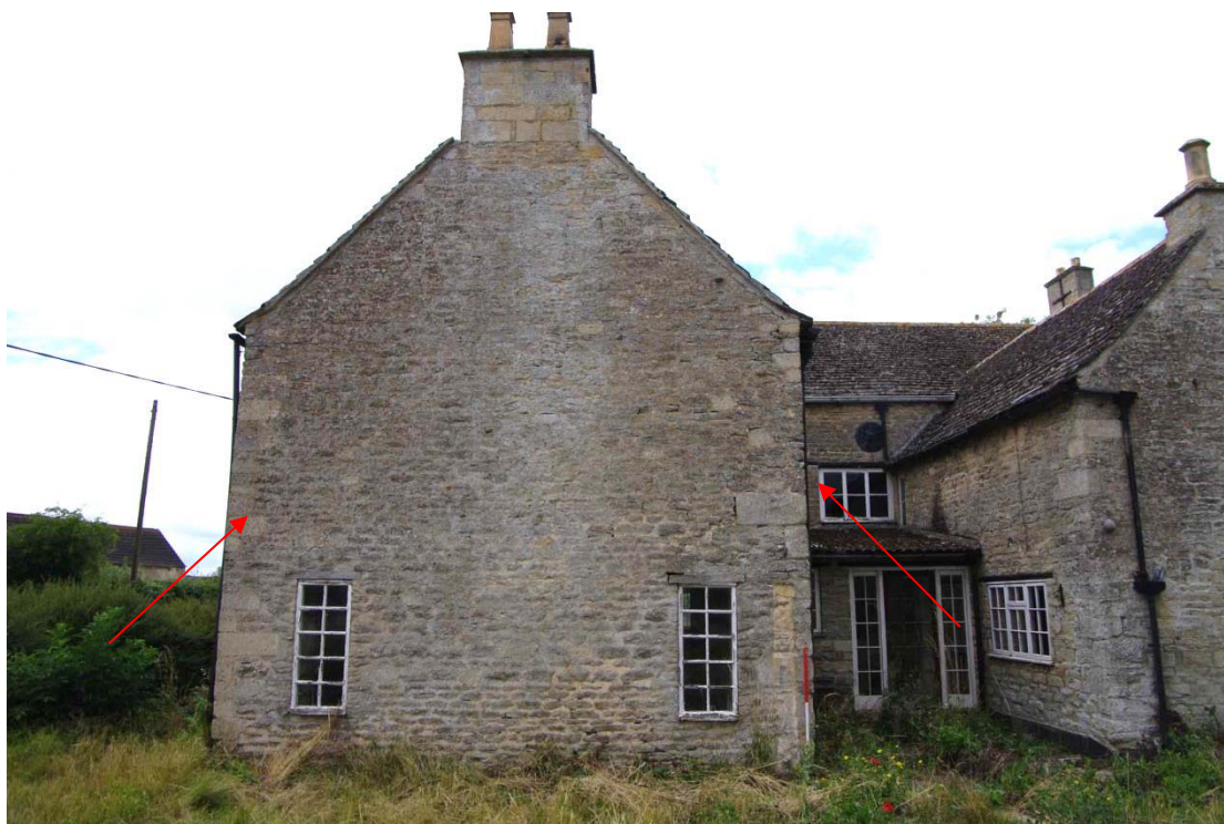
Figure 18: Farm House, rear south wing north facing elevation Looking west, 1m scale. Arrows show line of original gable
