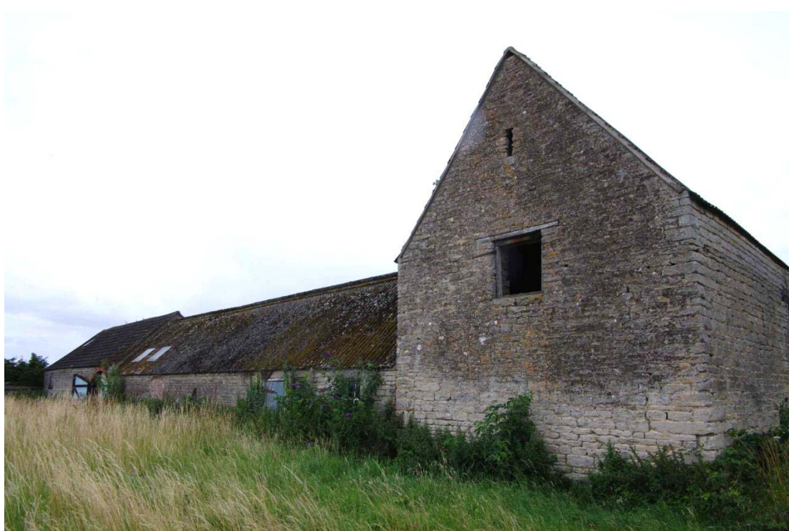
Figure 74: North range, north facing elevation Looking south-east. Building A on right, Building C on far left
