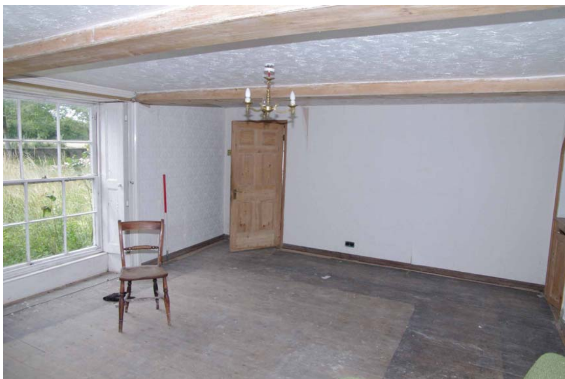
Figure 29: Ground floor, Room G3 Looking north-west, 1m scale. Note arched niche on right
