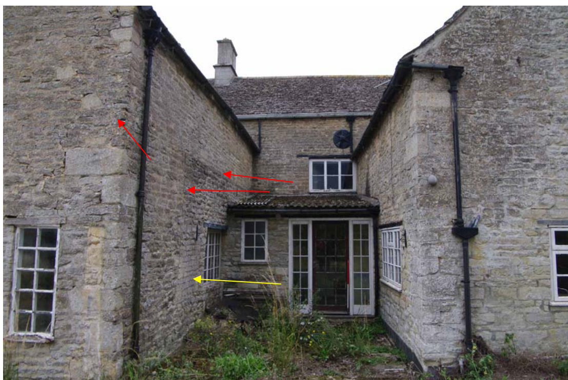
Figure 17: Farm House rear wings showing extension to south wing Looking west, 1m scale. Yellow arrow shows blocked window. Red arrows show joint in walls on southern wing
