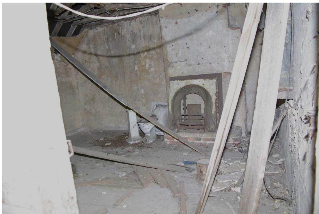
Figure 122: West range, first floor of Building G. Southern room Looking south-east from outside doorway
