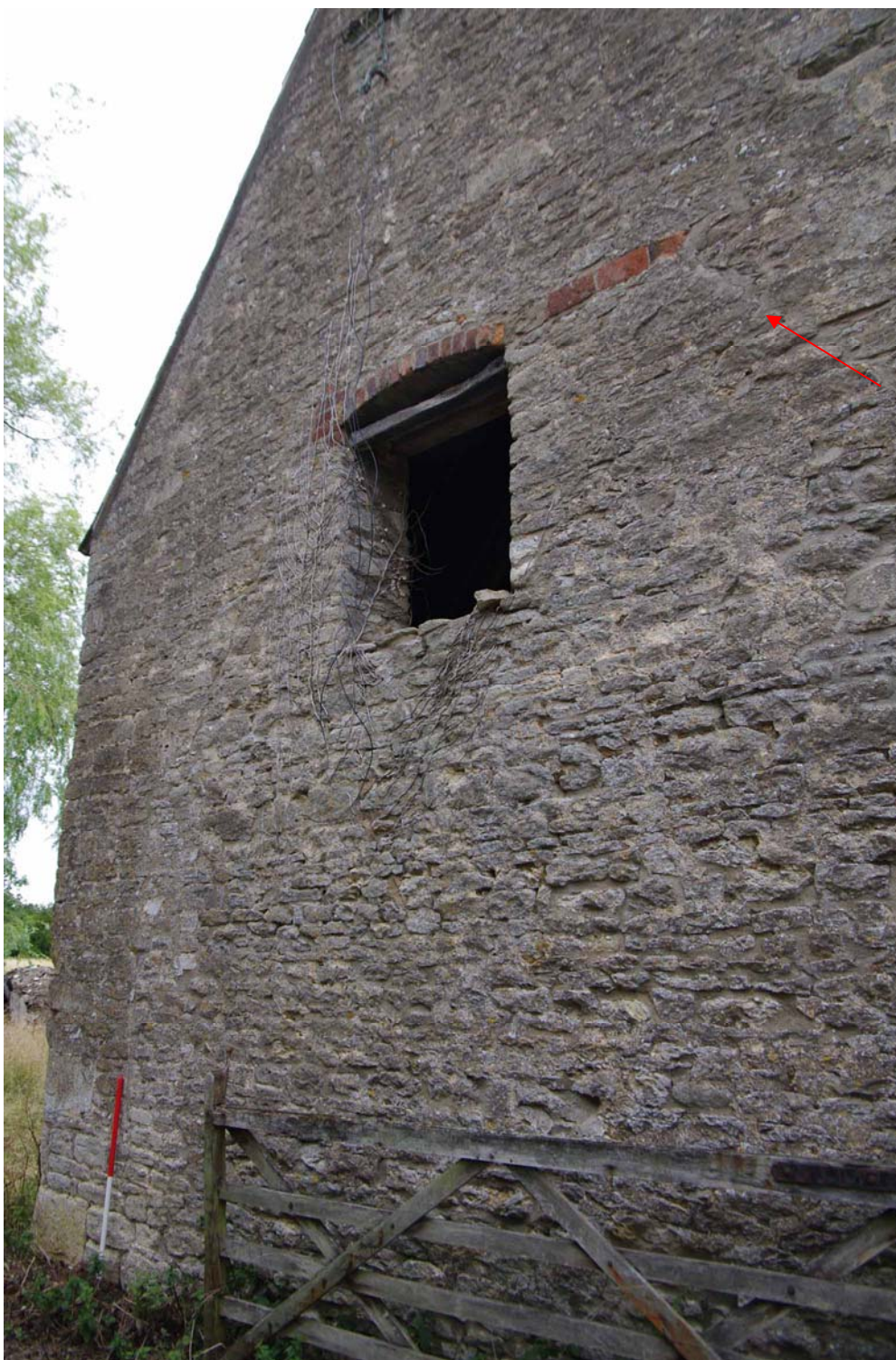
Figure 107: West range, south facing elevation of building A Looking north west. Note joint of earlier gable (arrowed), 1m scale marks the vertical joint of the earlier gable wall
