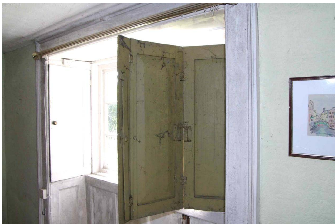
Figure 26: Ground floor, Room G2. Shutter detail Looking south-west. Note pivoting locking bar
