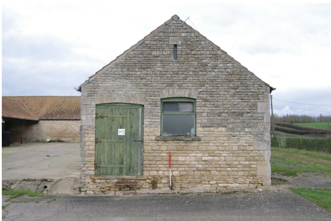
Figure 11 South facing gable end of eastern range Looking north. 1m scale. Note date stone above vent and scar left by removal of yard wall to the left of the door
