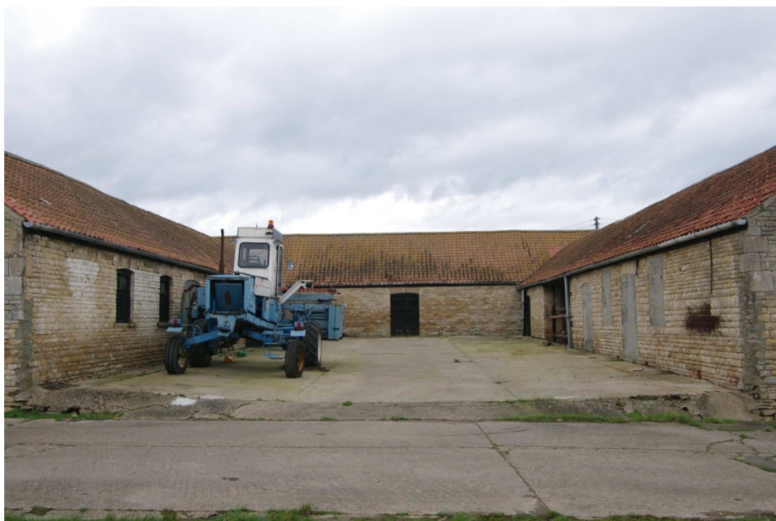
Figure 18 East yard Looking north. Note cut off yard wall stubs either side of the yard
