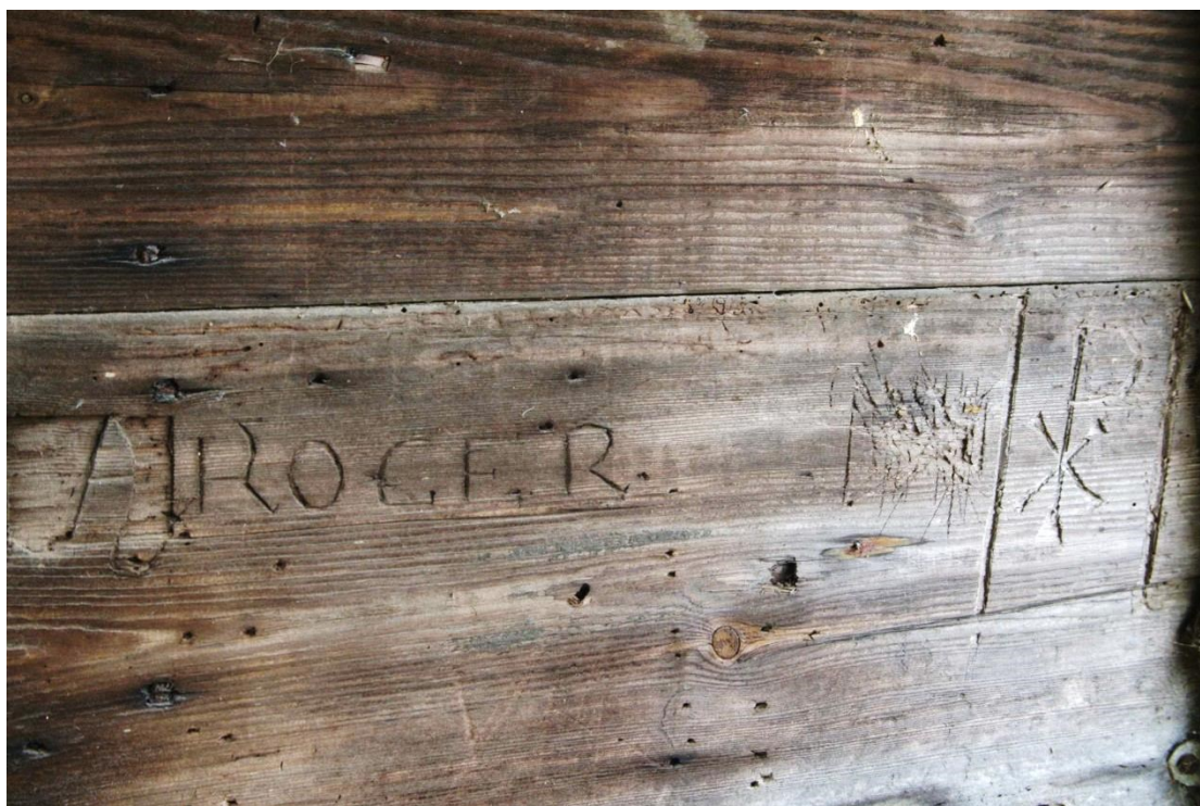
Figure 23 Graffiti on west partition wall of cart shed
