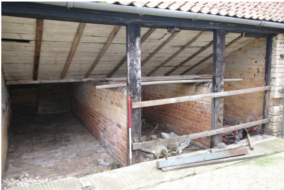
Figure 20 East yard, sties west facing elevation of east range Looking south-east. 1m scale
