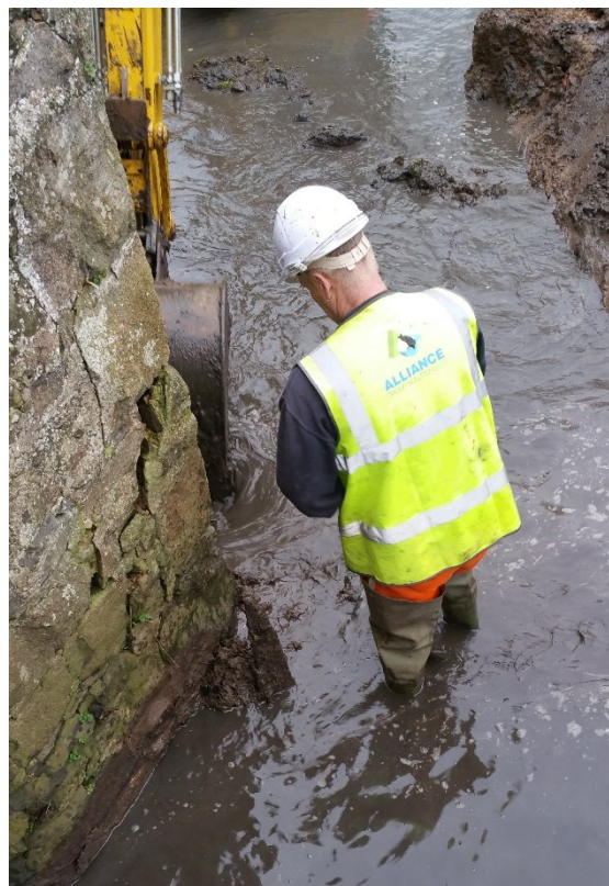
Figure 7: Hand clearance of river silt around Pier 1 with timber visible; view looking south-east
