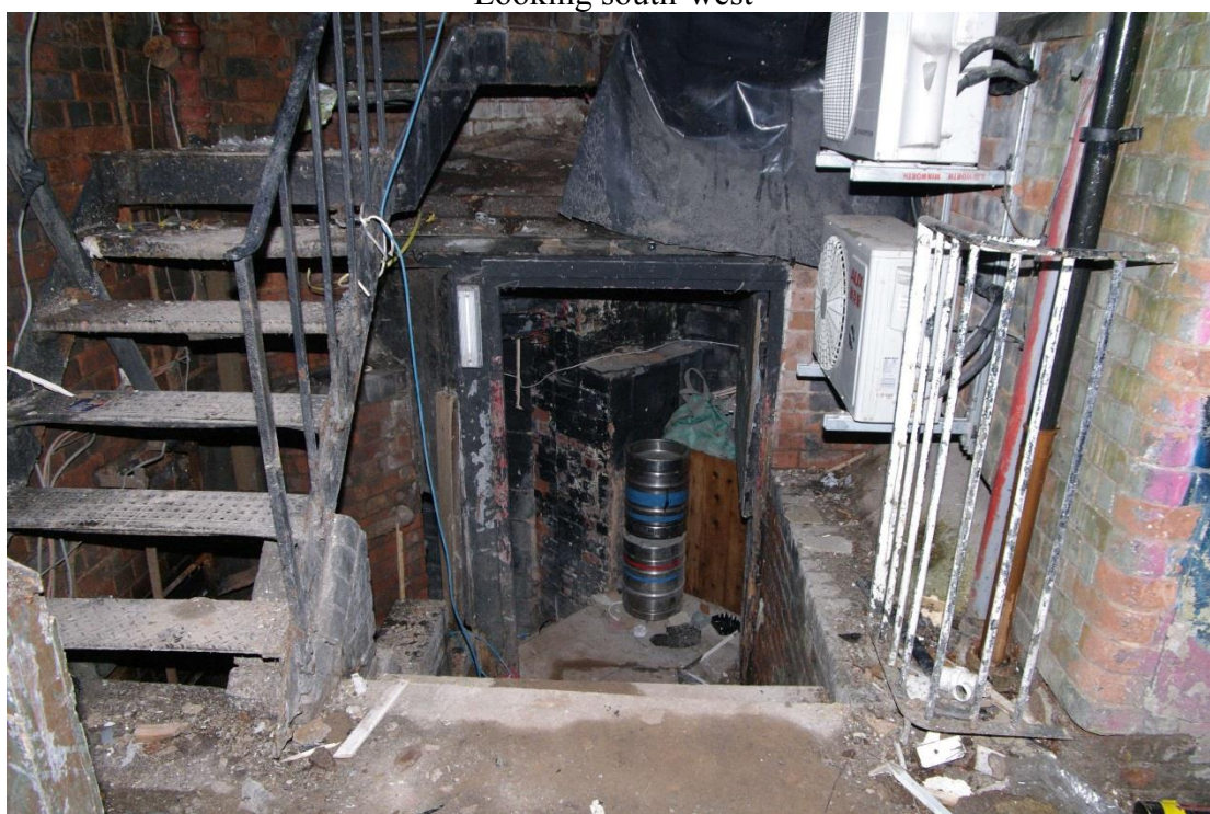
Figure 38 Basement steps from loading bay Looking west. The original steps were located slightly to the left of their present position and reached ground level where the fire escape is located
