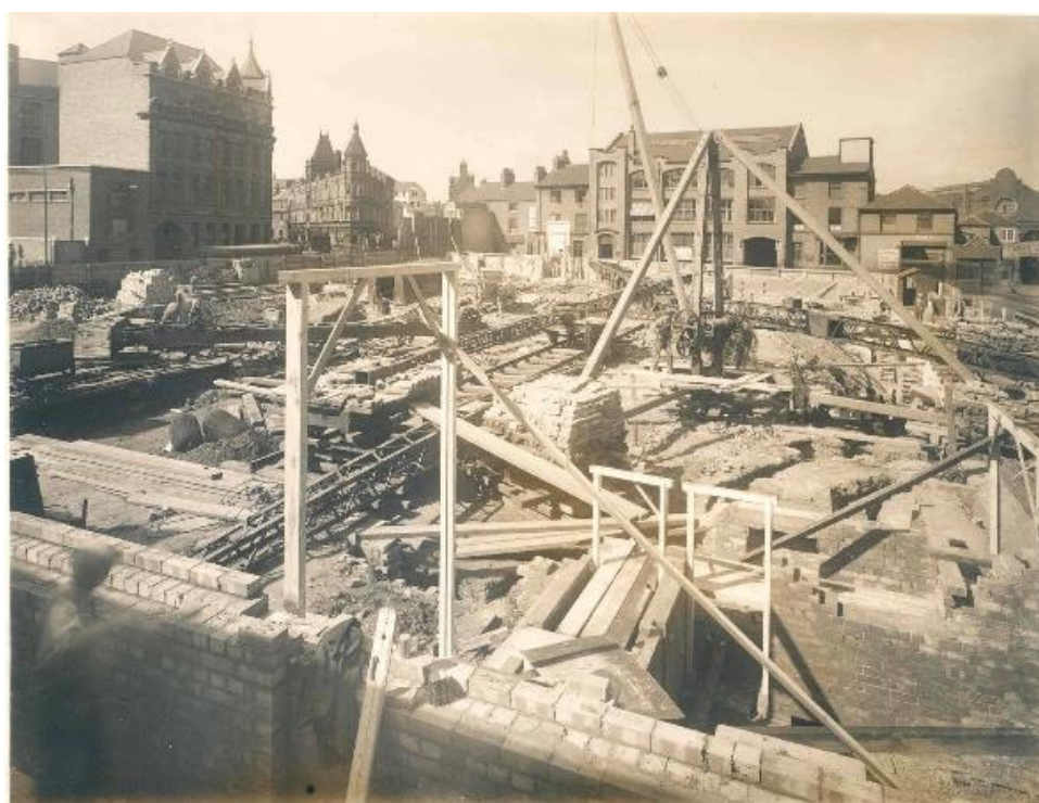
Queens Buildings in 1937 seen from the cinema (now Athena) construction site http://specialcollections.le.ac.uk/cdm/singleitem/collection/p16445coll8/id/84/rec/6
