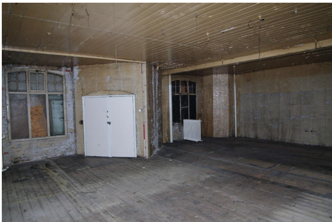
Figure 88 Third floor, rear range Looking south-east. 1m scale. Note boiler chimney breast in corner
