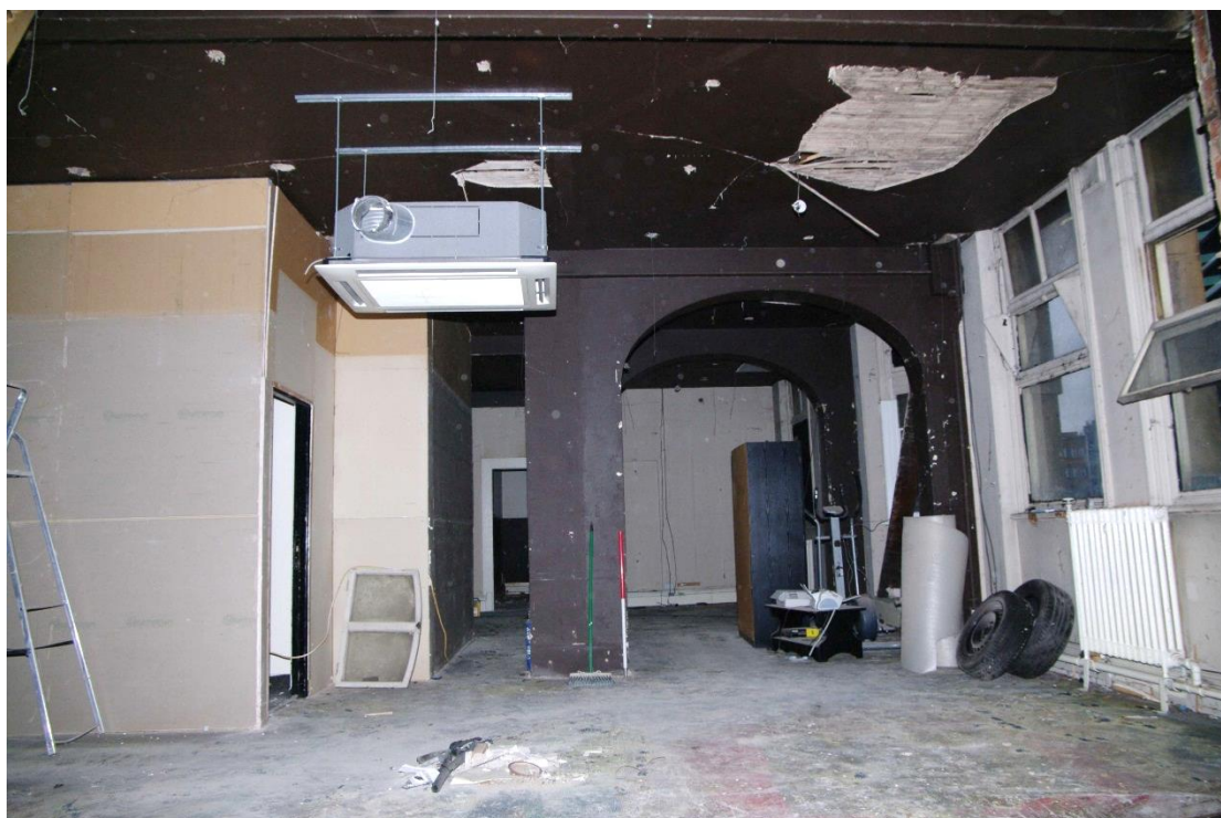
Figure 69 First floor, former office area Looking south-west. 1m scale. Boxed-in stairs on left. Masonry stub and arch of clerk's office centre right. Note modified windows on right
