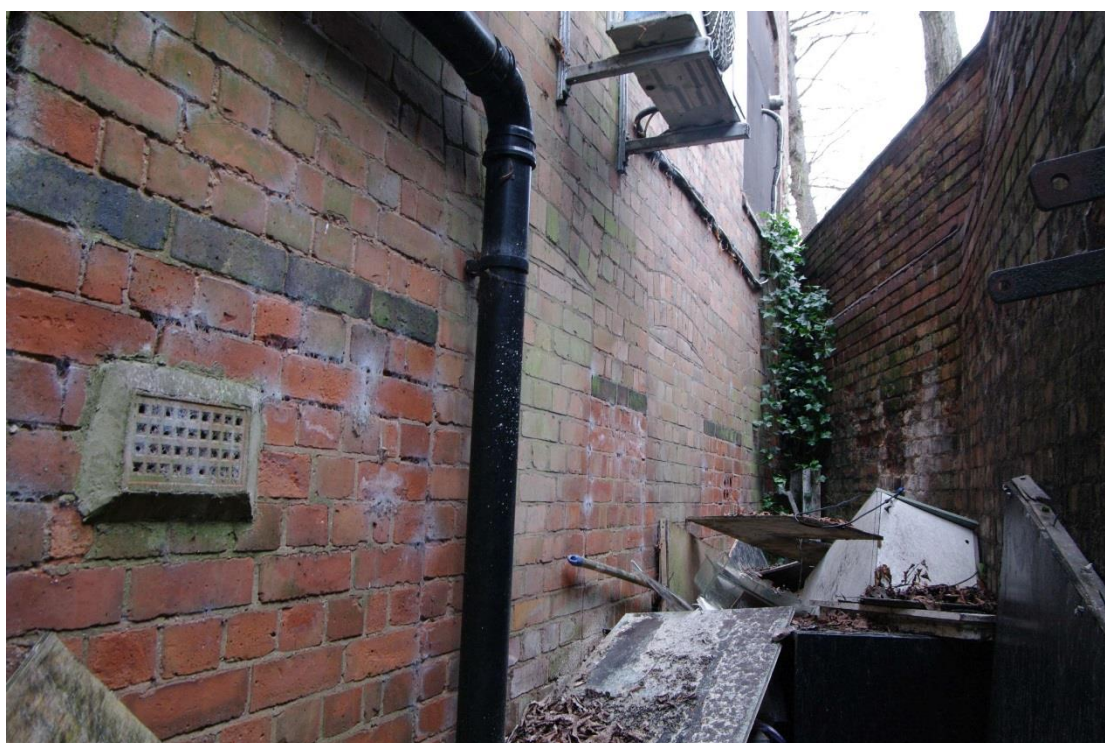
Figure 27 South-west facing elevation, blocked basement windows Looking south-east
