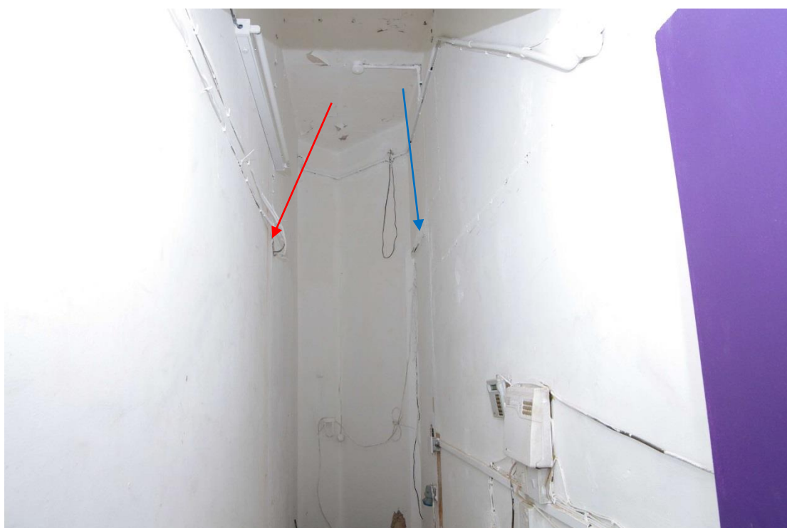
Figure 58 Ground floor rear corridor Taken from doorway shown in Fig. 57. Trace of blocked doorway into hair salon on left (red arrow), blocked doorway into warehouse of north-east facing warehouse on right (blue arrow)
