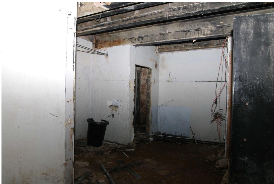
Figure 43 Basement, inserted rooms beneath north-east facing range Looking east towards the north-east corner of the basement. Note steelwork supports
