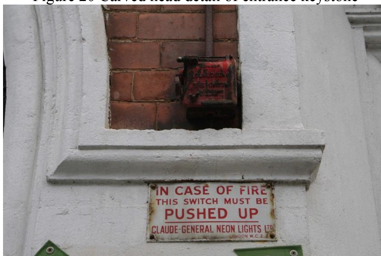
Figure 21 Electrical cut-off switch and plate near entrance
