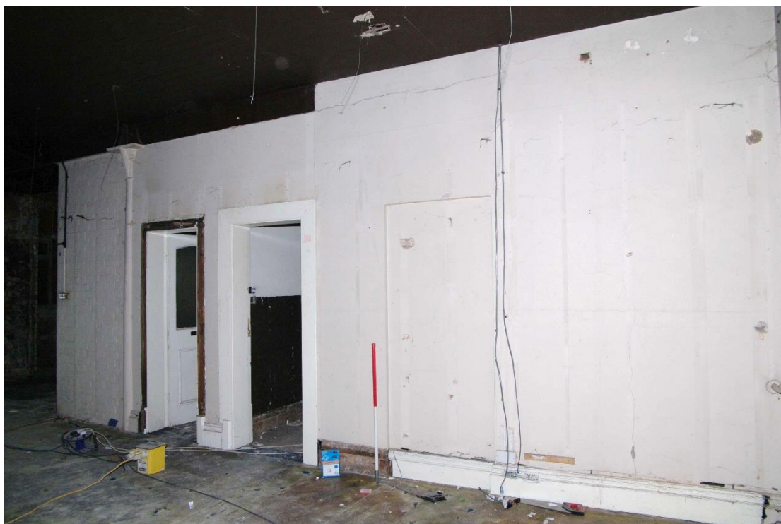
Figure 67 First floor, eastern wall of former reception room Looking south-west. 1m scale. Blocked doorway from reception to right of scale. Second doorway into reception room to left of scale. Original toilet door to left. Note metal column set into wall
