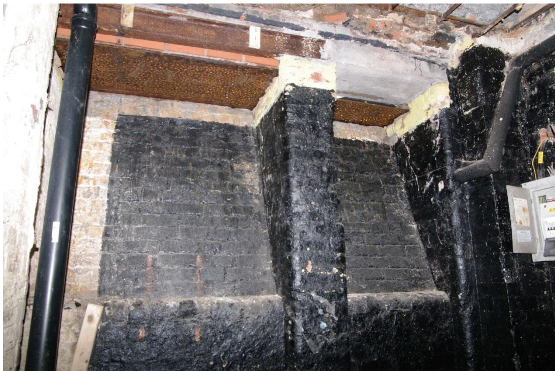
Figure 41 Basement, pavement vents or light wells beneath north-west facing range Looking north-west
