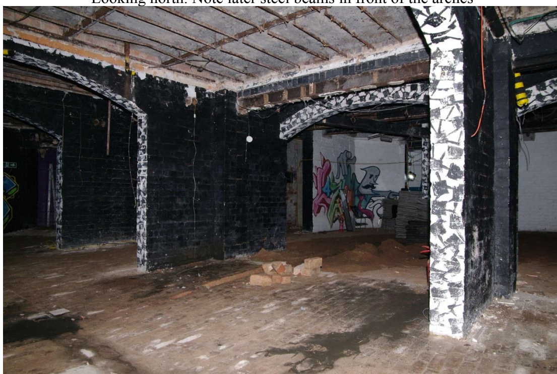
Figure 40 Basement, space beneath north-west facing range Looking west. Note original reinforced concrete ceiling and brick floor
