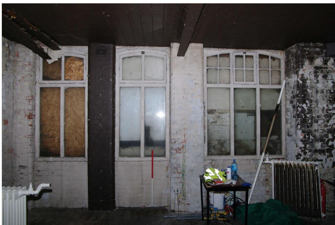
Figure 81 Second floor north-east facing range, south-west facing window detail Looking south-west. 1m scale
