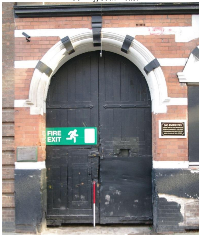
Figure 14 Gates into loading bay, NE facing elevation Looking south-east. 1m scale. Note bricked up basement window at ground level
