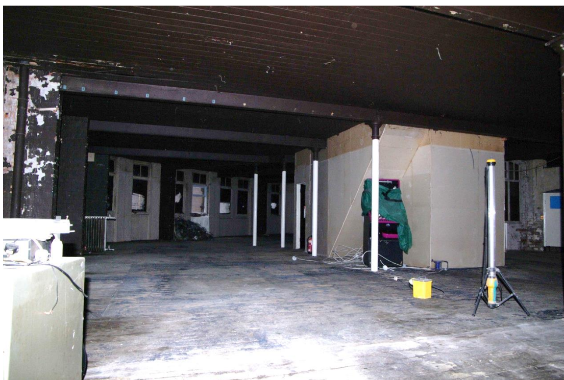
Figure 77 Second floor, general view and stairwell Looking east. Note original narrow stairs boxed in on left of stairwell
