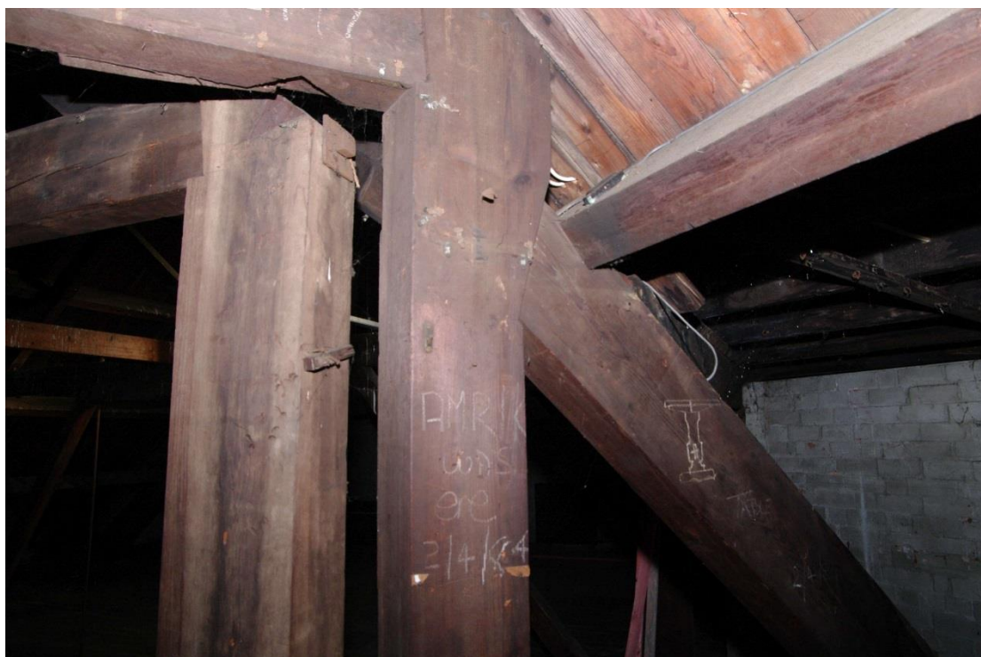
Figure 101 Fourth floor, graffiti Note drawing of pegged structure on right
