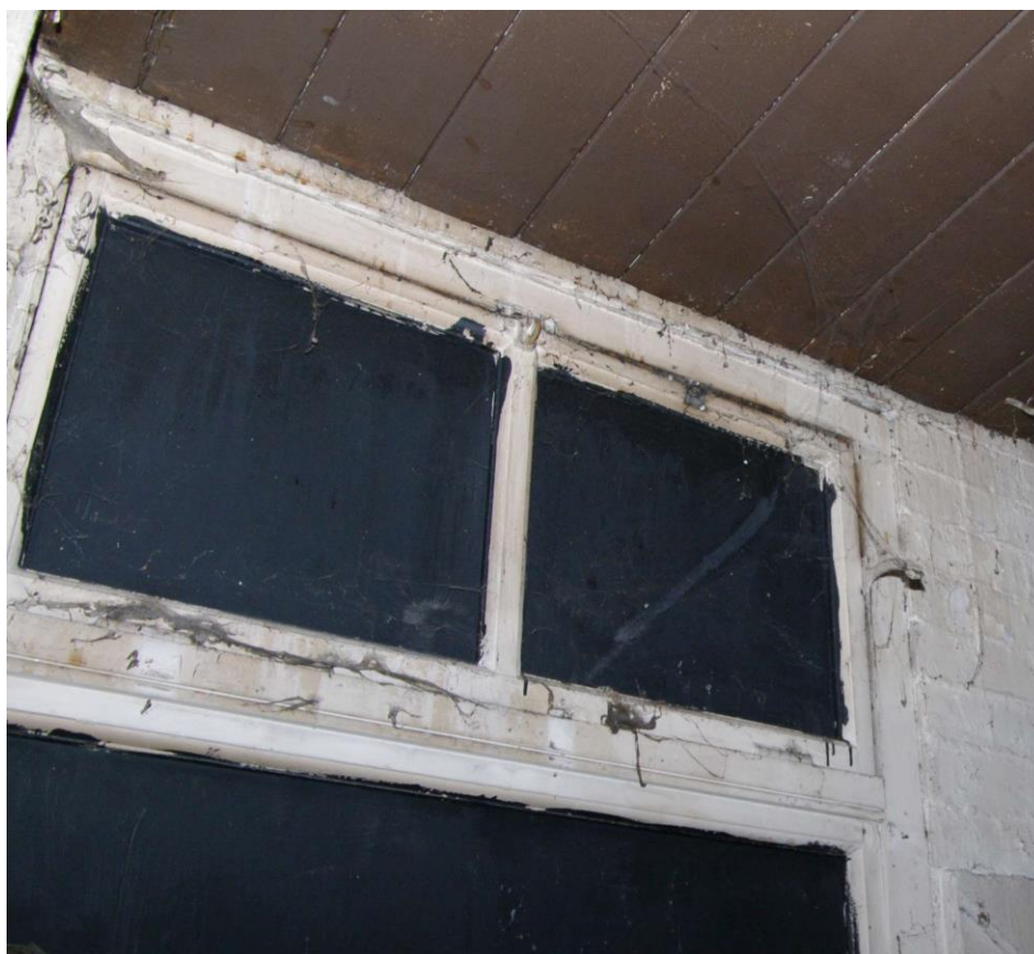
Figure 73 First floor window detail Upper opening panes, note securing chains (extreme left) and curving stops
