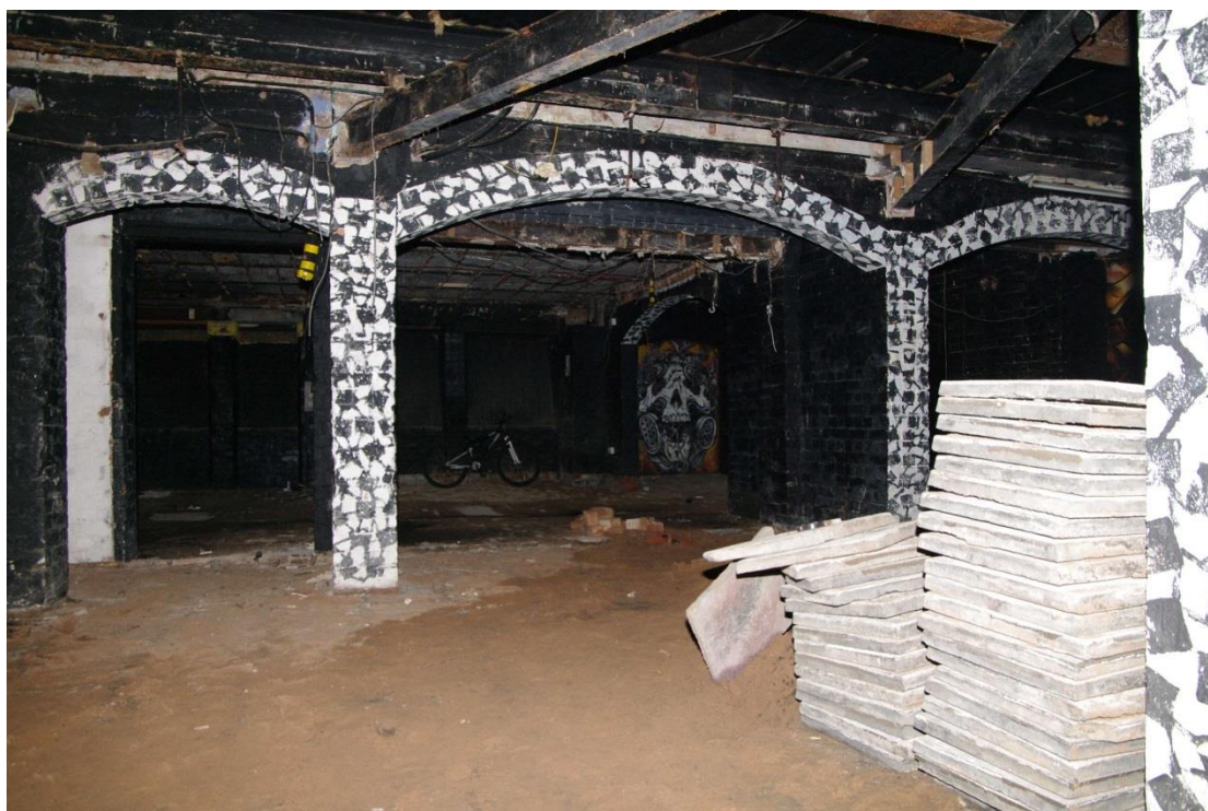
Figure 39 Basement, space beneath north-west facing range Looking north. Note later steel beams in front of the arches
