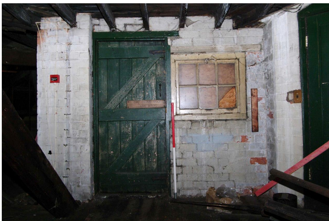
Figure 100 Fourth floor, fire escape door Looking east. 1m scale. Goods lift to right
