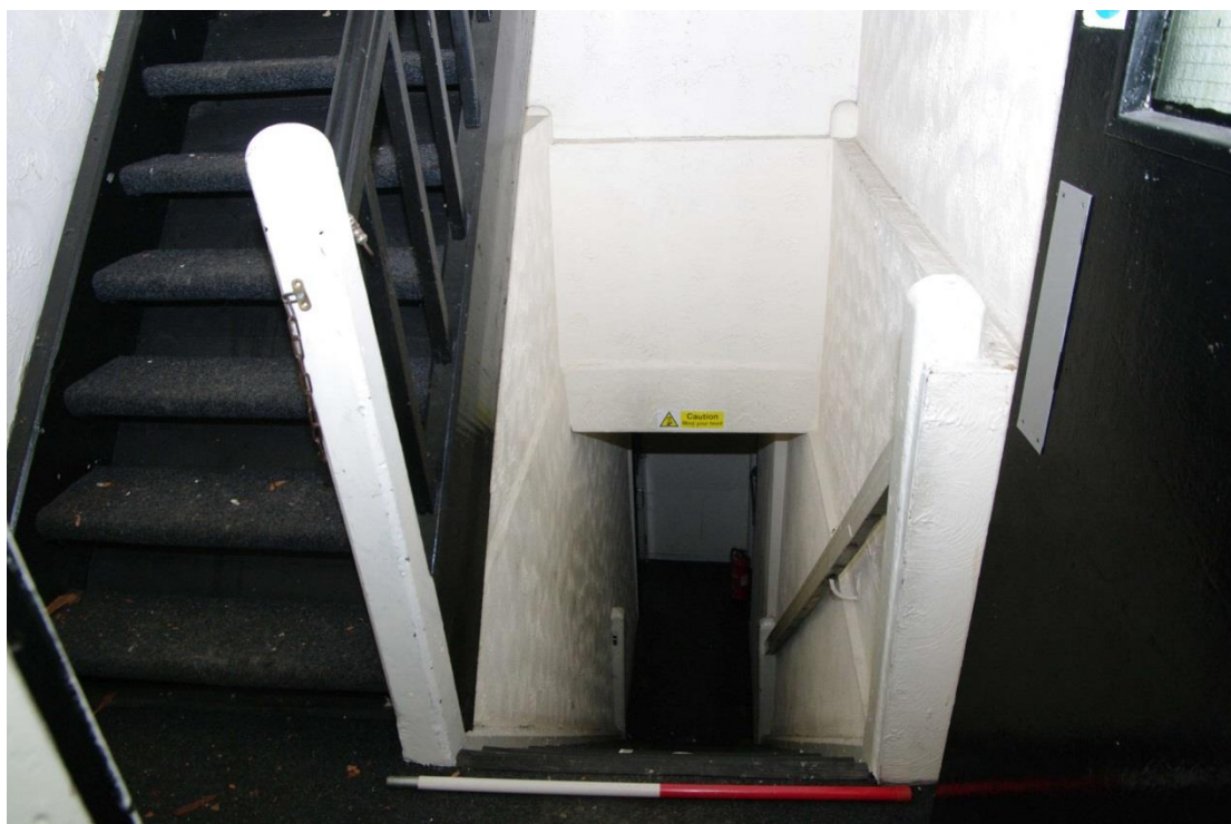
Figure 78 Stairs down to 2nd floor Looking north-east from 3rd floor landing. 1m scale. Stairs up to attic on left
