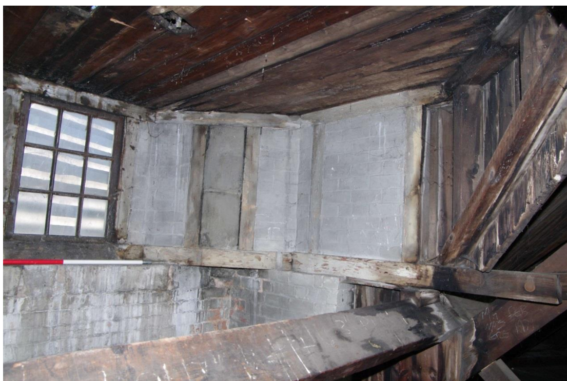
Figure 98 Fourth floor, base of tower Looking north-east. 1m scale. Note how octagonal tower sits on rectangular bay
