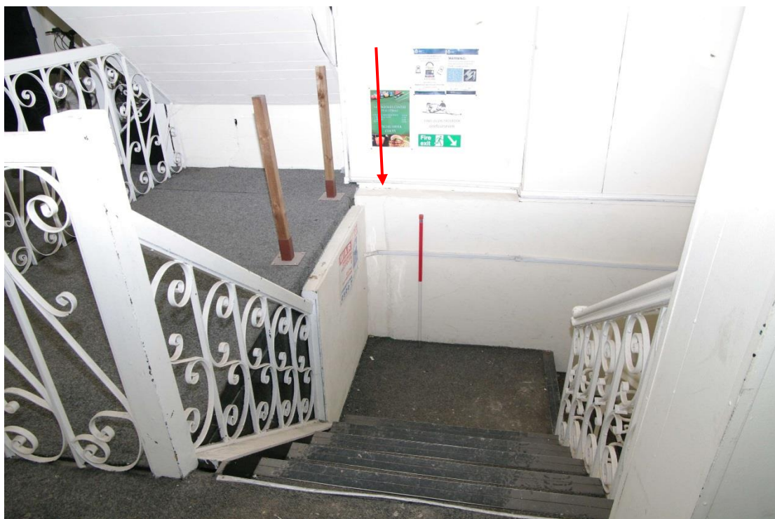
Figure 53 Stairs down to ground floor Looking south-west. 1m scale. Original width of stairs shown by scar on wall to left of scale (arrowed). Note original bannister on right, modern copy on left
