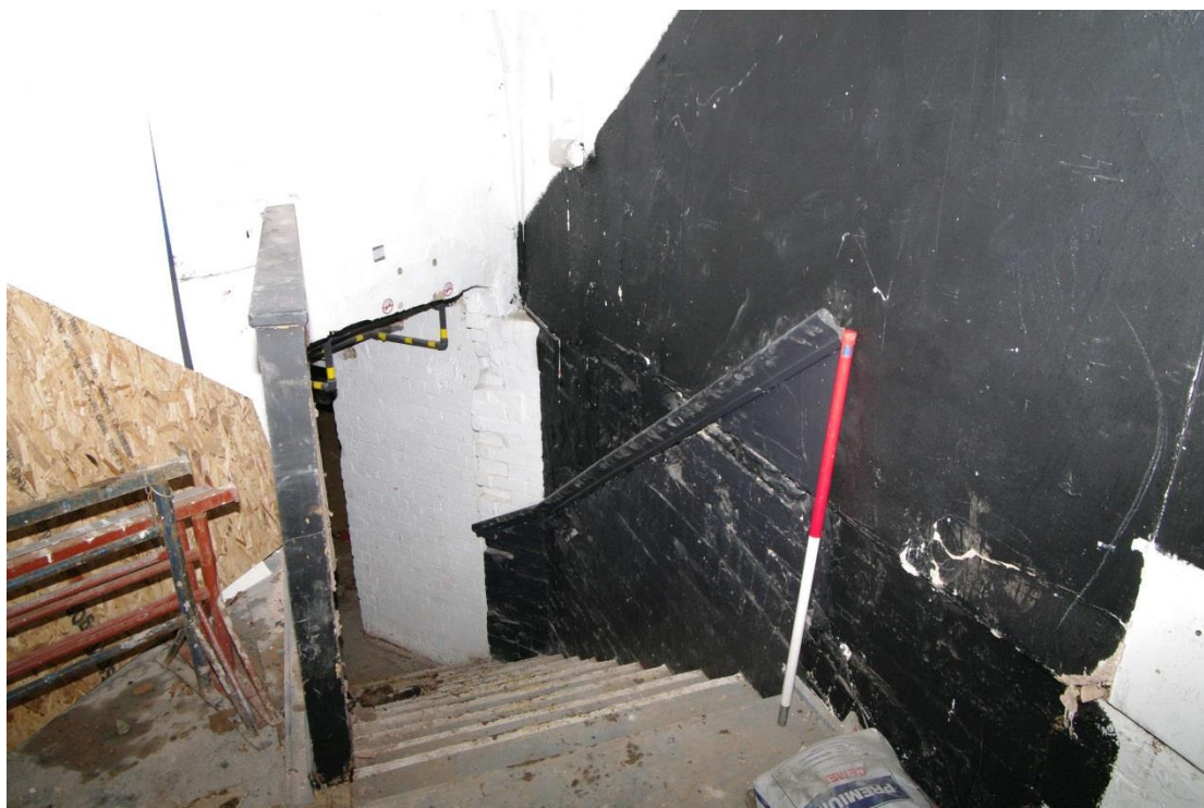
Figure 55 Ground floor, stairs to basement from corner room Looking south-east. 1m scale. Original stairs ran from where the metal trestles are standing. See also Figure 42
