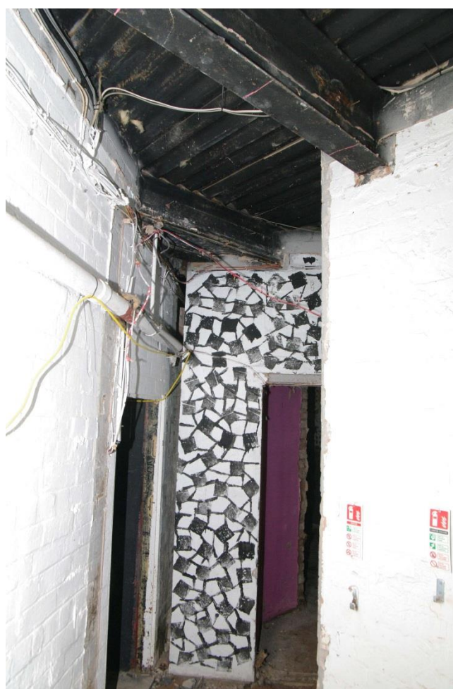
Figure 36 Basement rear range, inserted walls Looking south-west. Lift shaft door on right
