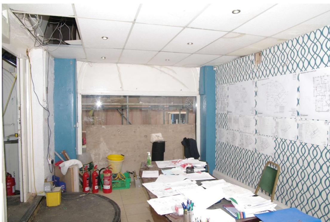
Figure 54 Ground floor, former hair salon Looking north-west. Modern doorway to entrance hall on left
