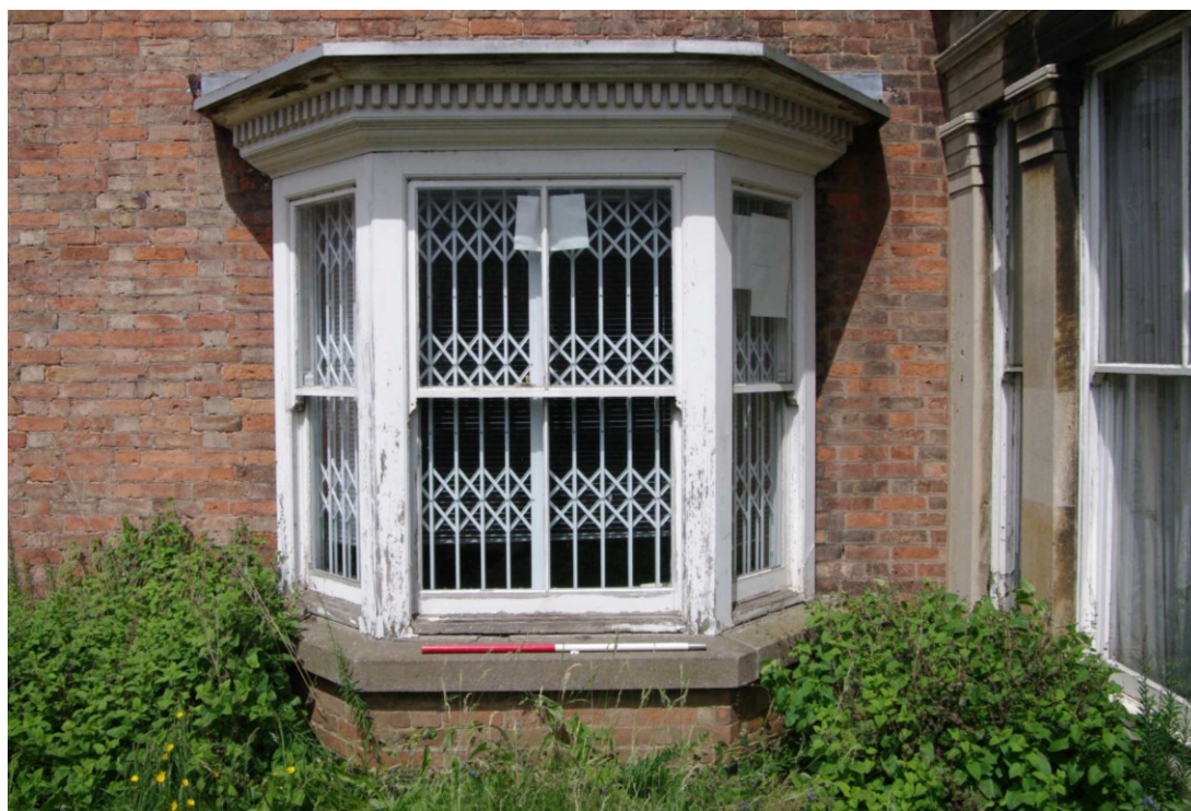
Figure 23 South-east facing elevation of rear south-east wing ground floor window Looking north-west. 1m scale
