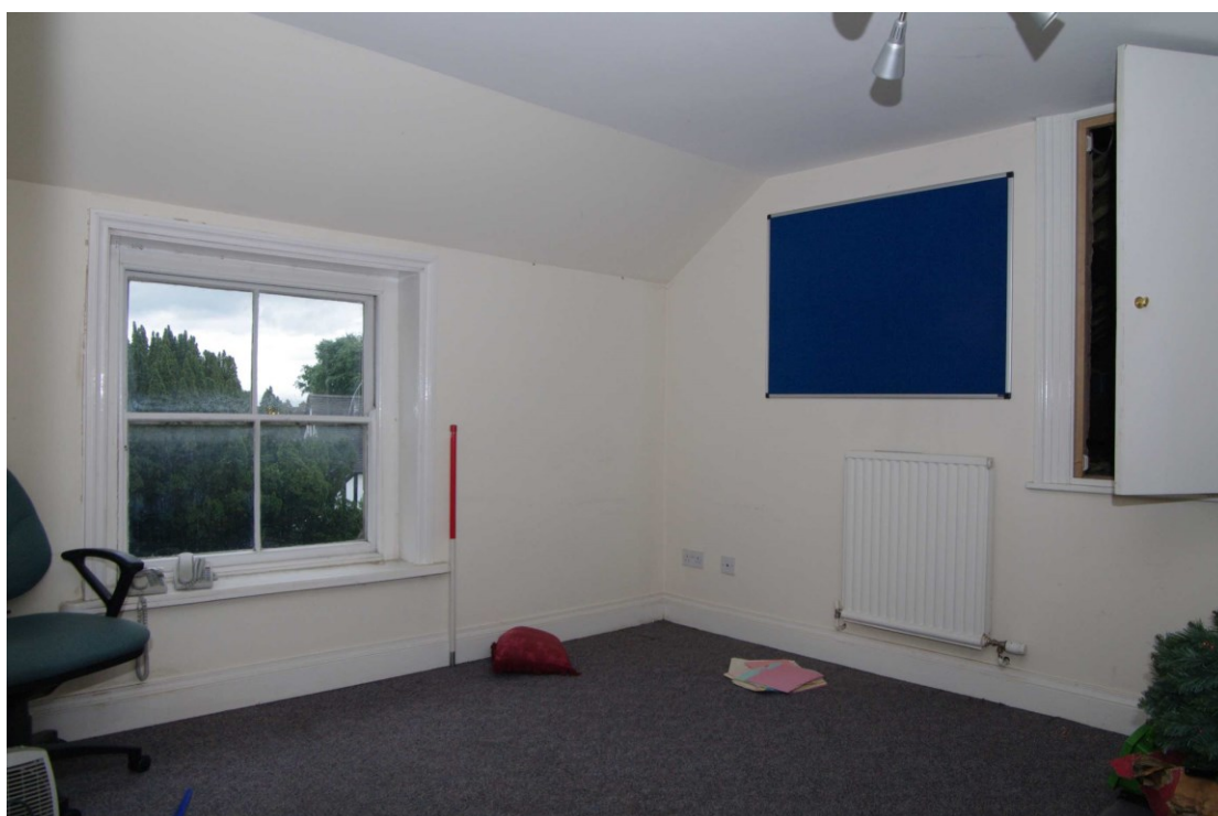
Figure 75 Room S2 Looking east. 1m scale. Hatch into Room S3 on right of picture
