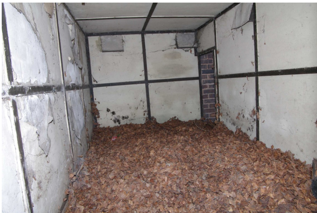
Figure 103 Inside air raid shelter Room OB8 Looking south-east from NW doorway towards SW doorway
