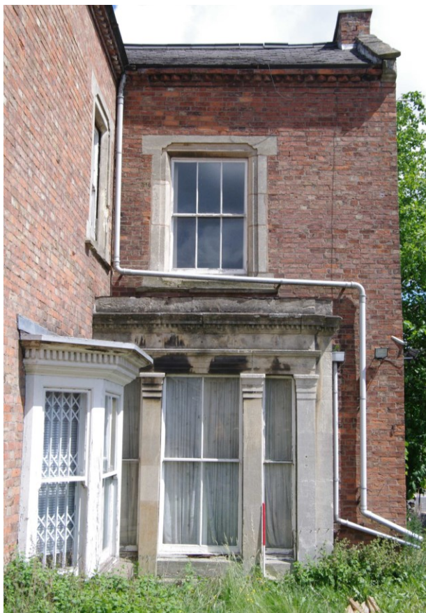
Figure 26 South-west facing elevation of main house: eastern end Looking north-east. 1m scale
