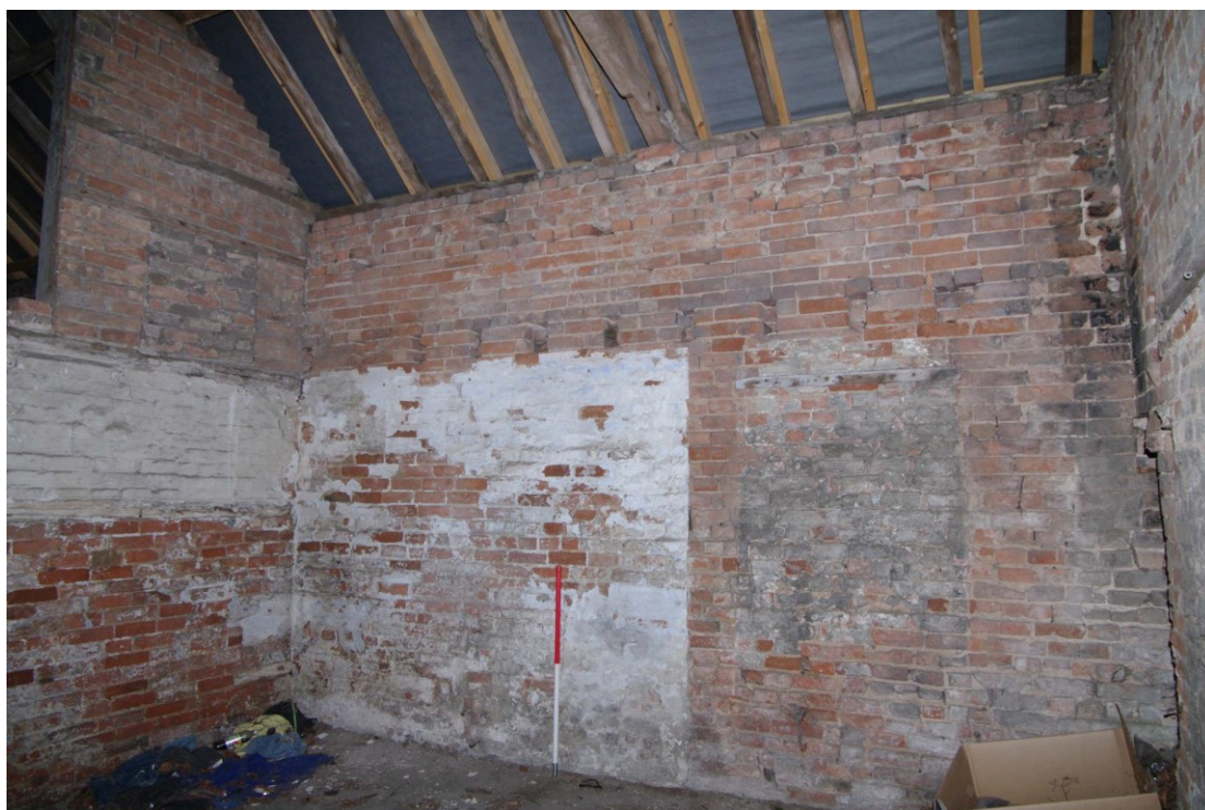
Figure 97 Outbuilding OB4 Looking east towards wall with OB3. 1m scale Note empty first floor joist sockets
