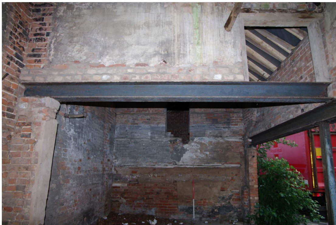
Figure 96 Outbuilding Room OB3 from OB2 Looking south-west. 1m scale. Note first floor doorway and blocked hatches. Also wooden bracket on left for hanging saddles or tack
