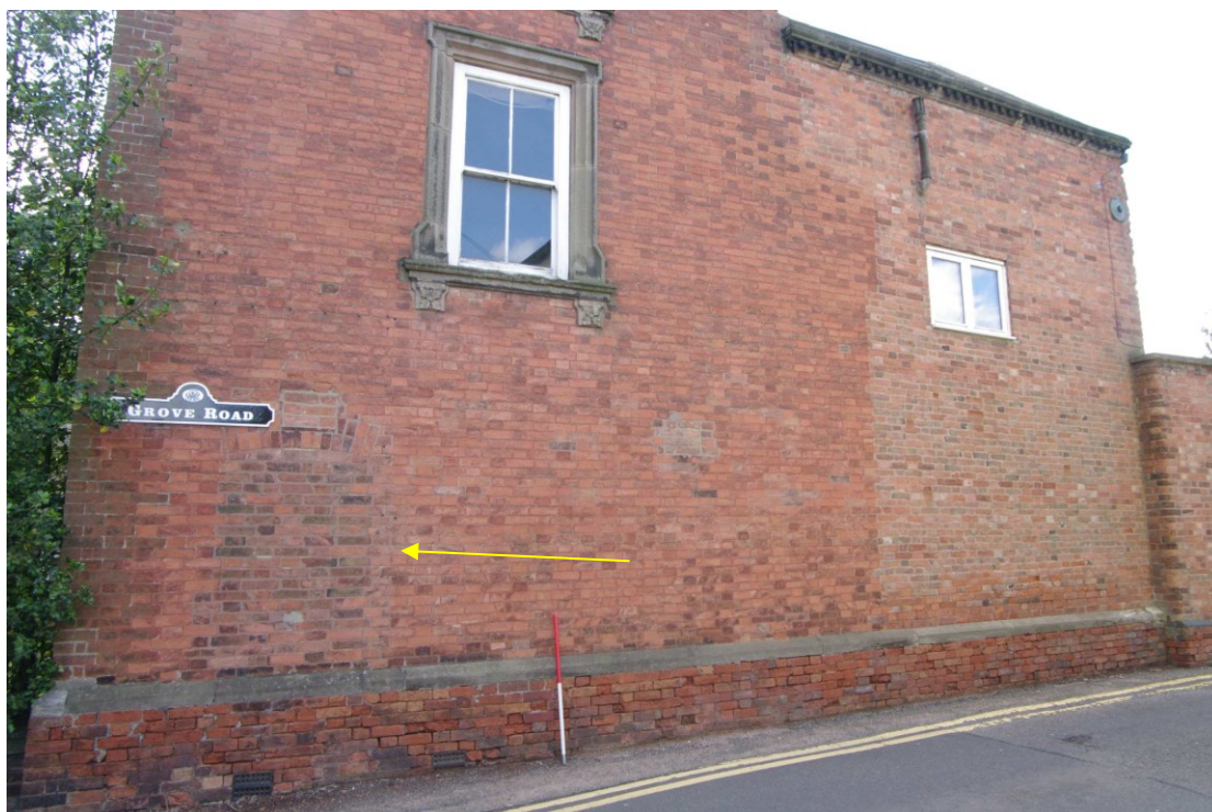
Figure 19 North-west facing elevation, ground floor blocked window Blocked window arrowed. Note repointed bricks and modern window on right of picture. Looking south-east. 1m scale
