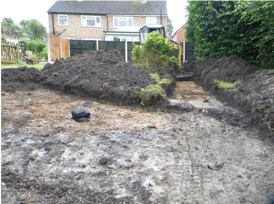
Figure 4: Excavation of area showing natural and modern deposits. Looking South (waste pipe diagonally across site)
