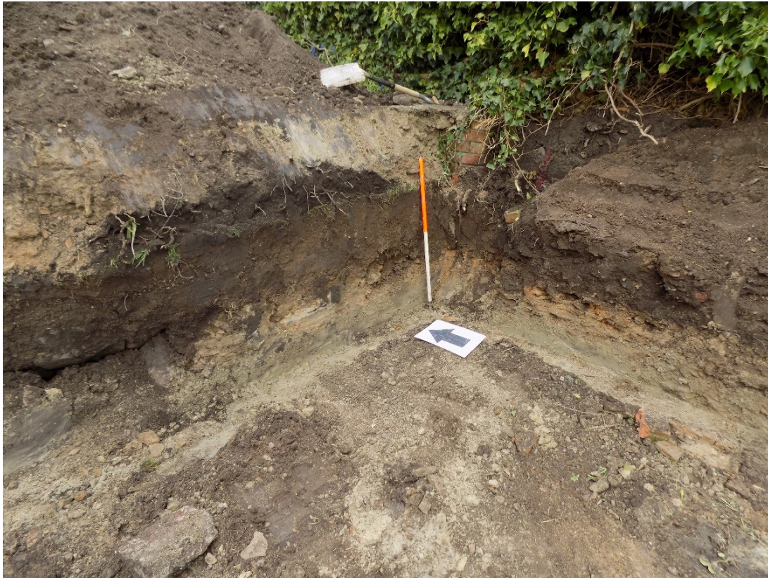
Figure 9: View looking north-east showing the foundation trench for the proposed retaining wall for the driveway.
