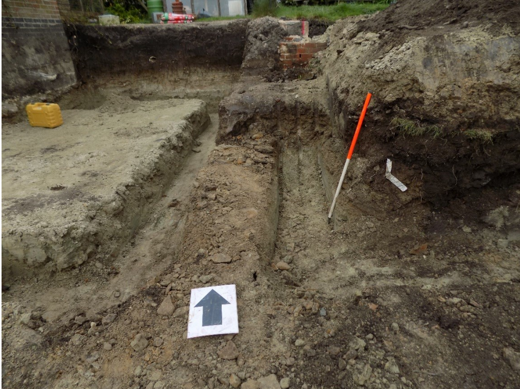
Figure 8: View looking north showing the foundation trench for the new retaining wall which will surround the new driveway and to the east of the proposed garage.
