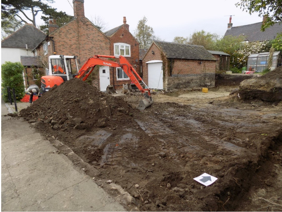
Figure 11: View post-excitation waiting for excess soil to be removed in preparation for the arrival of the ready made concrete.
