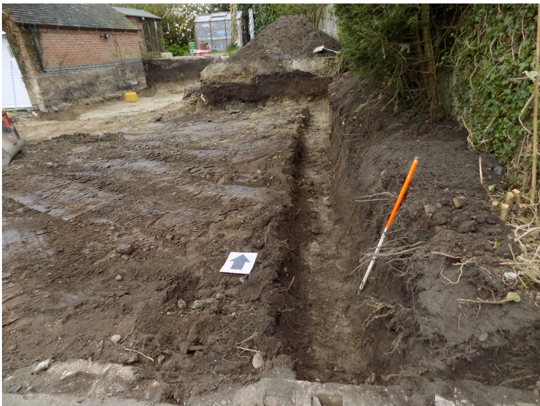
Figure 10: View looking north along the easternmost boundary of the development showing the foundation trench for the retaining wall surrounding the driveway.
