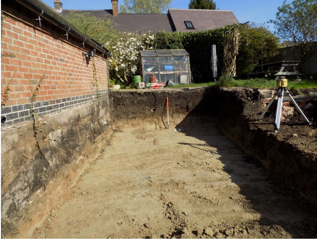
Figure 4: Prepared area of land for the garage extension to the east of the existing garage, looking north. The view shows the stripped area prior to the foundation trenches being dug. Land drains are visible in section.
