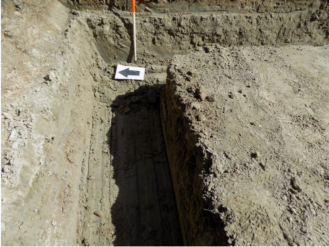
Figure 5: View looking east, showing north-eastern area of the foundation trench for the garage extension.
