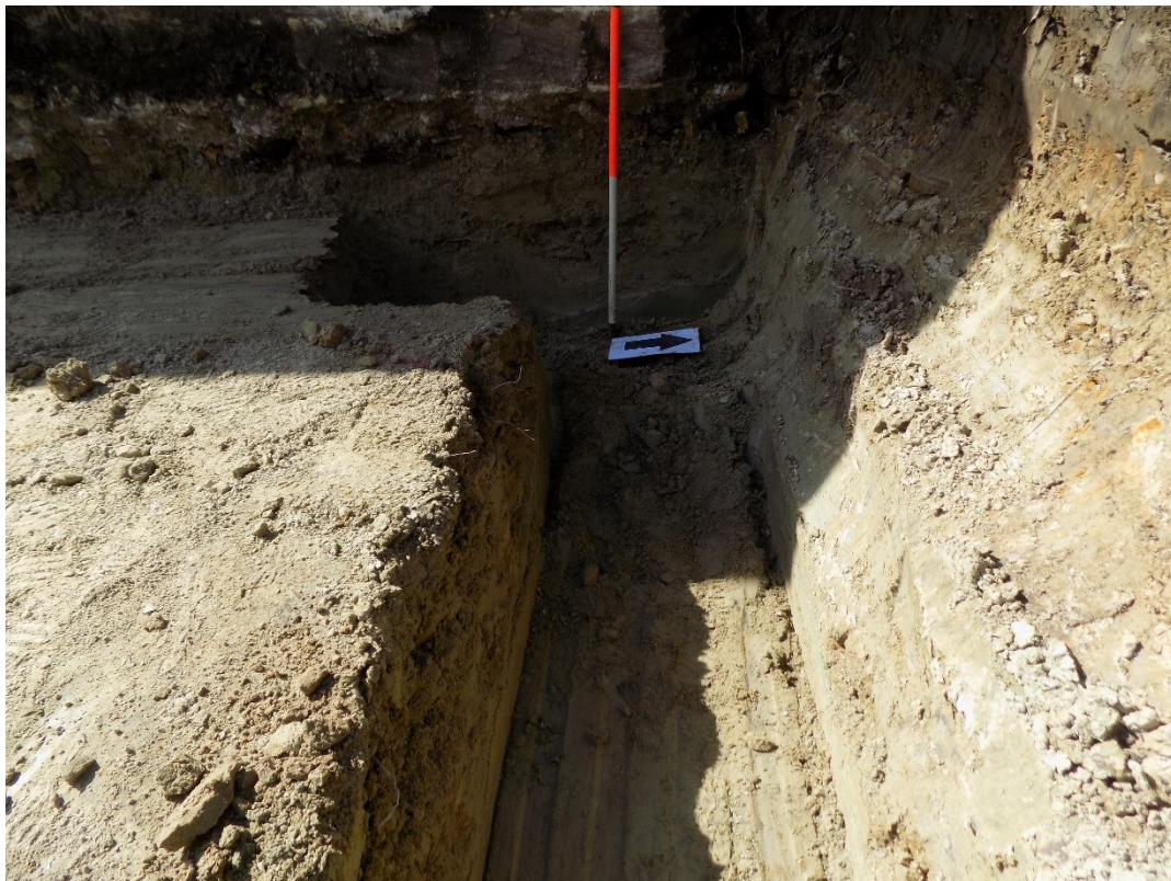
Figure 6: View looking west, showing north-western area of the foundation trench for the garage extension.
