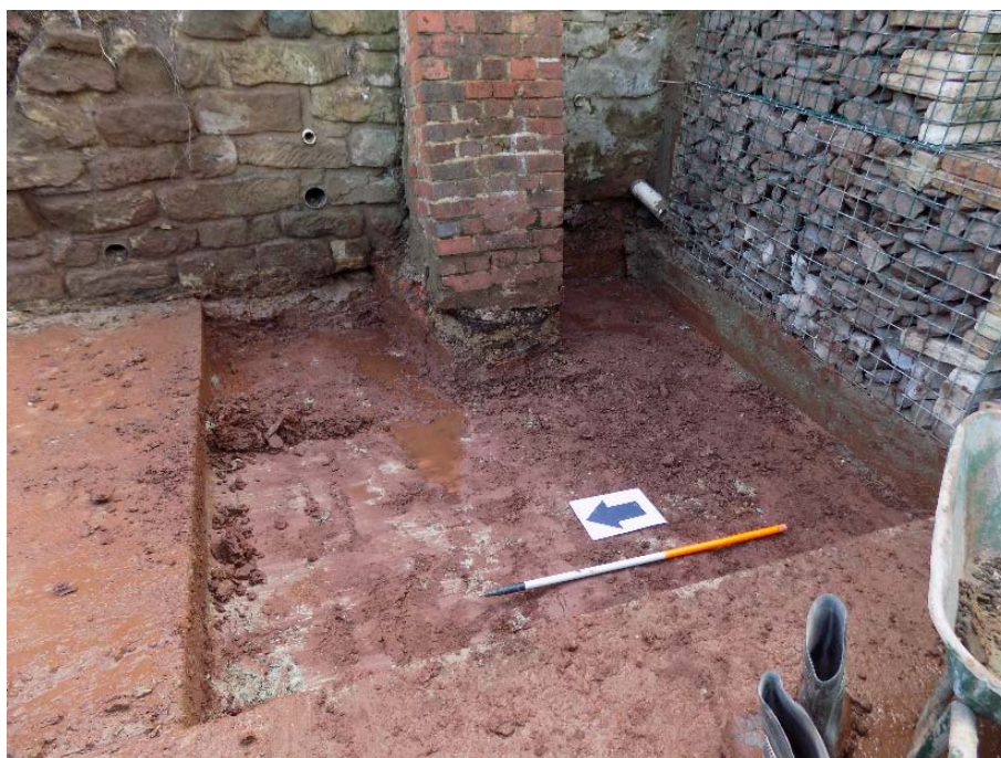
Figure 20: Excavated footing ready for the concrete base for the retaining gabions. Photograph shows that the footings are dug directly onto the natural substratum of sticky red clay.
