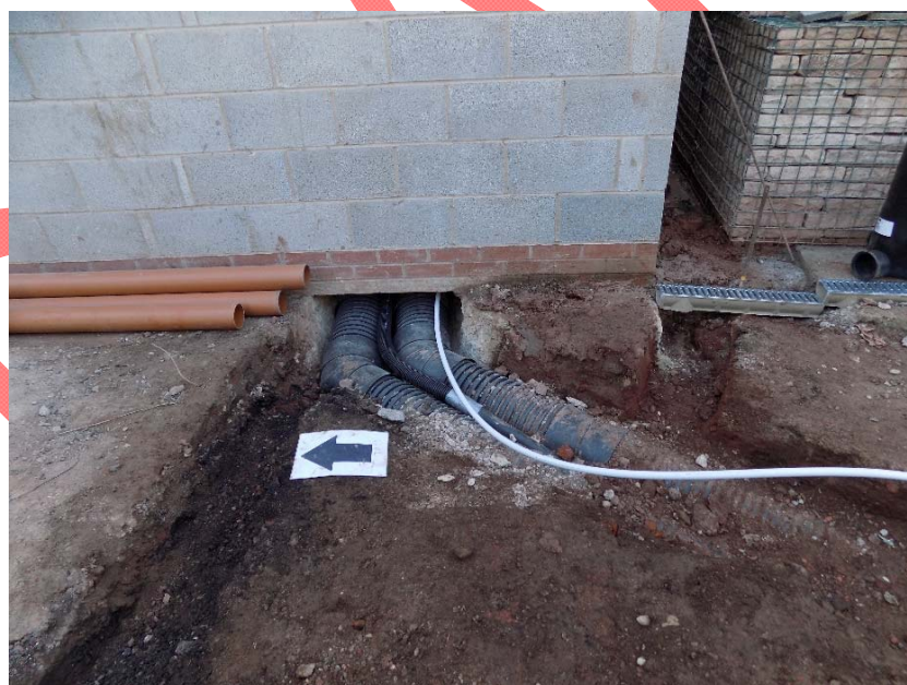
Figure 15: Excavated ground for refrigeration and drainage pipes on the western side of the new cellar building.
