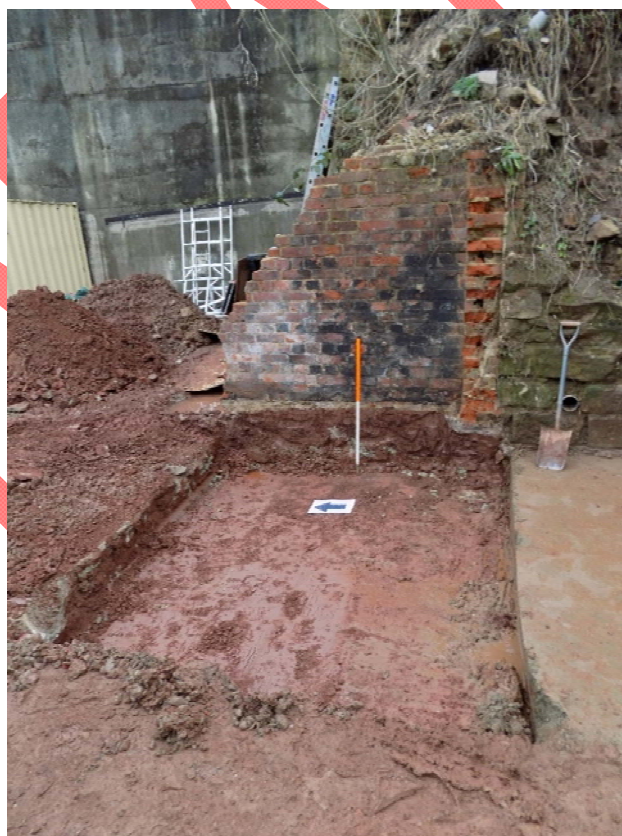
Figure 21: Area excavated ready for the concrete footing for the retaining gabion. Photograph also shows brick wall to be removed and replaced by retaining gabion.
