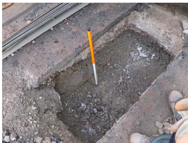
Figure 6: Photograph showing part of the western most foundation trench for the new cellar building. Note the pre-disturbed, truncated modern stratigraphy.
