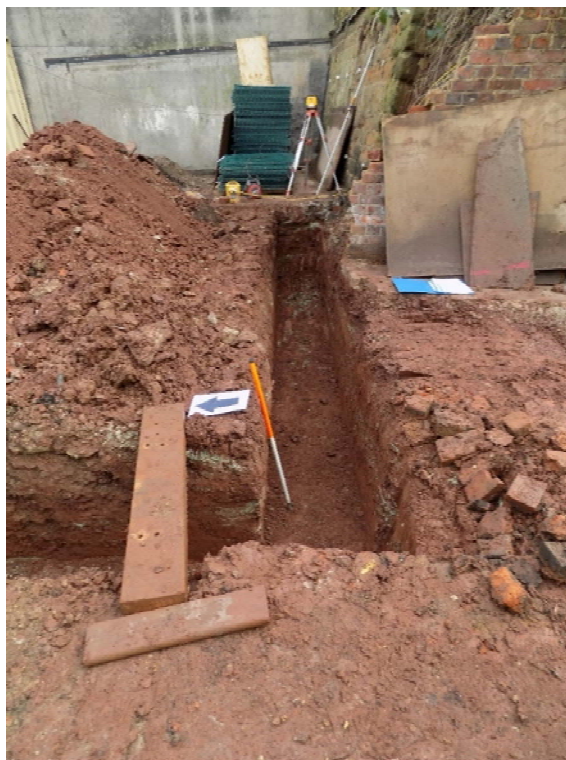
Figure 11: South western corner of the foundation trench for the proposed cellar building. Brick path / surface visible at the right side of the photograph, placed directly onto the red natural clay.
