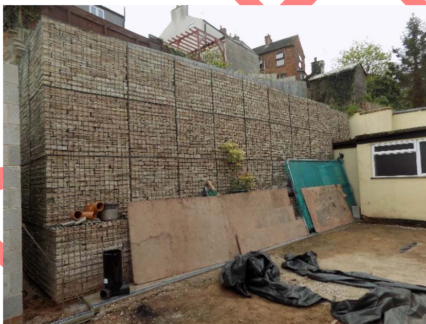
Figure 25: Photograph showing the newly constructed retaining wall of gabions to hold back the bank.
