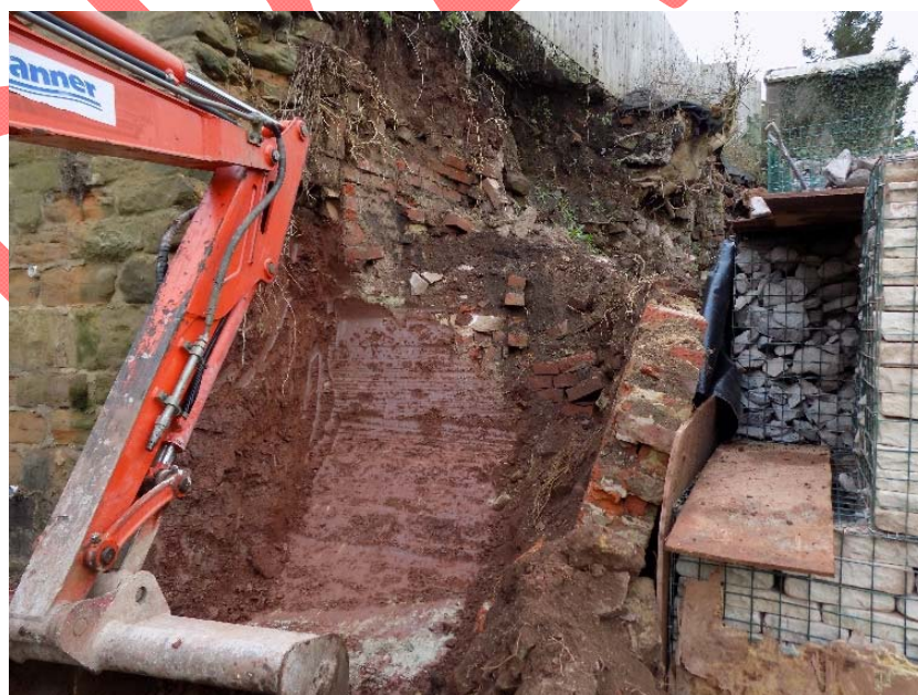
Figure 23: Photograph showing removal of bank and existing retaining brick wall in advance of the construction of retaining gabions.
