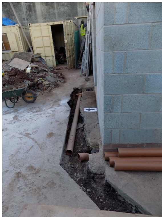
Figure 14: Excavated ground for drainage next to the new cellar building at the northernmost point looking east.
