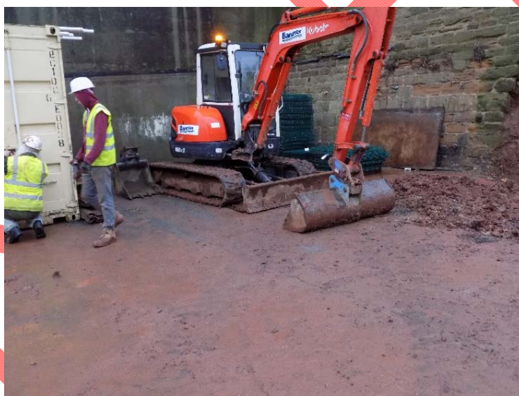
Figure 5: Photograph looking south west at the area for the construction of the cellar. Retaining walls for the bank are visible in the background.
