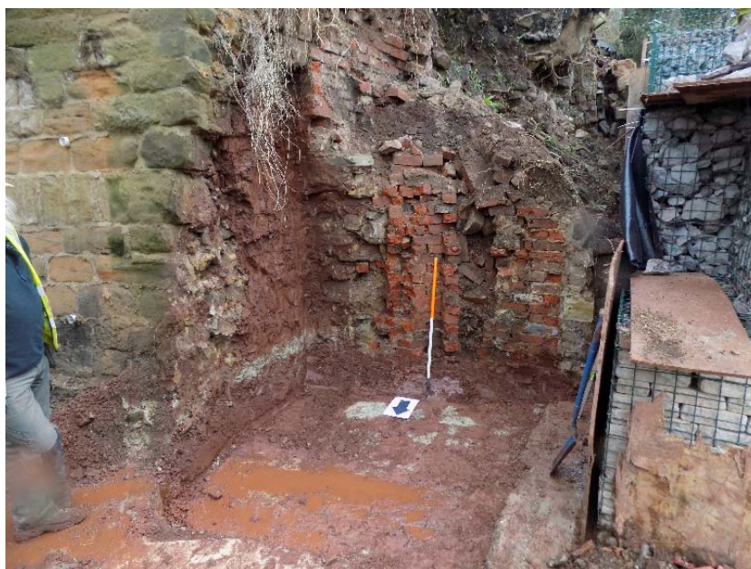
Figure 24: Photograph showing the area of the bank which has been removed, and also the remains of existing buttresses and stable block which had become enveloped by the bank.
