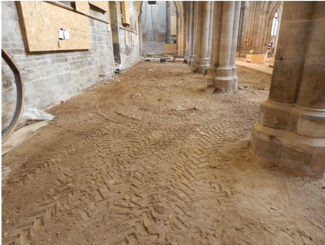
Figure 6: The north aisle after the reduction and compaction of the soils, looking east
