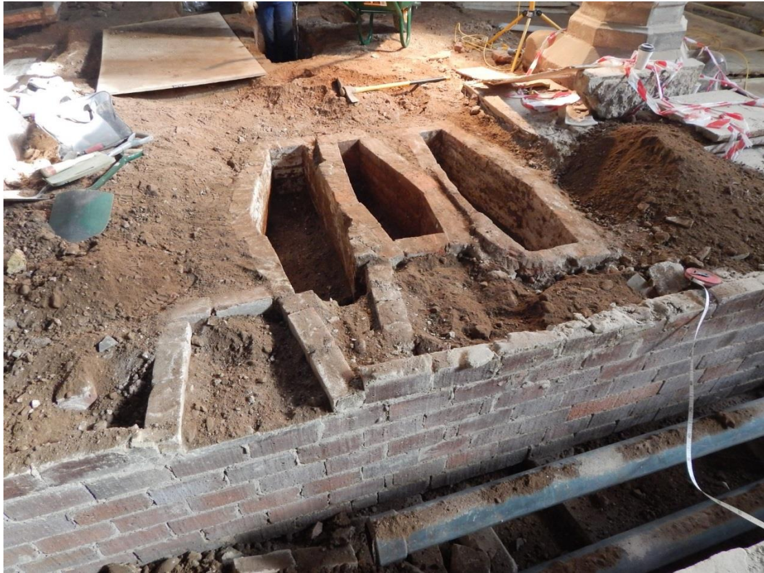
Figure 35: Three small graves at western end of north transept (Graves 36-38), with damaged graves and heating system, looking south-east
