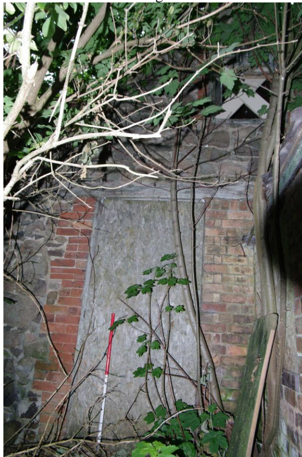
Figure 15 Gable end wall of western brick built structure Looking north. 1m scale. Note former double doorway reduced to single doorway by later brickwork. Hayloft door top right
