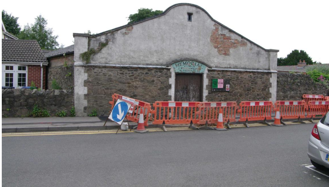
Figure 11 North and west facing elevations Looking south-east. Note the brick courses on the north wall
