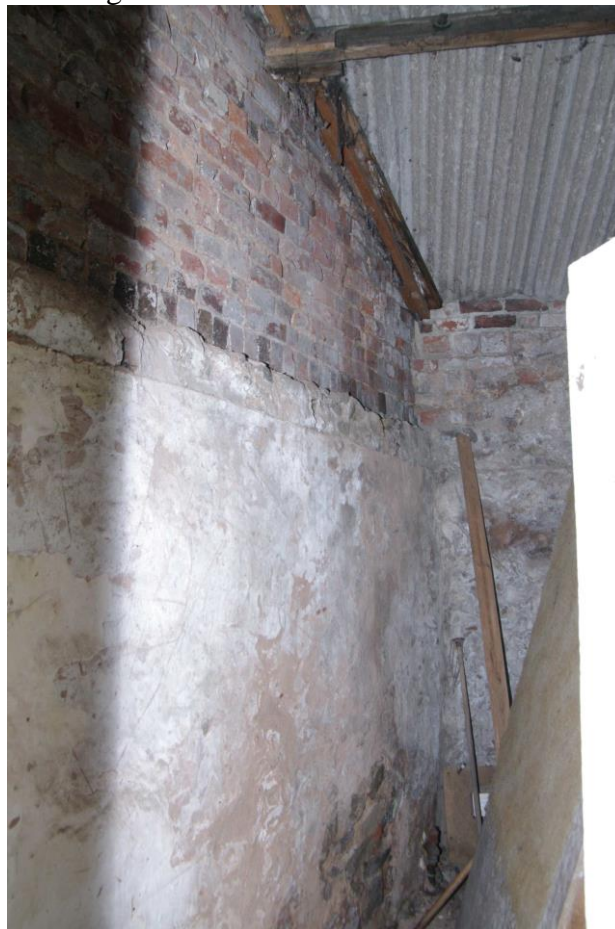
Figure 20 Cloakroom attendant's room Looking north through door from vestibule. Note pitched stone copings on outside wall beneath brickwork
