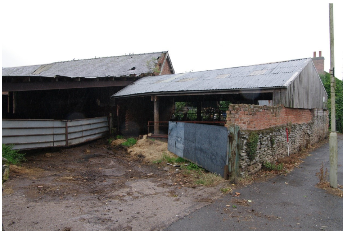
Figure 42: Open barn to west of Barn B, west and north facing elevations Looking south-east from Lady Gate. 1m scale. Barn B on left
