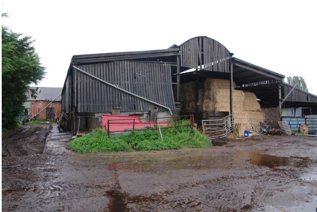
Figure 7: Post Great War barn Looking north. Barn B in distance to left
