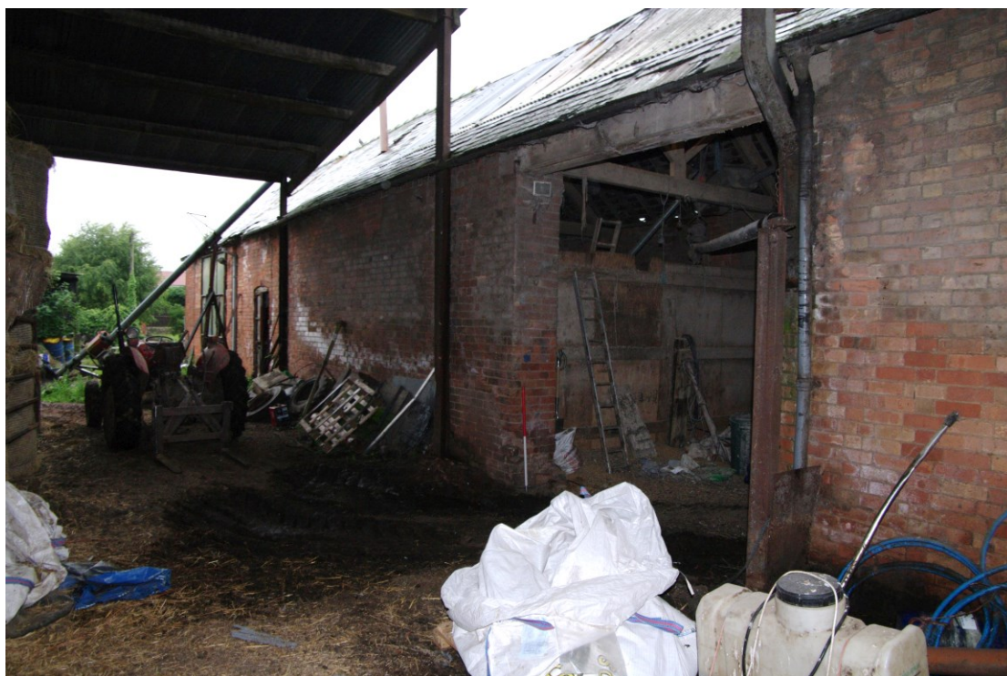
Figure 29: Barn B, south facing elevation (centre portion and threshing doors) Looking north-west. 1m scale
