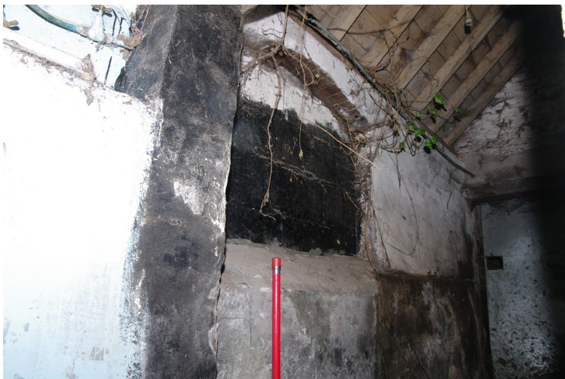
Figure 23: Barn A, blocked window on north wall in silo room Looking north-east
