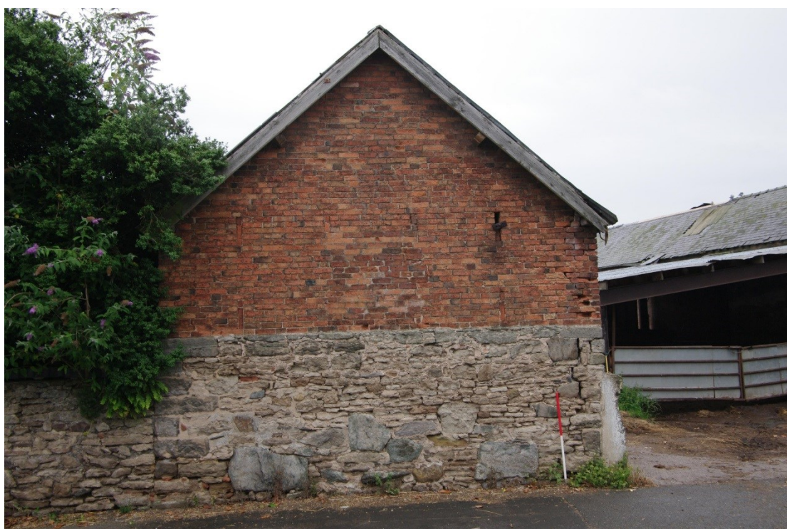
Figure 10: Barn A west facing gable end Looking east from Lady Gate. 1m scale
