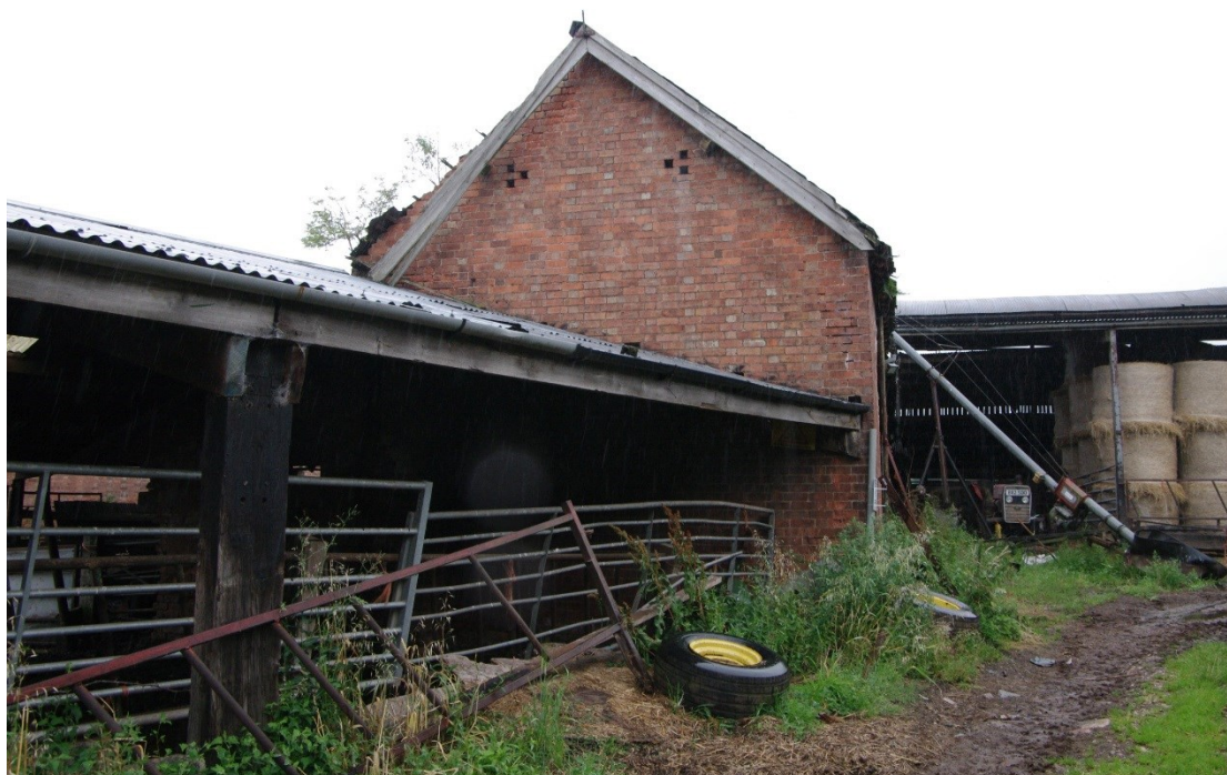
Figure 26: Barn B, west facing gable end Looking east from track down to Lady Gate
