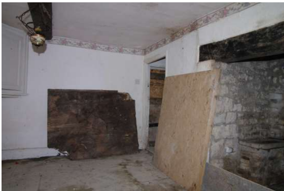
Figure 33 Ground floor Room G3 Looking north-east. Doorway to Room G4 centre right
