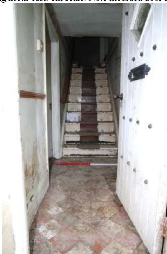
Figure 31 Room G2 hall and stairs Looking north. 1m scale. Door to G1 on left at foot of stairs
