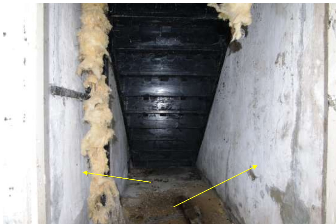
Figure 49 Space beneath stairs before stripping out of stairs and plaster Looking south. Arrows point to blocked doorways revealed after strip
