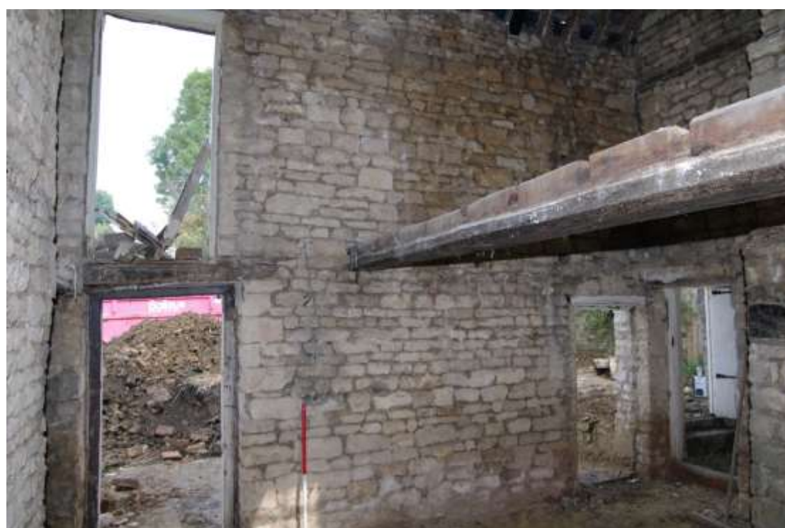
Figure 50 North wall after strip Looking north-east. 1m scale. Photo taken from approximately the foot of the stairs
