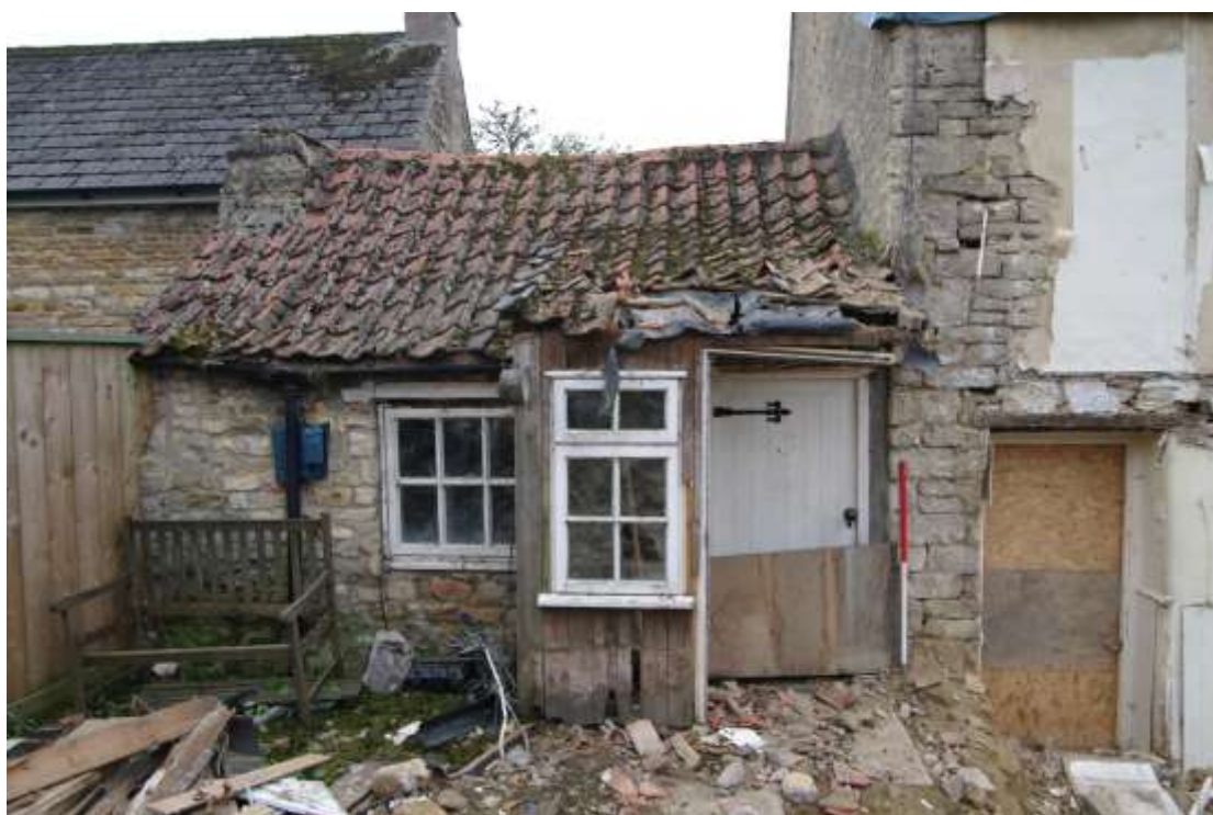
Figure 22 North-facing elevation. Single-storey extension on east of house Looking south. 1m scale
