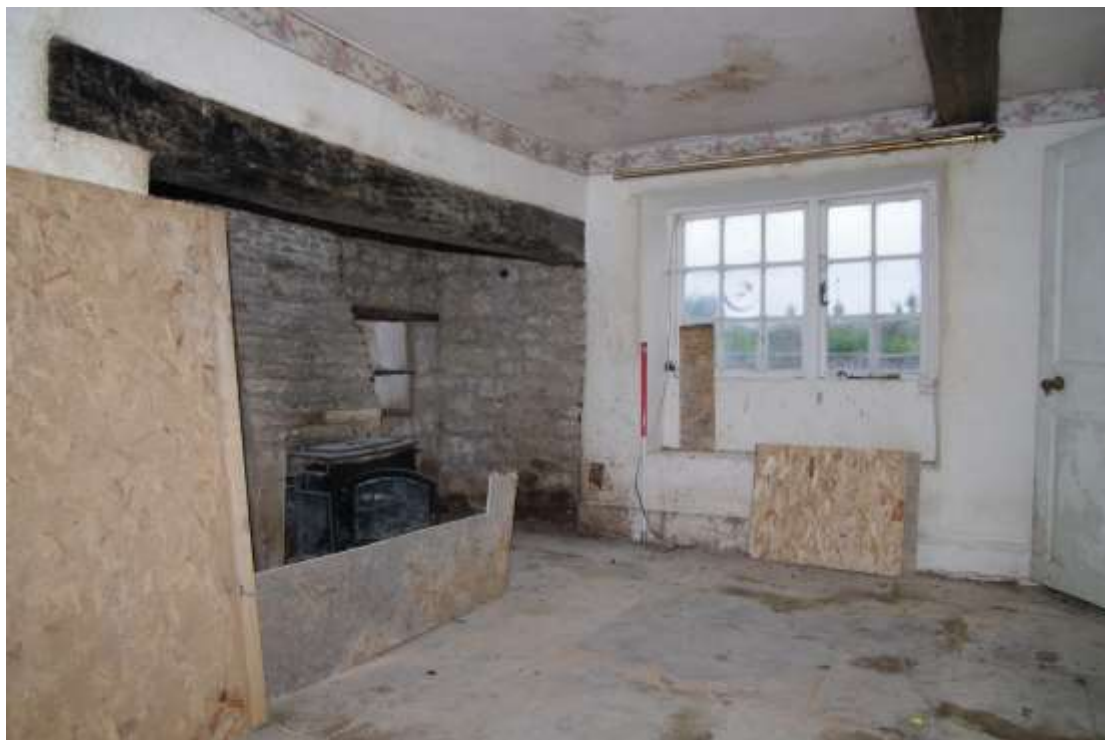
Figure 32 Ground floor Room G3 Looking south-east. 1m scale. Door to hall G2 on right
