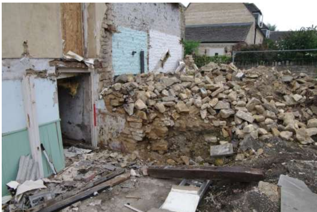
Figure 21 Former area of lean-to extension Looking north-west from former bathroom. 1m scale
