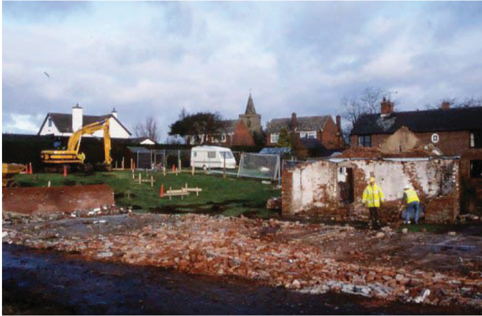
Plate 1. General shot of development site looking north west. Plot 1 being excavated, Plot 2 in foreground under bricks. Outhouses being demolished.
