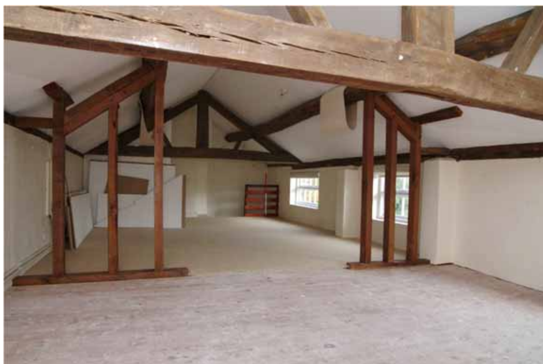
Figure 57 Second floor Looking north east. Stairs down are behind the 1m scale
