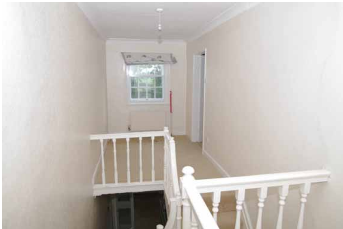
Figure 49 Room F3 landing Looking south-east. 1m scale. Doorway to F1 on right
