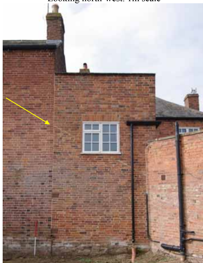
Figure 16 South-east facing elevation extension Looking north-west. 1m scale. Arrow indicates the original height of the extension and its subsequent raising
