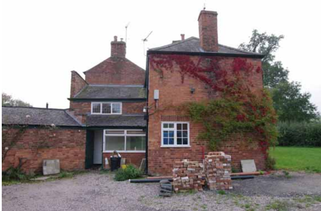
Figure 21 North-east facing elevation Looking south-west. 1m scale. Original house on left. Note parapet wall in front of lean to extension. Outbuilding on far left
