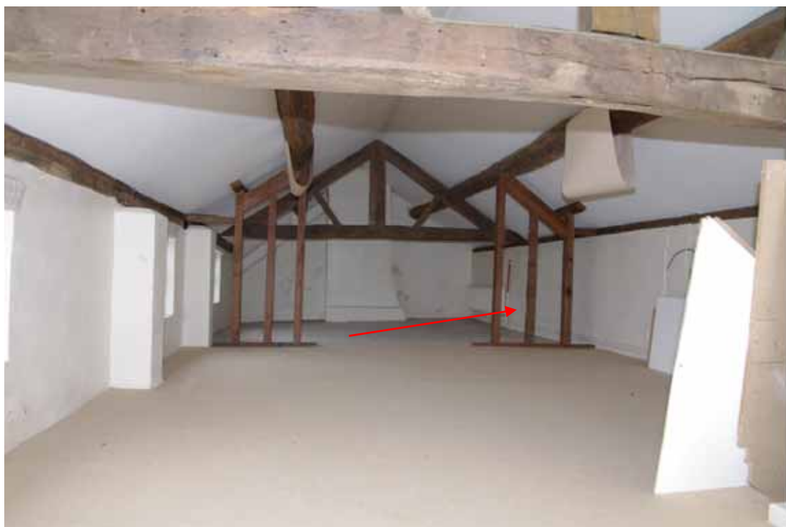
Figure 58 Second floor Looking south-west. 1m scale. Arrow marks approximate point where new stairs will enter the room.
