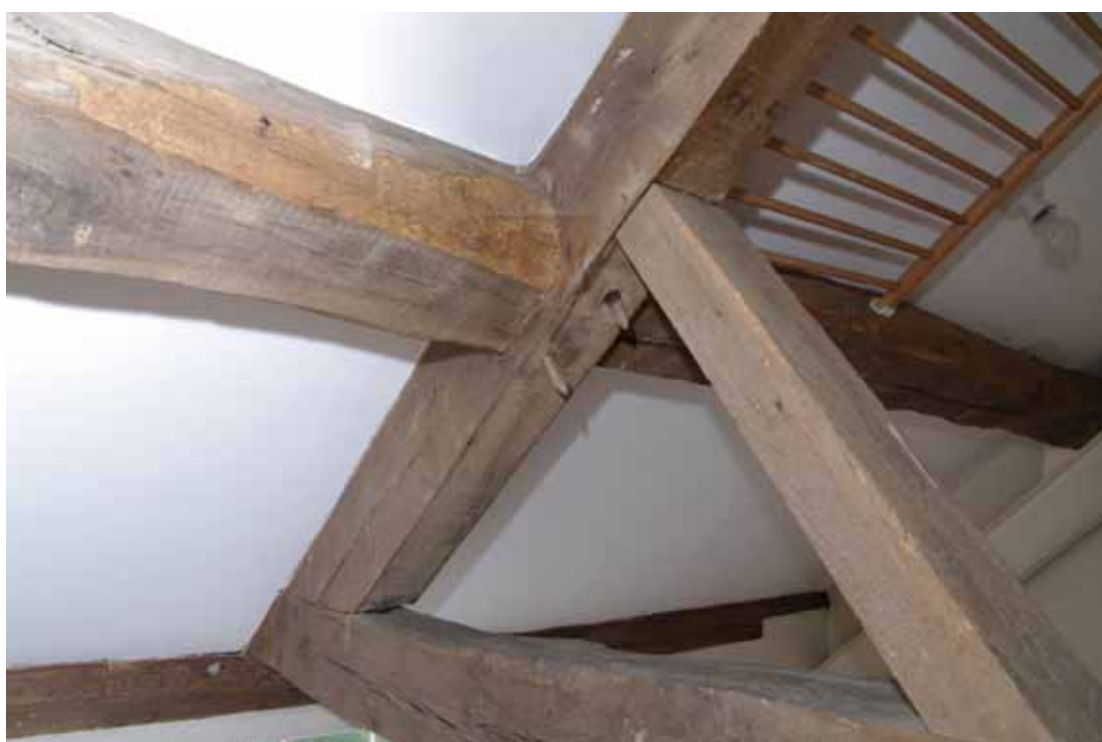
Figure 59 Second floor, detail of pegged roof timbers Southernmost truss. Note steel inserted to support the corner of the roof.
