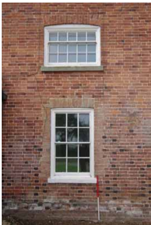
Figure 15 South-east facing elevation ground and first floor window detail Looking north-west. 1m scale
