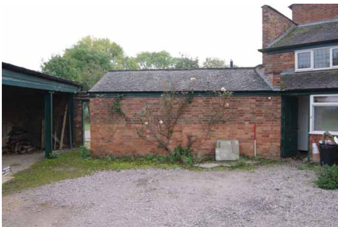
Figure 28 Outbuilding, north face Looking south. 1m scale. Note upper rebuilt/extended wall (at top of scale)
