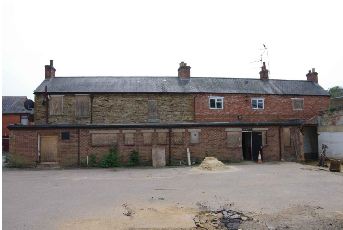
Figure 15 North facing elevation Looking south. 1m scale. 1970s extension to left of ranging pole. Demolished outbuildings on right of picture
