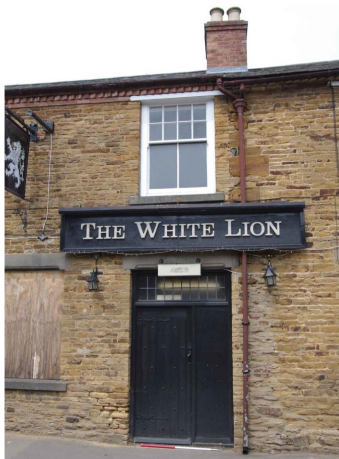
Figure 11 South facing elevation, joint between east and west portions Looking north. 1m scale
