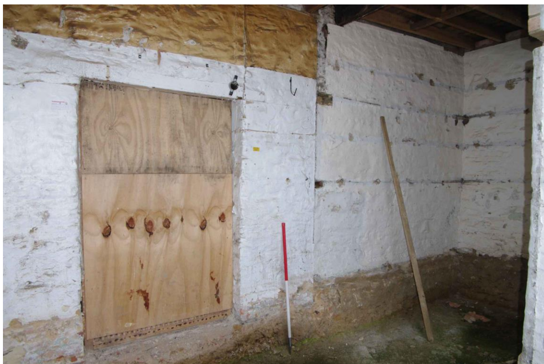
Figure 18 North facing elevation, ground floor wall at west end Looking south-west. 1m scale
