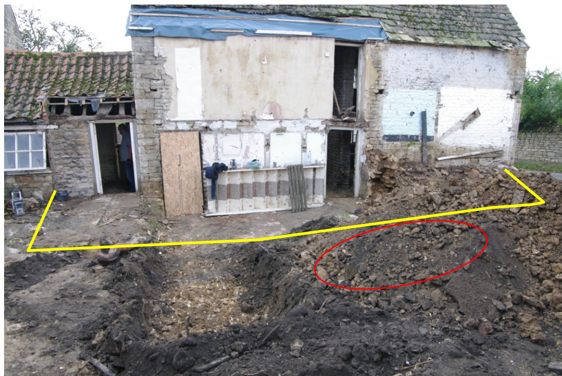
Figure 5: Proposed area of new extension Yellow line indicates approximate location of demolished extension Red circle shows area of modern service disturbance
