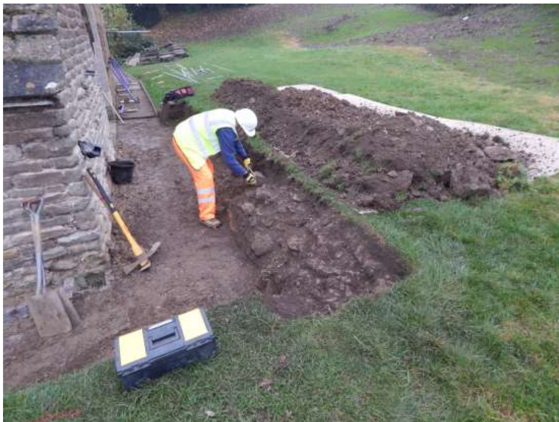
Plate 1: Work in progress on Test Pit 4, where path turns to the east, looking south-west
