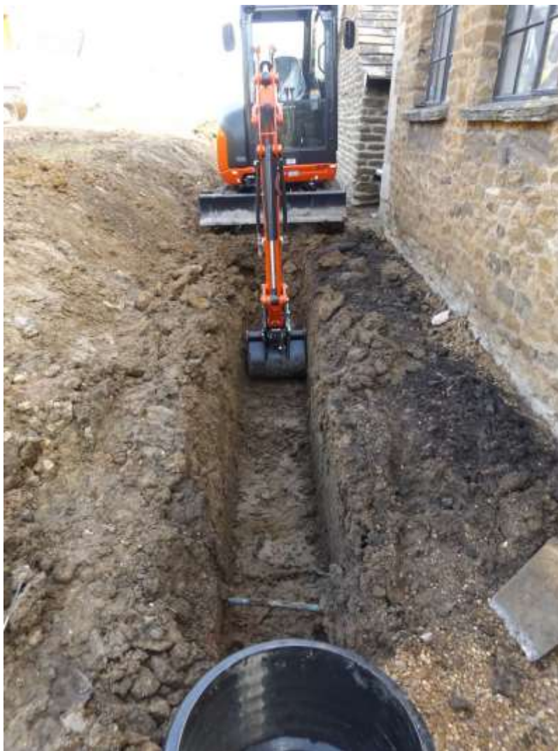
Plate 27: Work in progress on water pipe trench, west side of building, looking north
