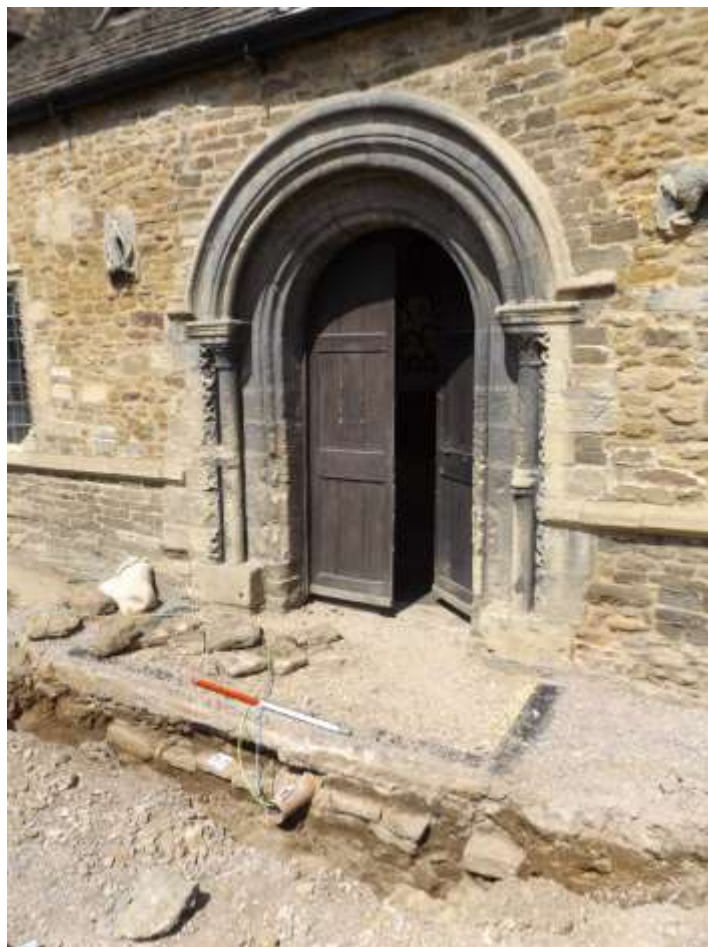
Plate 60: Stone drain found during excavation of cable trenches in front of Great Hall, looking north-west
