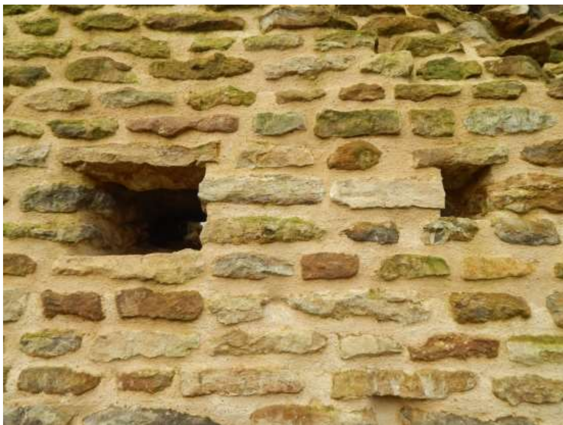
Plate 49: Close-up of putlog holes
